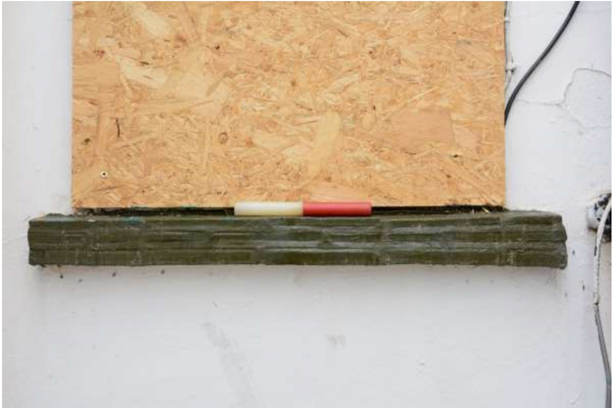
Fig.34: Sill construction at the rear/northern part of the building reiterating that seen at the front (0.2m scale)
