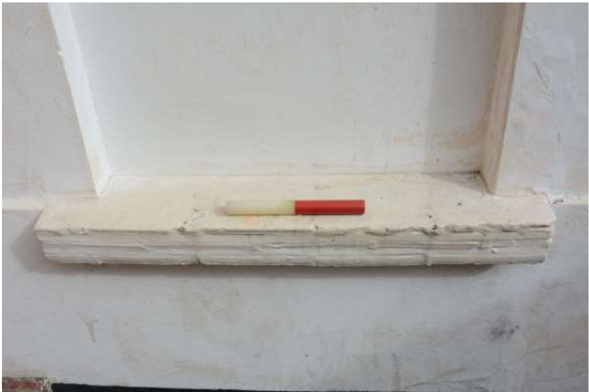
Fig.33: The same sill construction seen on the blocked lower section of the window to the right of the secondary front entrance
