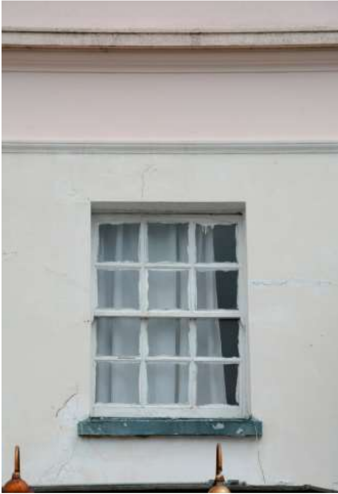
Fig.39: The southernmost sash window on the building frontage, with stone sill below
