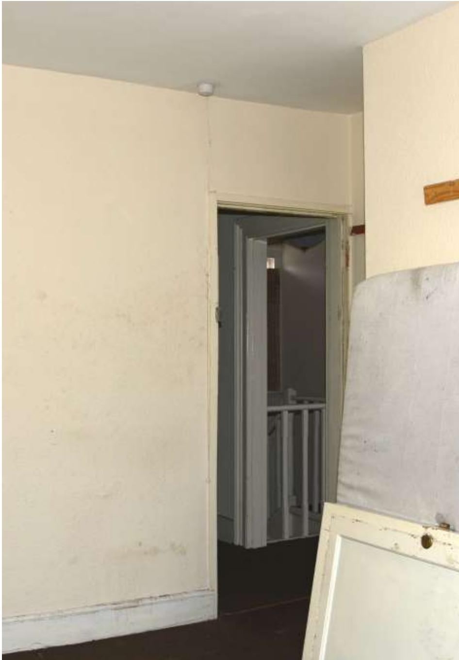
Fig.107: The northwestern bedroom, looking back towards the landing. The doorframe appears quite modern – much simpler than elsewhere – and was presumably cut through when the small central room was created
