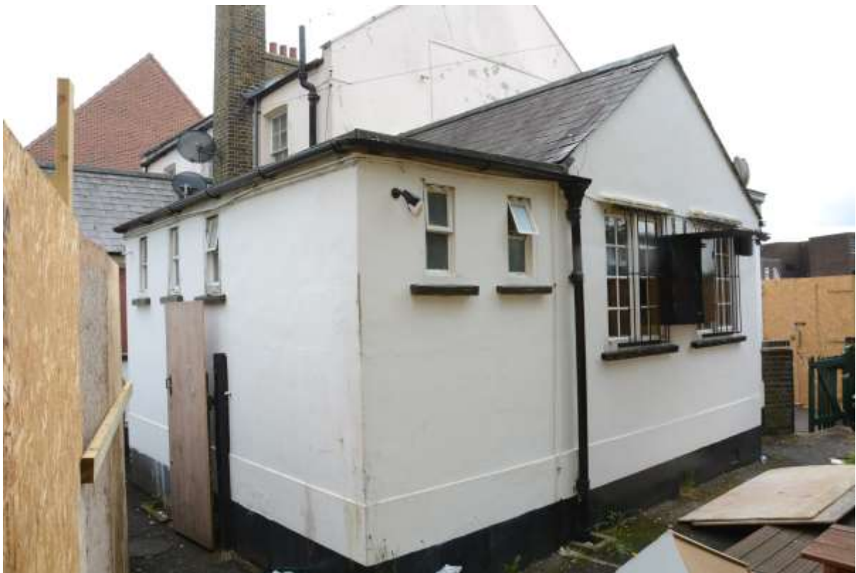
Fig.17: The northwestern extensions to the property, view looking south. The toilet block to the left is probably an addition to the main pitched-roof central block, the junction discernible in the external rendering
