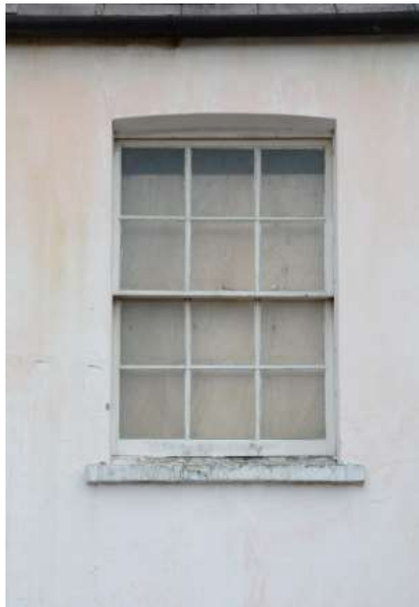
Fig.40: The southernmost window at the rear of the building, similar to that above but slightly rounded headed
