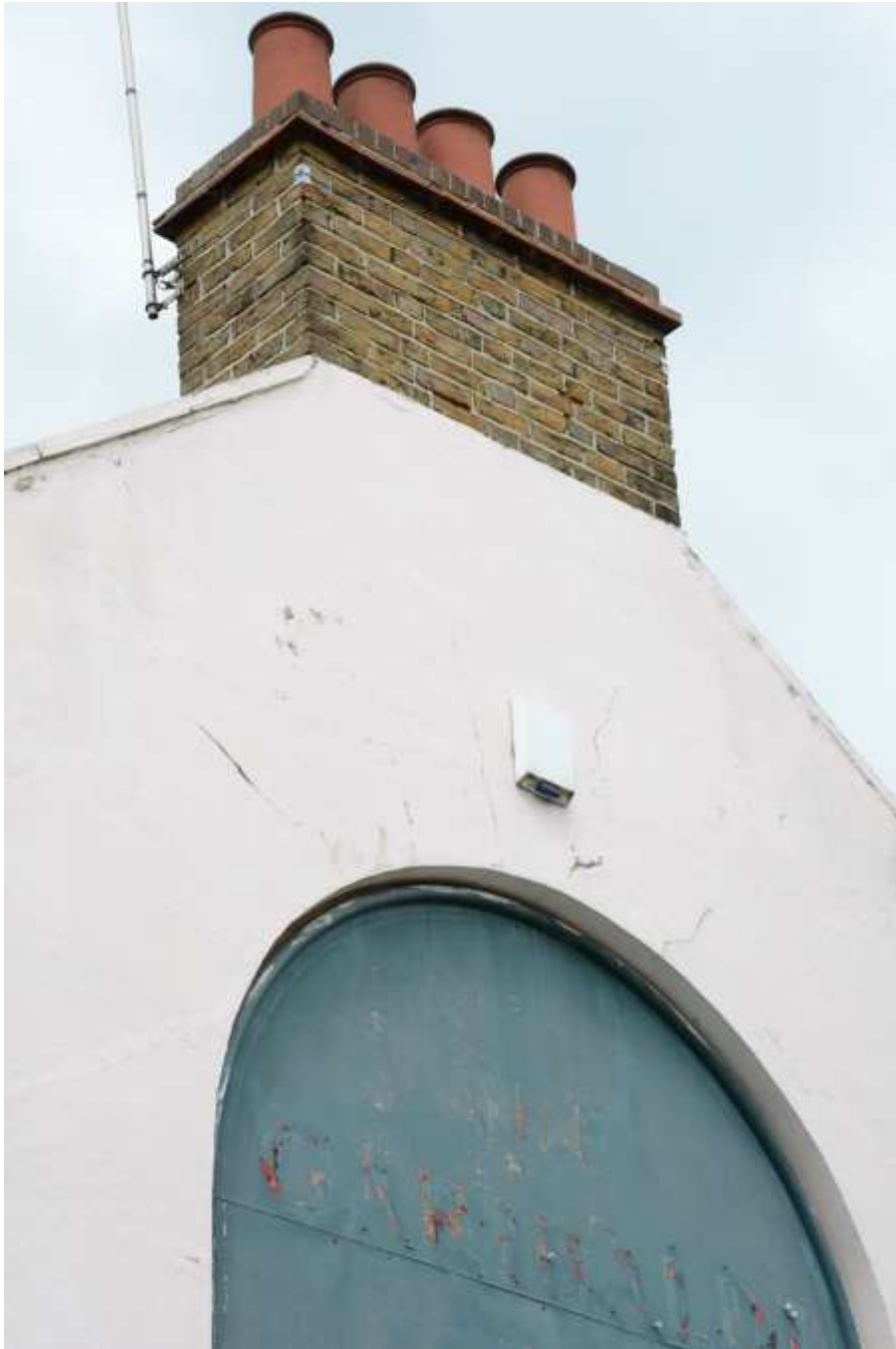
Fig.43: Detail of the southeastern gable end and projecting chimney breasts. At the northwestern end these are flush with the wall, but the front chimney here was smaller (cf. Fig.113; also reflected in three rather than four pots)
