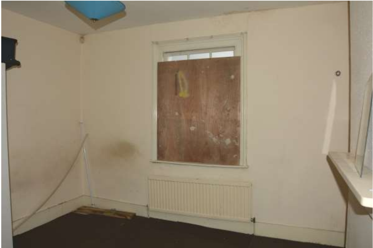
Fig.99: The boarded up back bedroom window (see Fig.40 for exterior view)
