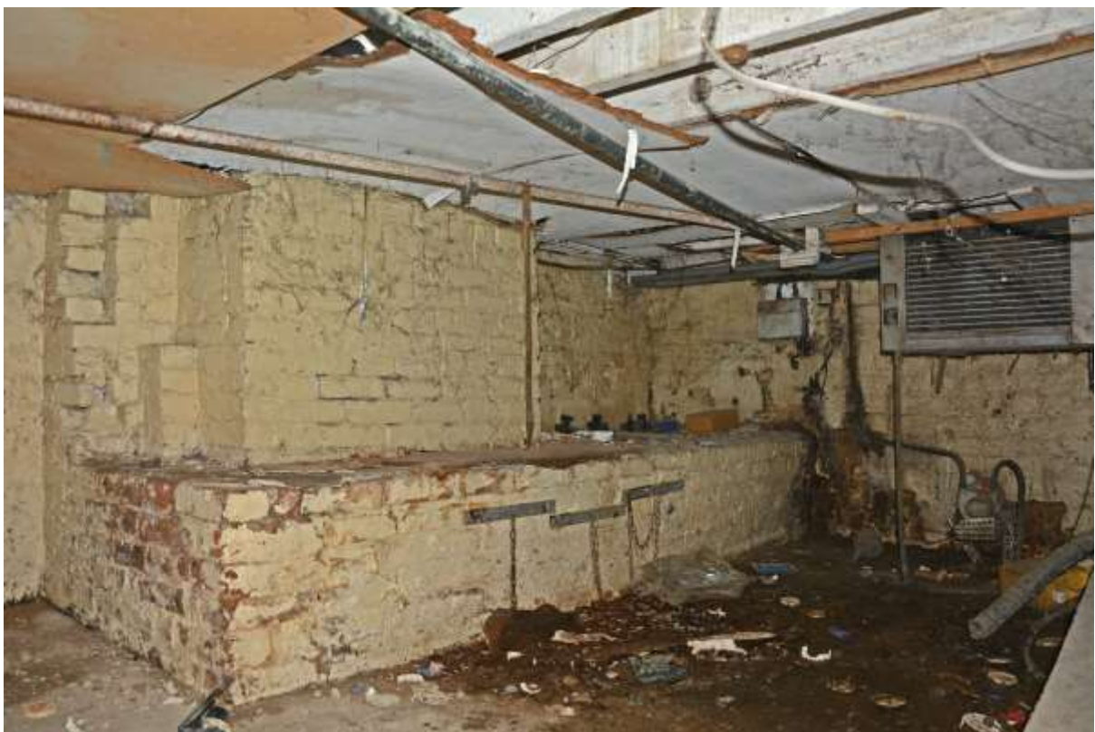
Fig.49: View of the substantial brick base below the rear (northernmost) chimney stack. To the left of the frame this has evidently undergone some modification, although the reasons for this are not clear. There is no such base towards the front of the building to support the chimney stack there, but this appears to be a less substantial structure (see also Fig.115)
