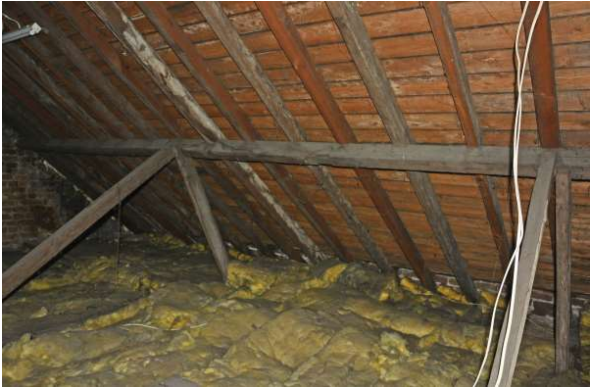
Fig.113: The southwest side of the roof space, highlighting the double strut arrangement here, and also a cut-out on the purlin for what may have been a further intermediate support
