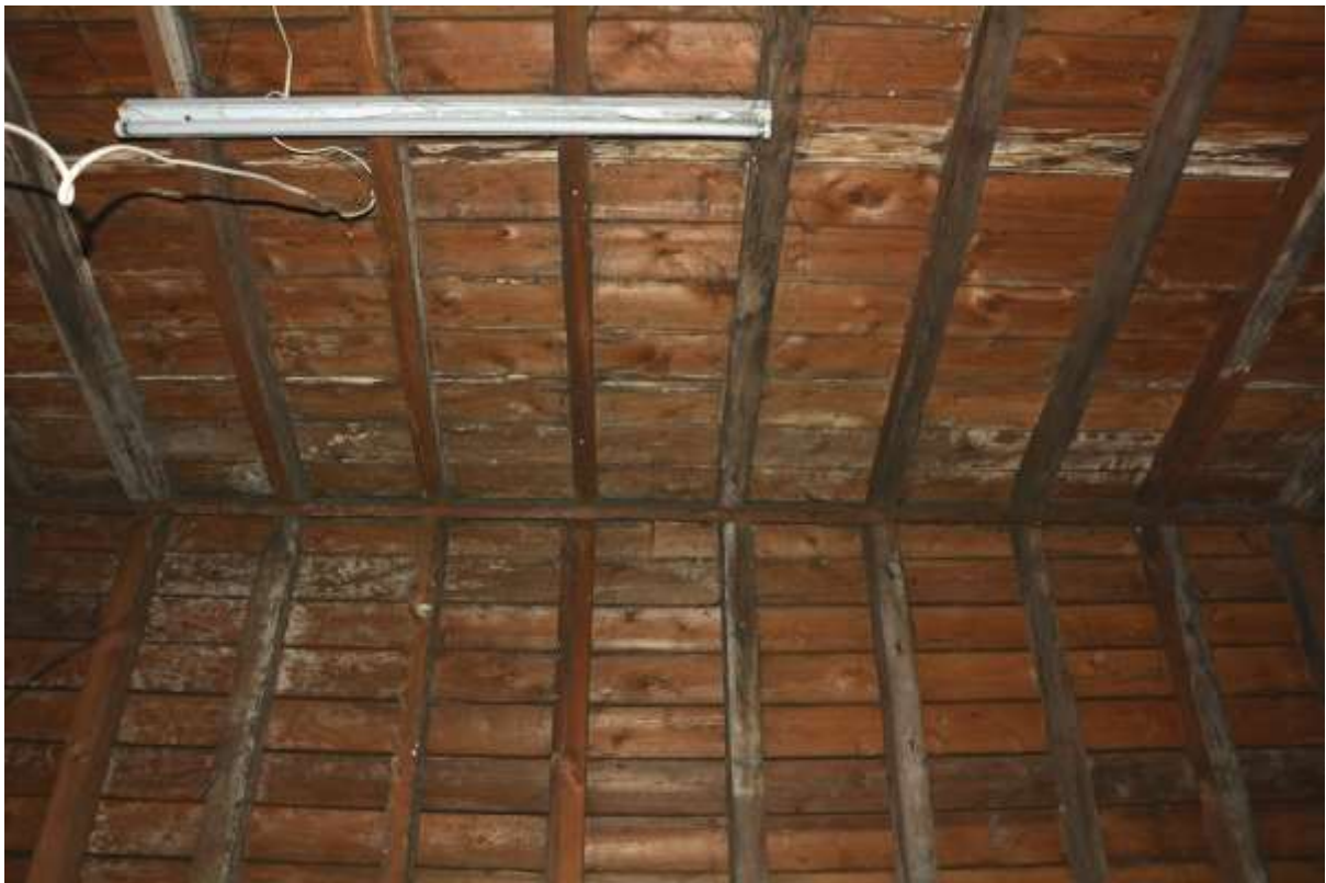
Fig.116: View looking directly up to the ridge board, towards the NW end of the roof
