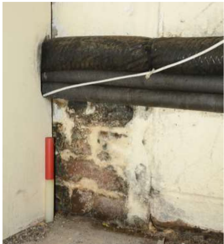
Fig.83: Close-up of the junction between the storeroom breeze-block extension and to the left the original eastern corner of the main building (0.2m scale)
