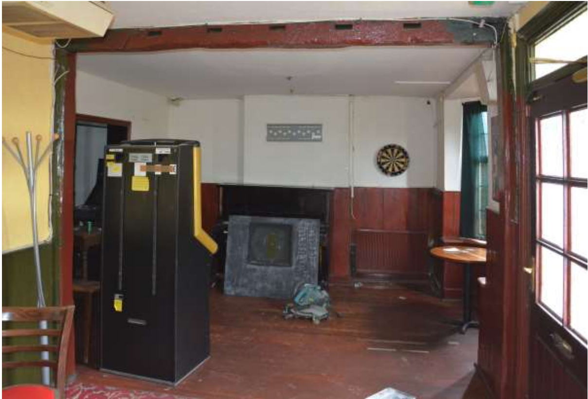
Fig.56: The southeastern end of the bar. It is not clear whether the ceiling beam in the foreground (with mortice holes on this side only) is original, though it is assumed to follow the line of an original division
