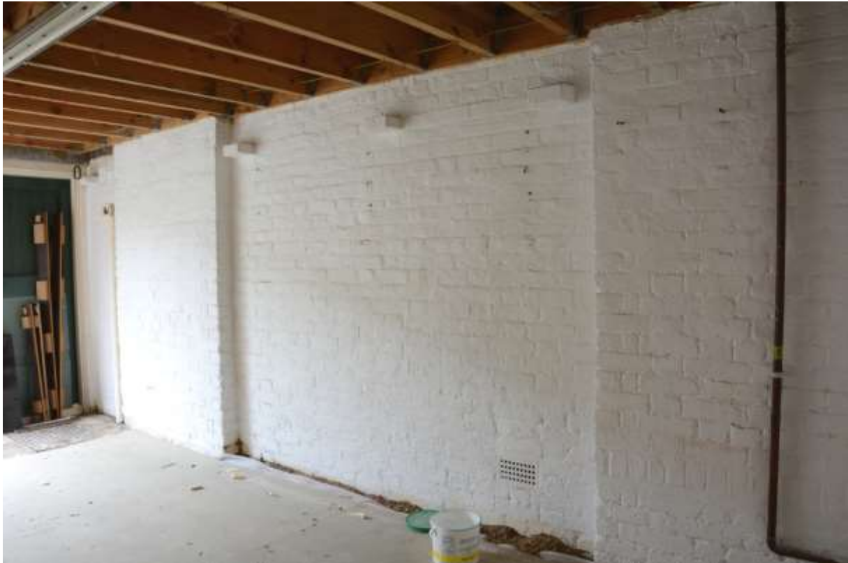
Fig.75: The SE wall of the main building, with projecting chimney breasts and five corbels for an earlier roof (two beyond the further chimney breast; see Fig.76). The wall itself is not rendered, which may reflect the original building design – see above (5.3) for further discussion
