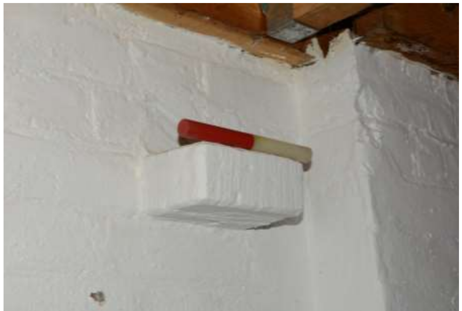
Fig.78: Close-up of corbel on the main wall, adjacent to the NE chimney stack. The brick coursing around (& particularly above) the corbels was slightly disturbed, suggesting that they been set into the wall after construction
