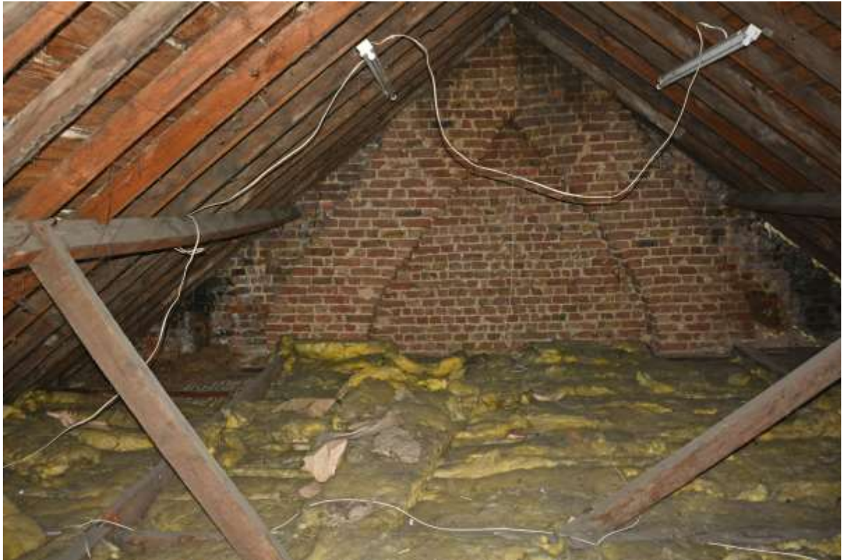
Fig.111: Looking towards the southeastern end of the roof and illustrating the differing angle of support struts for the purlins on either side. The chimney breasts are also visible in the gable end, narrower than those on the external face of the wall (cf. Fig.43)
