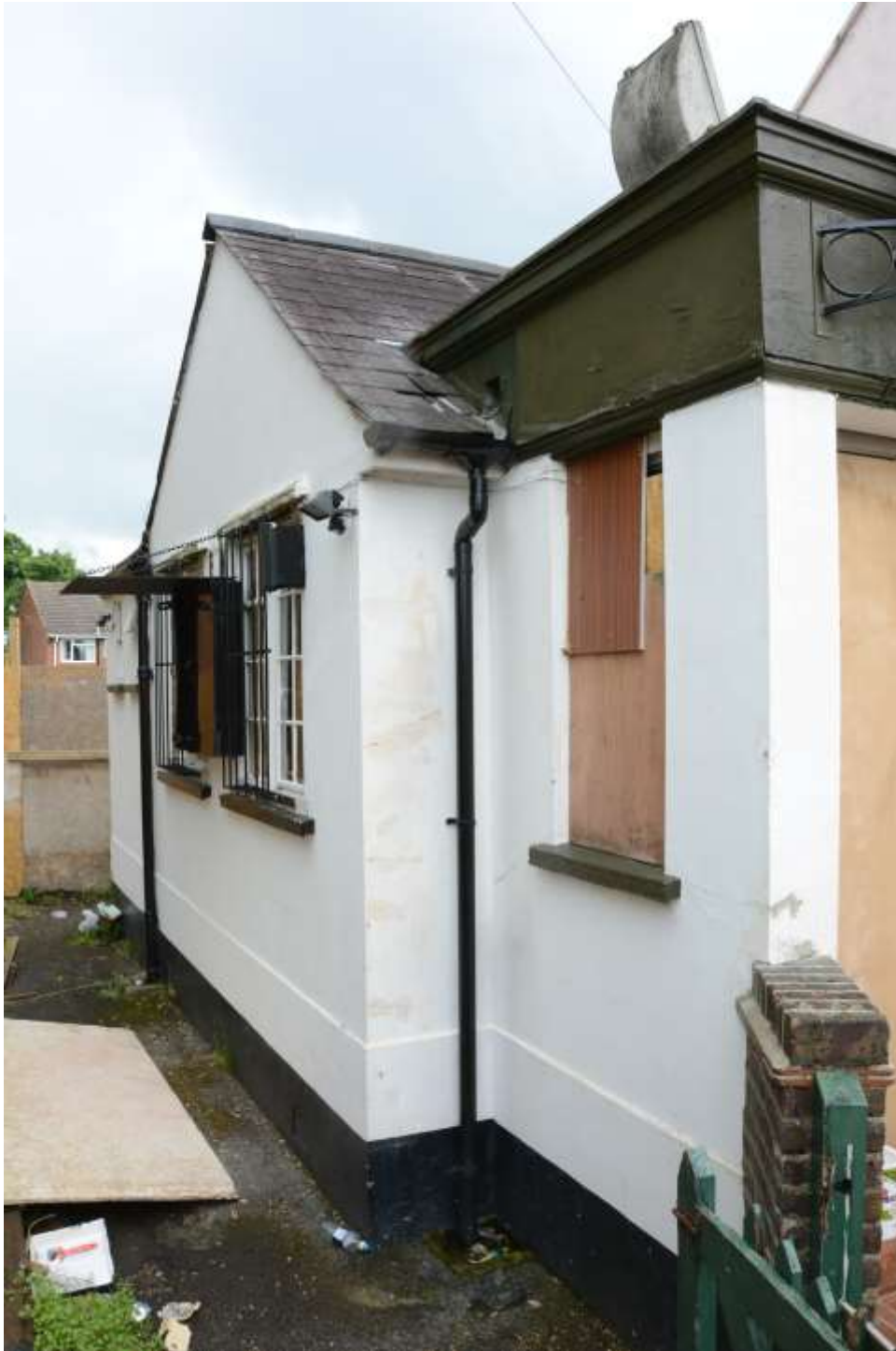
Fig.26: The northwestern end of the property, showing what are probably two phases of extension – the central block with its pitched roof and the flat-roofed entrance lobby in the foreground
