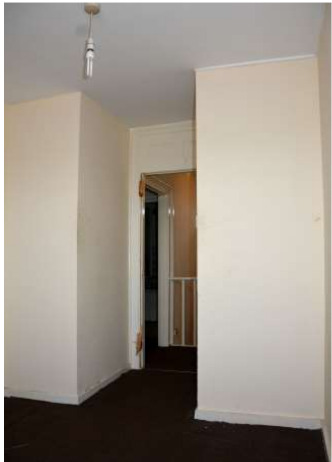
Fig.104: View of central front room looking back towards the landing, the side walls cut in to maintain access to the adjacent rooms
