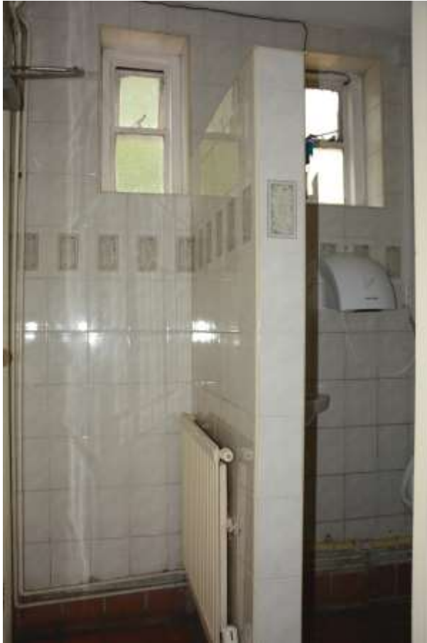
Fig.67: The interior of the men's toilets at the northern corner of the building
