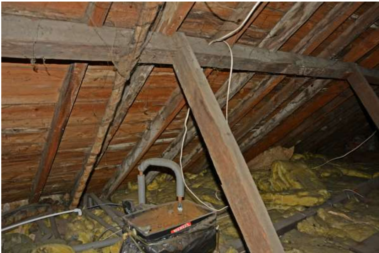
Fig.114: The northeast side of the roof space, detail of purlin and single supporting strut
