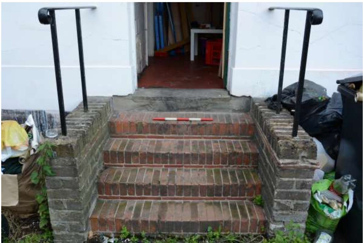
Fig.31: Steps to the main rear (kitchen/scullery) entrance, almost certainly contemporary with those above
