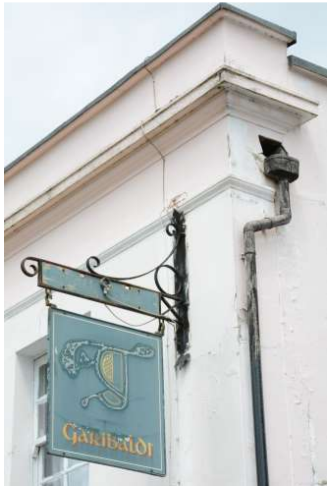
Fig.42: The southeastern end of the parapet, actual roof level clearly indicated by the downpipe
