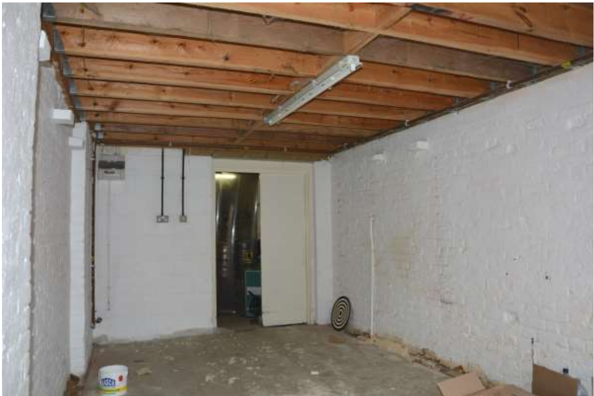
Fig74: A similar view to the above, the main building (& three corbels) once again to the left of the frame
