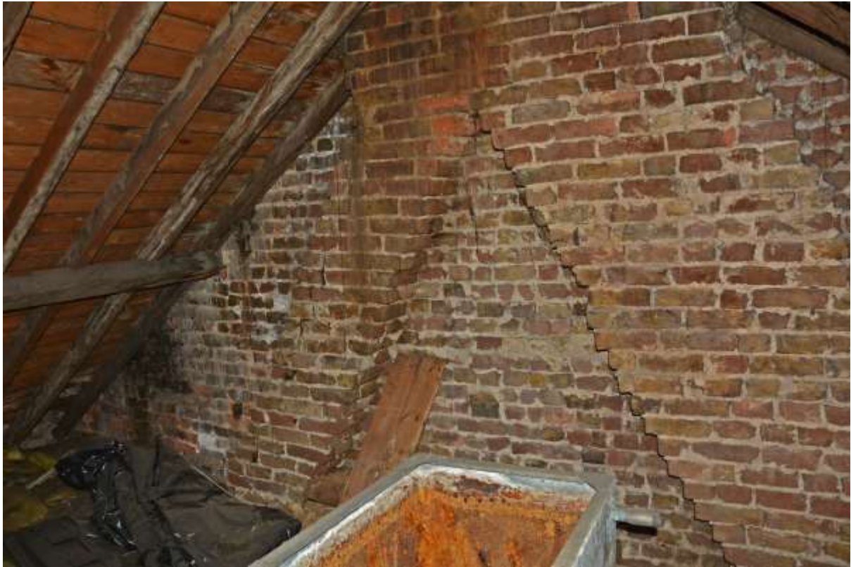
Fig.115: Interior of the northwest gable end and showing the chimney breasts, which are not visible on the exterior wall. The breast in the foreground (& at the rear of the building) is approximately twice the width of that to the SW
