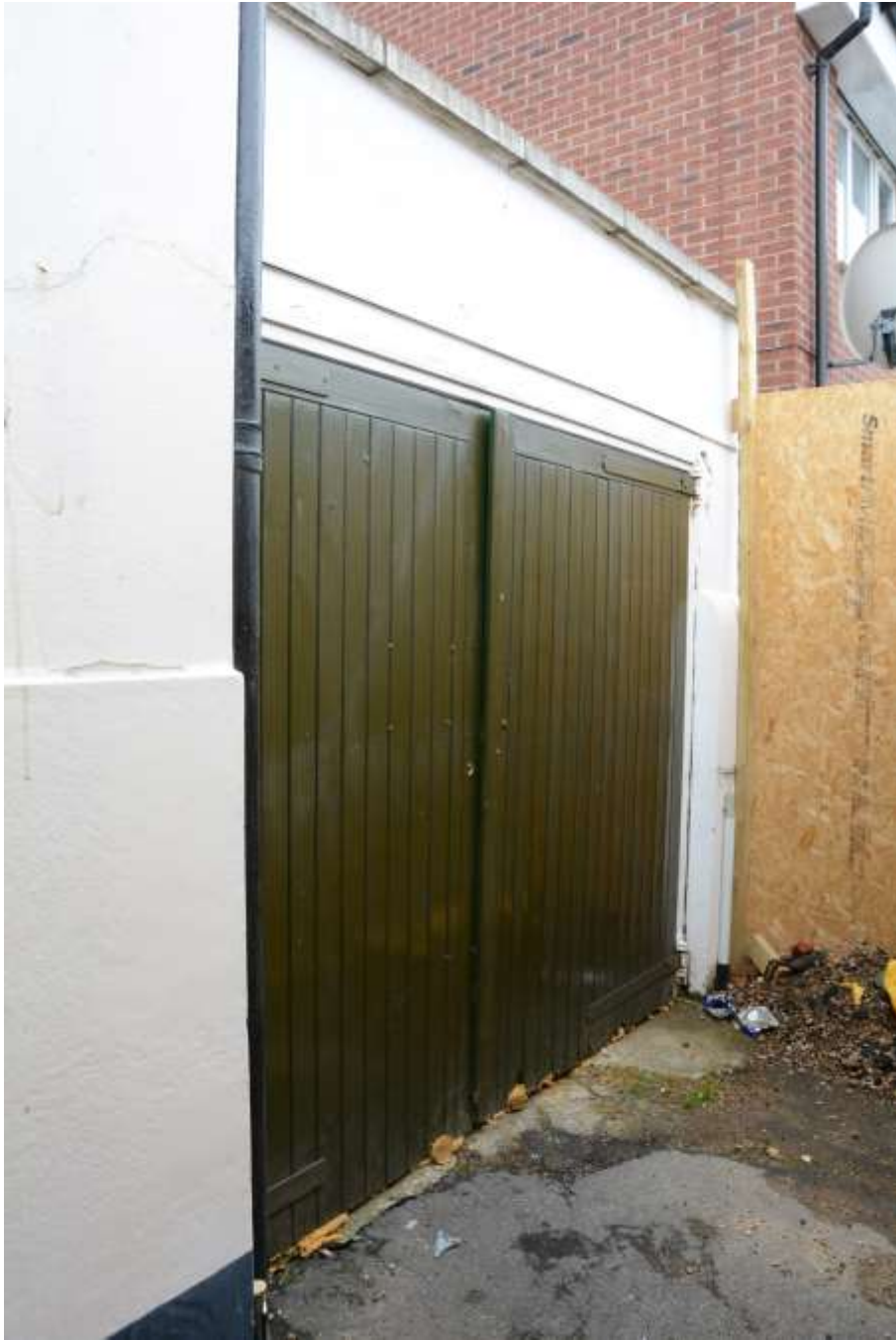
Fig.37: Modern double garage doors at the southern end of the building frontage
