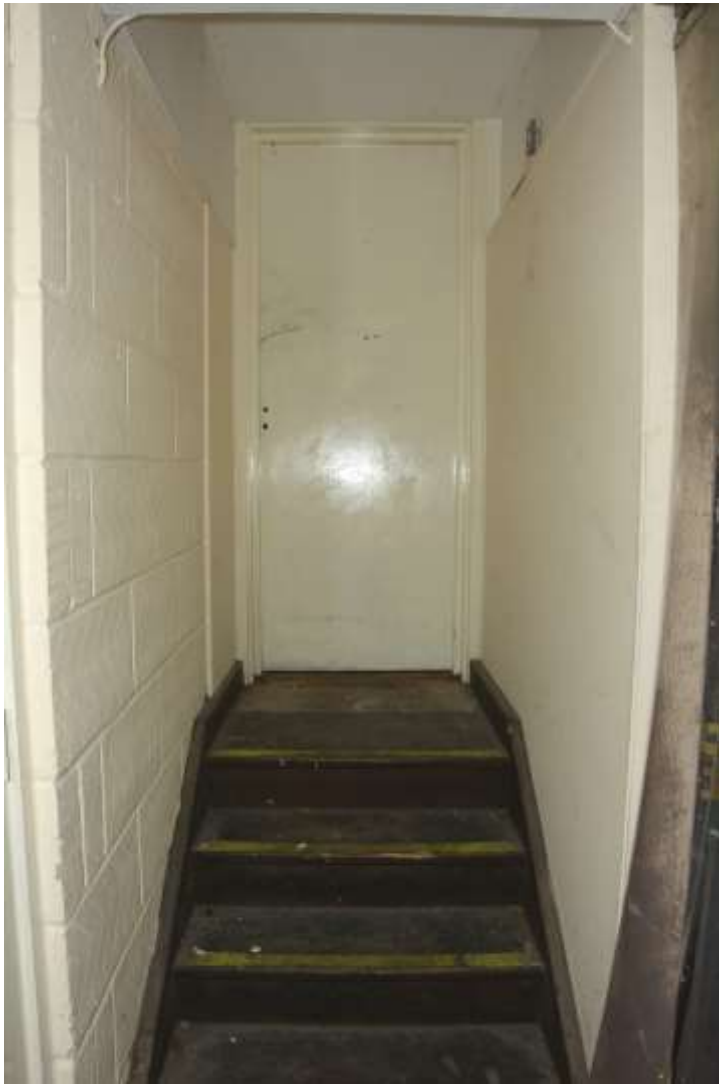
Fig.82: Stairs and doorway into the main building (see Fig.60 for the other side)
