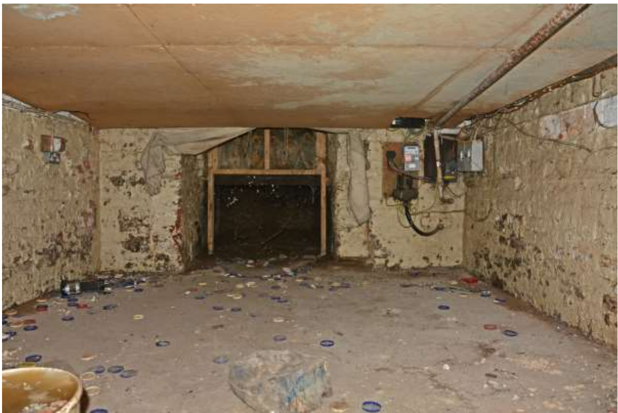
Fig.47: The main cellar, looking towards the external access hatch at the front of the building. The headroom is very low, approximately 1.4m to the base of the overlying joists
