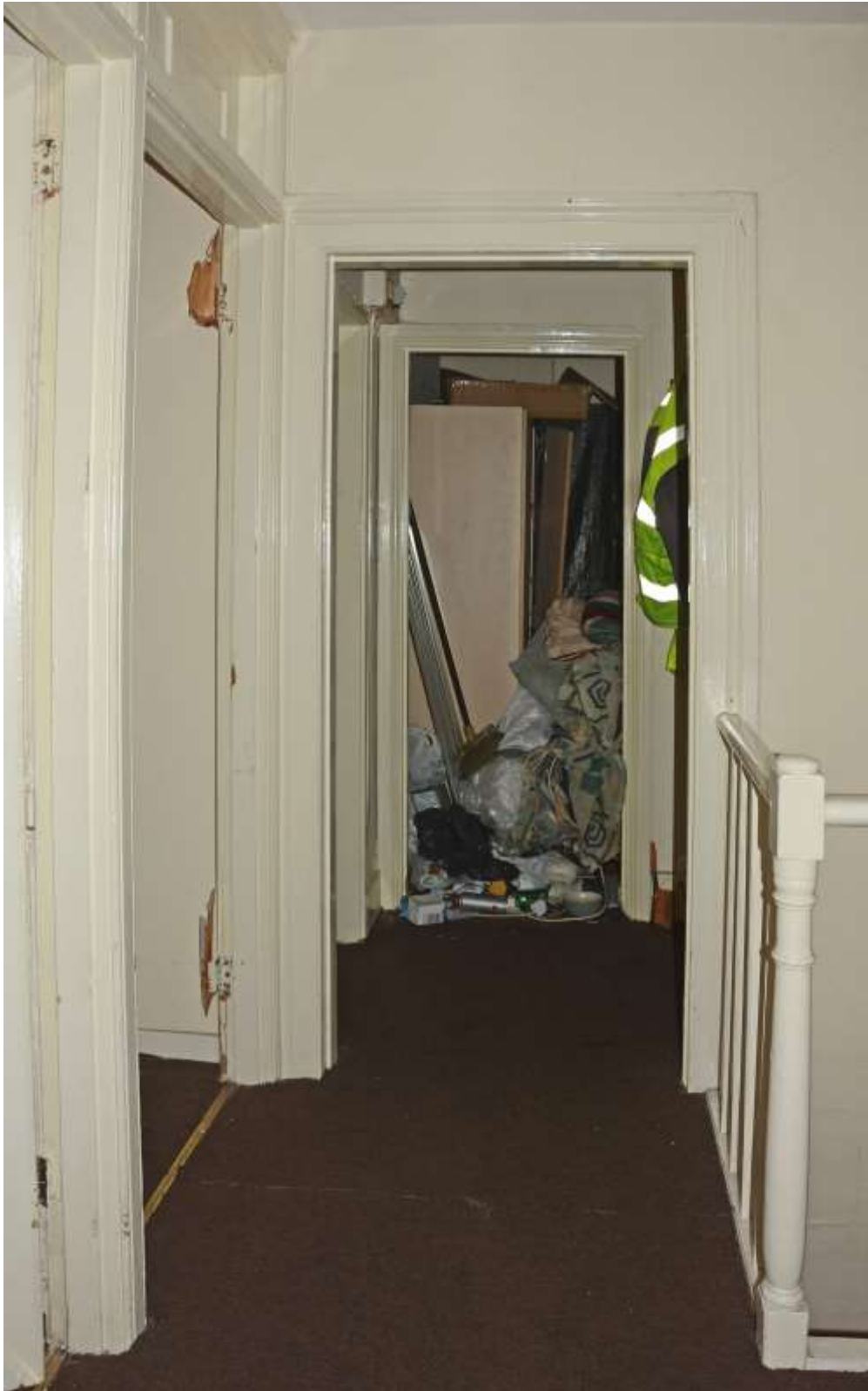
Fig.96: The landing looking NW. Three different styles of joinery are visible around the doors in this picture: probable original moulding in the left foreground and at the end of the balustrade, framing around the cupboard to the rear as part of a later (?earlier 20 th century) subdivision, and just visible between these the apparently modern frame of the northwestern bedroom door
