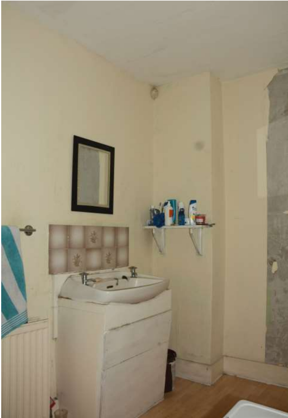
Fig.110: The bathroom, looking toward the NW corner and one side of the chimney breast. It is likely that this room and the part of the adjacent landing and cupboard were formed out of one larger original bedroom, with a fireplace on the northwest wall
