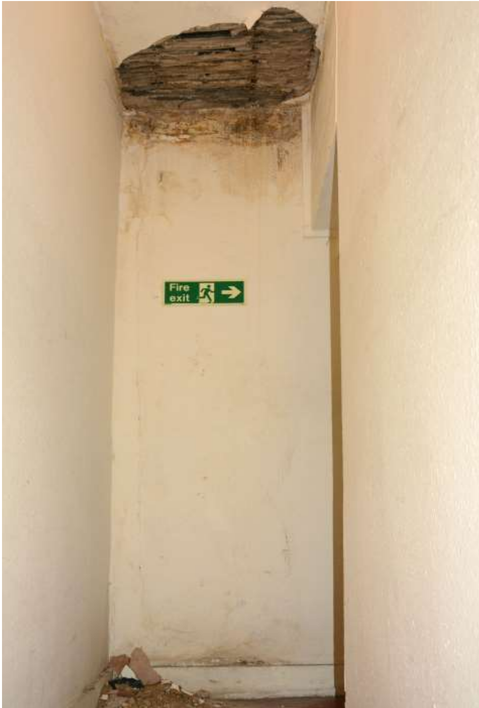
Fig.88: The passageway leading to the stairs and first floor. At the northeastern end an area of ceiling plaster has broken away, exposing the underlying lath-and-plaster construction
