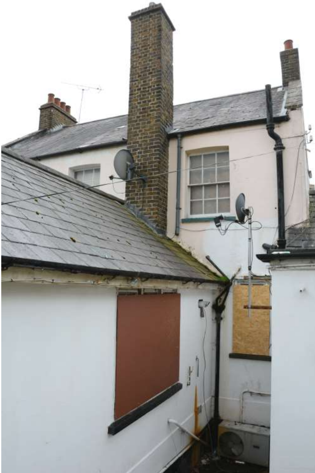
Fig.29: The rear of the building with extensions to its original northern corner, looking SSW
