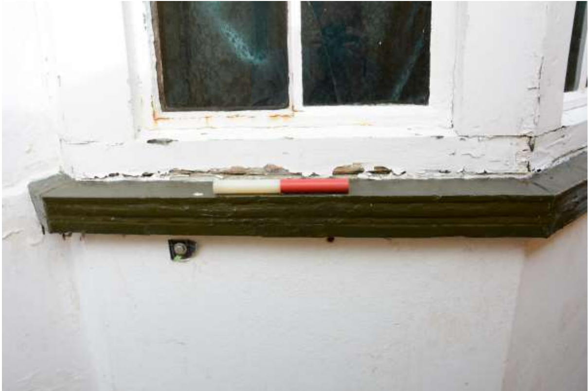
Fig.32: Detail of the front/ northwestern bay window sill, showing the layered tile construction (0.2m scale)
