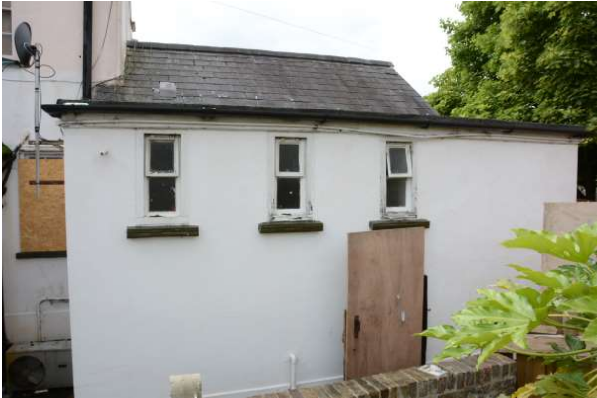
Fig.28: The back (NW) wall of the rear toilet block, almost certainly a secondary extension to the single storey pitched roof structure in the background
