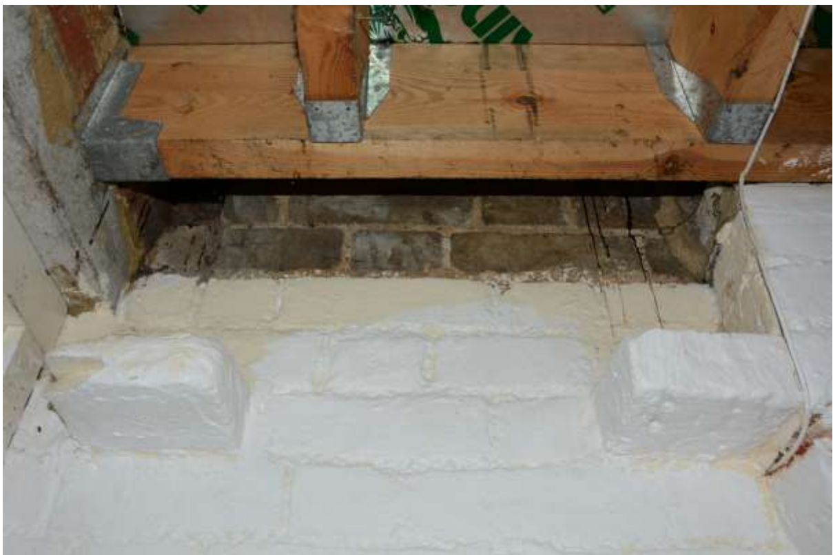
Fig.76: Detail of the two corbels at the SW end of the main building wall. This also shows that the wall (at least in this area) was originally bare brick, neither painted nor rendered
