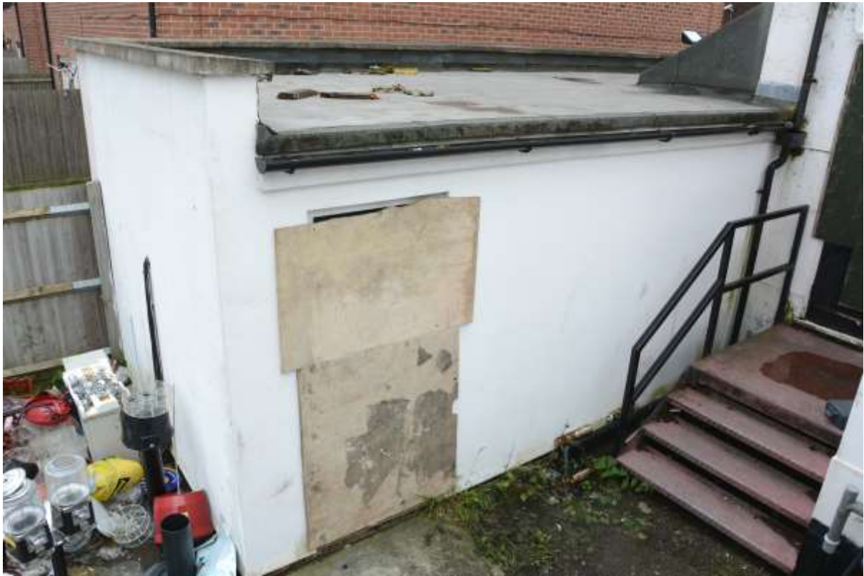
Fig.36: The modern breeze-block built single storey extension at the eastern corner of the building. The fairly recent metal-framed steps to the right give access to the principal rooms, and suggest that the doorway here is also quite modern
