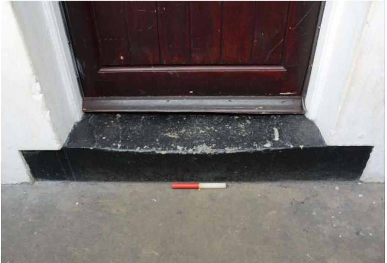
Fig.24: Close-up view of the worn front entrance step (0.2m scale). Both ends are slightly recessed, indicating that the adjacent rendering is later – see also Figs 79 & 83 below
