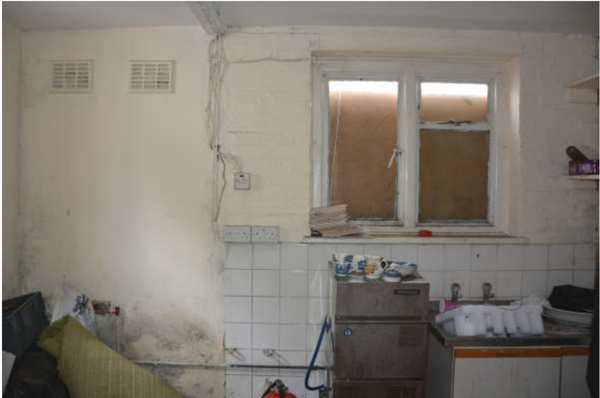
Fig.86: The smaller utility room/scullery behind the main kitchen. Only at the NW end and extending c 1.2m is the brickwork rendered (as shown to the left of the frame: the ventilators here indicate that this was originally a separate larder
