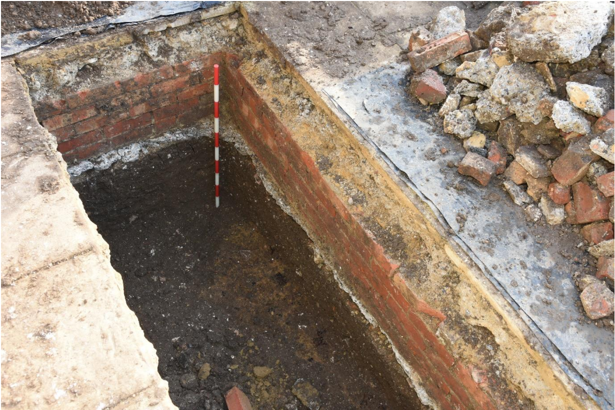
Figure 13: Trench 1 eastern end. Brick wall [102] with the underlying made ground deposit (104) and the surfaces of (105) and (106 at the trench base. Looking south-east, scale 1m.
