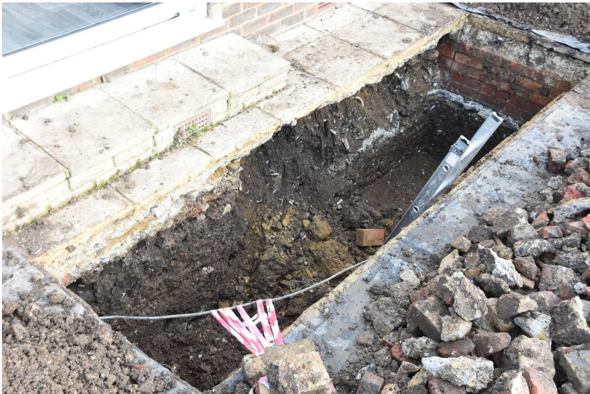
Figure 12: Trench 1 after further section collapse, looking north-east. No scale.
