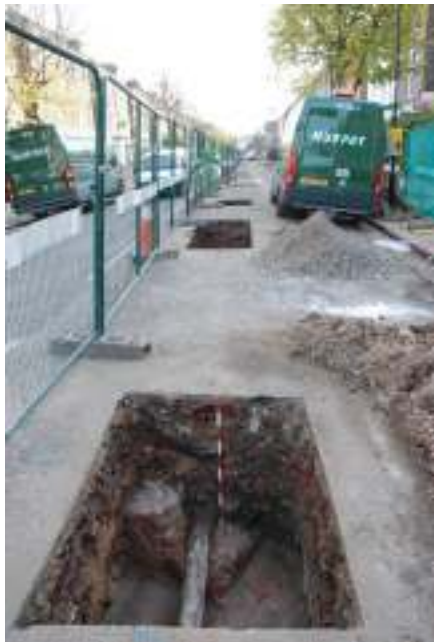
Figure 9: General view looking south down Wilberforce Road from Test Pit 3, showing the nature of water main replacement works on Wilberforce Road. Test Pits 1 and 2 are located to the north of this point. In the next test pits visible, 4 and 5 by the front wheels of the Murphy's van, a stratified sequence of probably natural alluvial clays was recorded (Figures 10 and 11).
