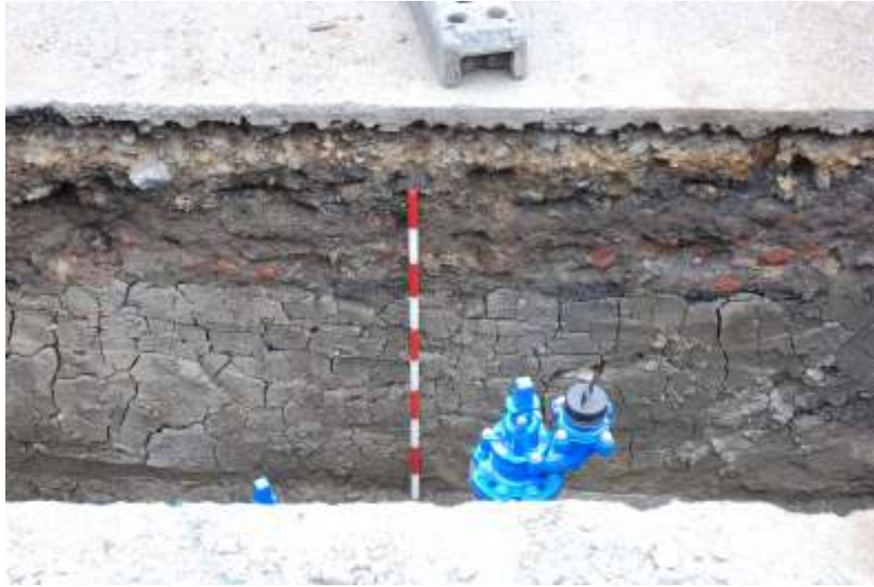
Figure 43: Pit at the Wyatt Road and Riversdale Road junction showing modern road layers overlying alluvial deposits.
