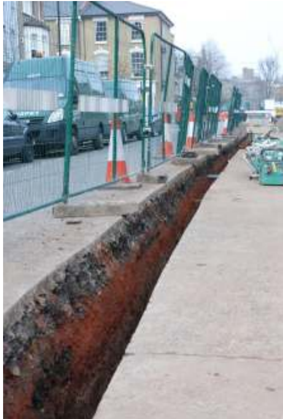
Figure 40: Trenching on Somerfield Road, showing evidence of the red brick made ground layer, which formed a base for the late 19 th century road.
