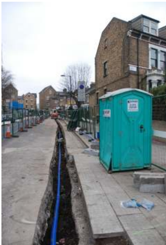
Figure 28: General view of Trench 2 looking approximately west from the junction with Queen's Drive.
