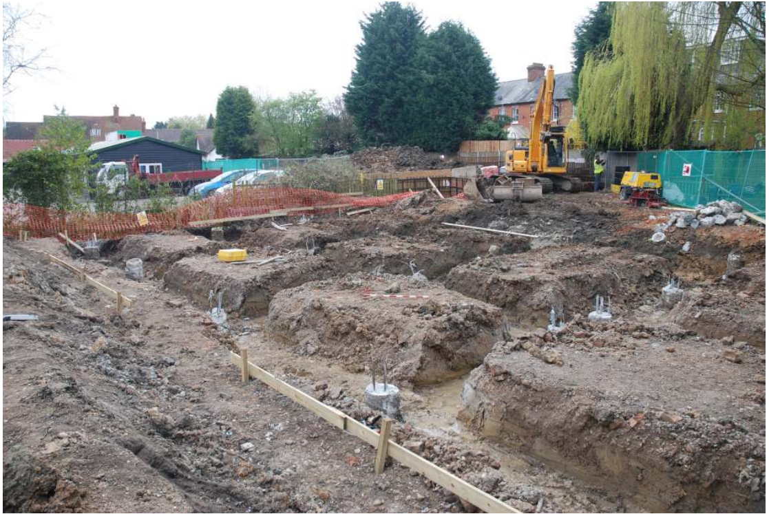
Figure 4 General view of the footprint of the new houses, looking south (scale 1m).
