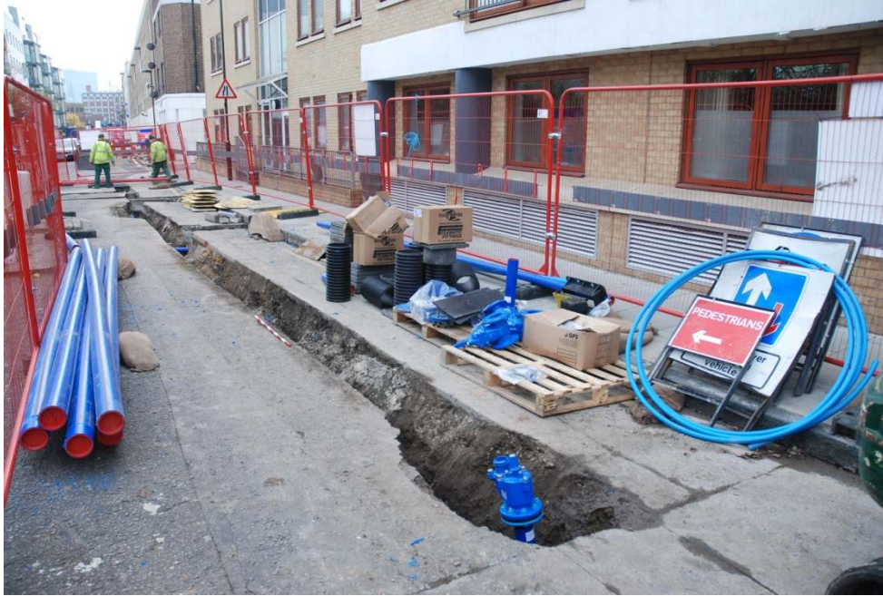
Figure 12: Trenching on Graham Street, looking north to the junction with Coombs Street (1m scale).
