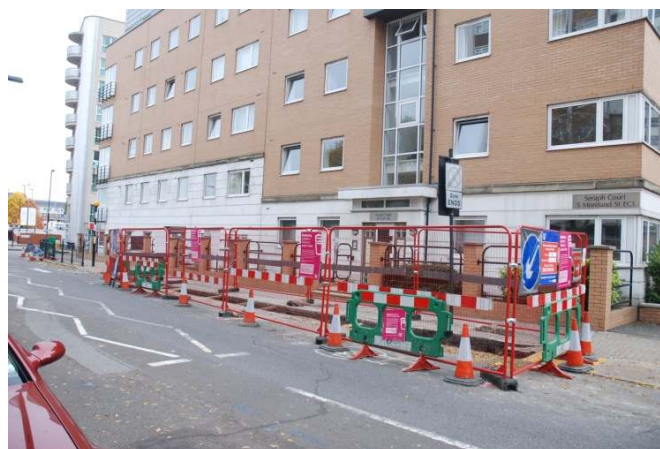
Figure 15: General view of trenching on Moreland Street looking northeast towards the junction with Central Street.
