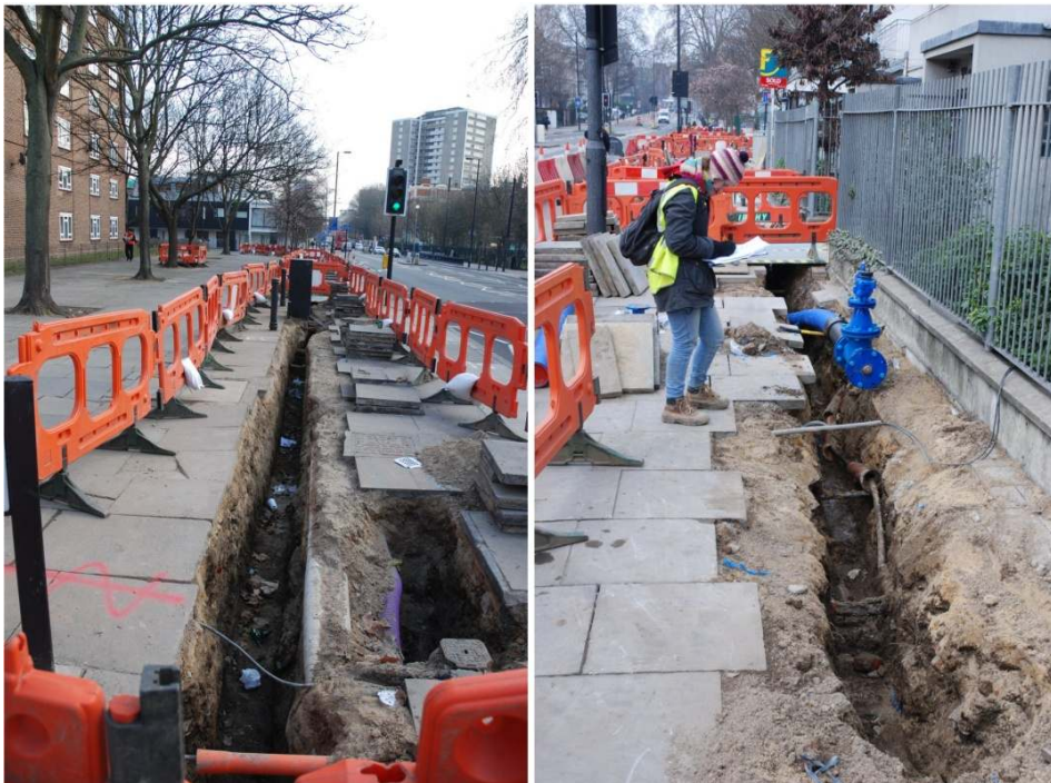
Figure 10: Trenching on City Road, to the east of Nelson Terrace (left) and to the east of Haverstock Street (right), showing modern road and paving over service deposits.
