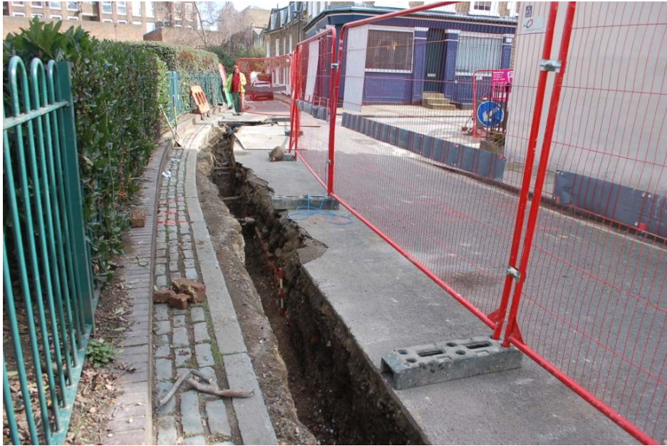
Figure 18: Trenching to the west of Remington Street on Nelson Place, showing section of brick wall in the north facing section (0.5m scale).
