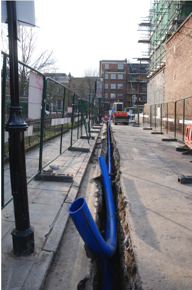
Figure 20: Trenching on Nelson Terrace looking south to the junction with City Road.
