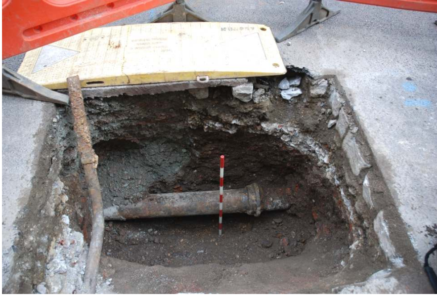
Figure 9: Trenching on the east side of City Garden Row c.35m north of the City Road junction, showing cut and backfill of the Victorian water main (1m scale).
