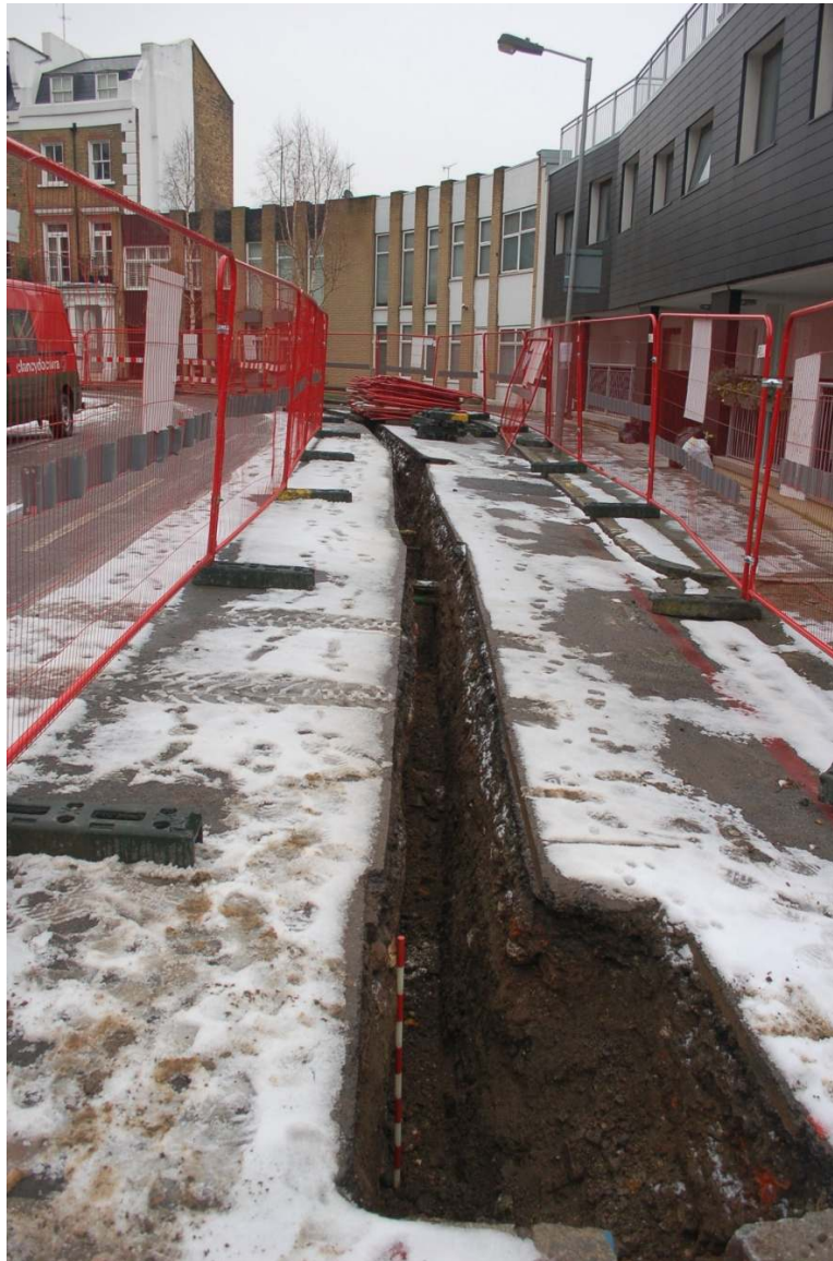
Figure 21: Trenching on Oakley Crescent looking north from the junction with City Road (1m scale).
