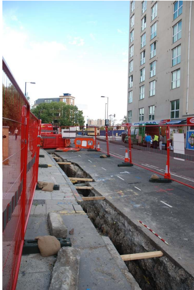
Figure 4: General view of trenching on Central Street, looking north to the junction with Moreland Street (1m scale).
