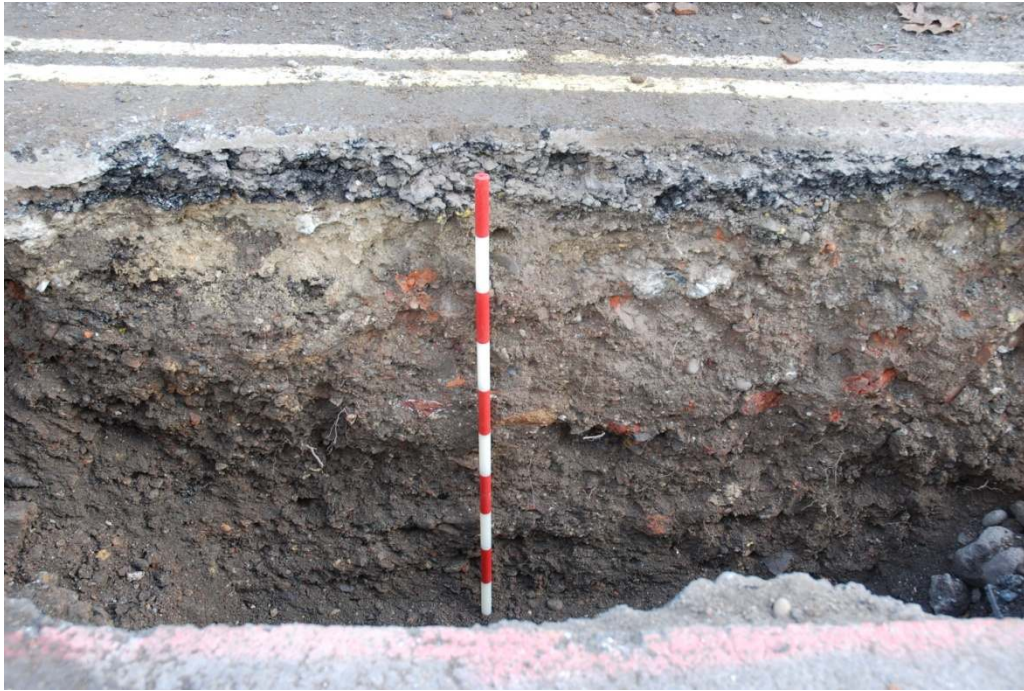
Figure 7: West facing section of trenching on City Garden Row immediately south of the Rocliffe Street junction, showing 19 th century buried made-ground deposits overlain by modern made-ground and road layers (1m scale).
