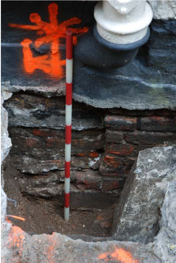
Fig. 3: Photo of the eastern section of trial pit 1, clearly showing the two different wall foundations.
