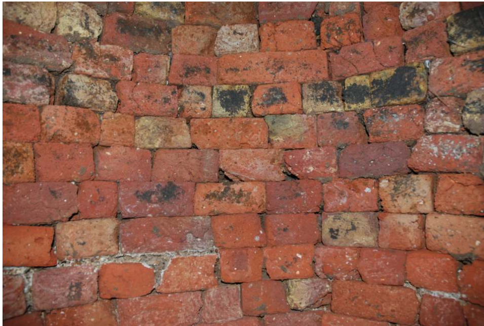
Fig. 6: Photo of the interior of the well in trial pit 1, clearly showing its brick-lined structure.
