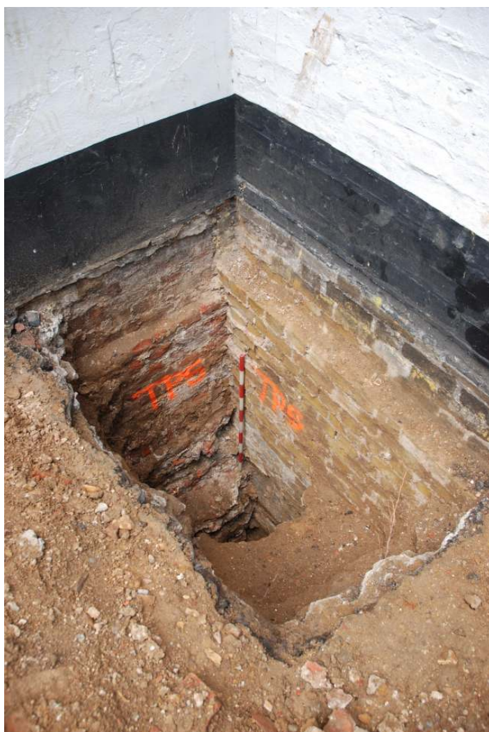
Fig. 16: Photo of trial pit 5, from the south-east, showing the contrasting red brick & rubble and yellow stock wall bases.
