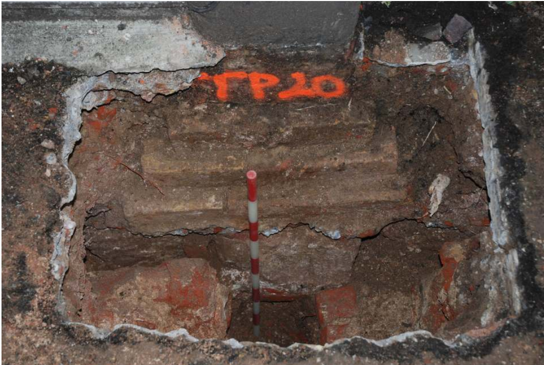
Fig. 59: Photo of trial pit 20, clearly showing the pier base and stone / mortar / brick base beneath this.
