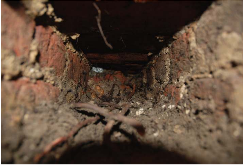
Fig. 32: Photo of interior of the brick drain in trial pit 10A, looking northwest. The drain appears to be blocked approximately 1m along this section.
