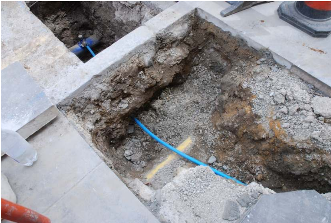
Figure 4: Trenching on Parnell Road showing modern service deposits [1] from which a wig curler was recovered.
