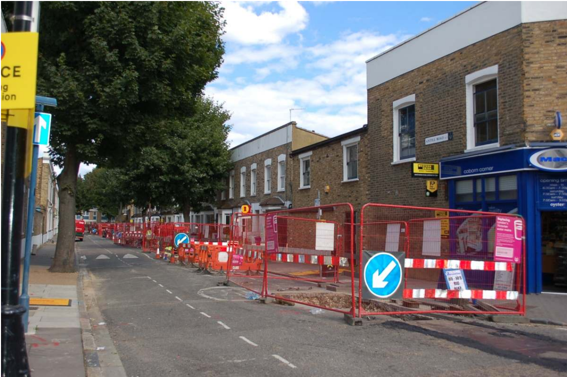
Figure 17: Trenching on Antill Road looking east from the junction with Coborn Road.
