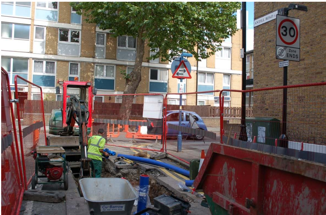
Figure 18: General view of trenching on Antill Road at the junction with St Stephen's Road.
