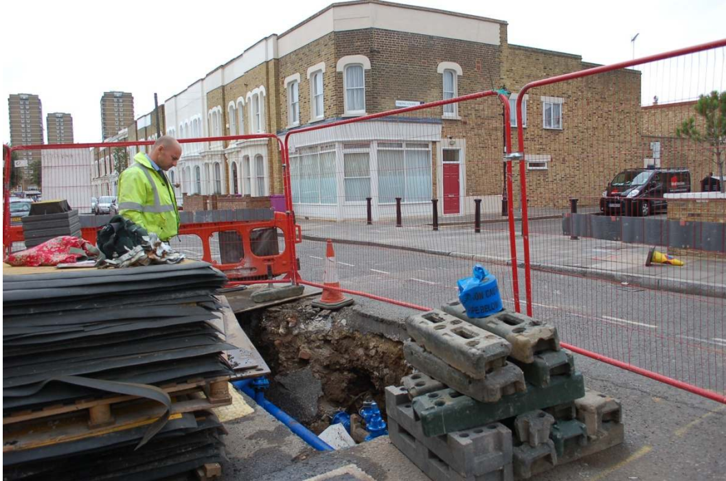
Figure 16: Trenching on Lyal Road at the junction with Viking Close, formerly Stanfield Road.
