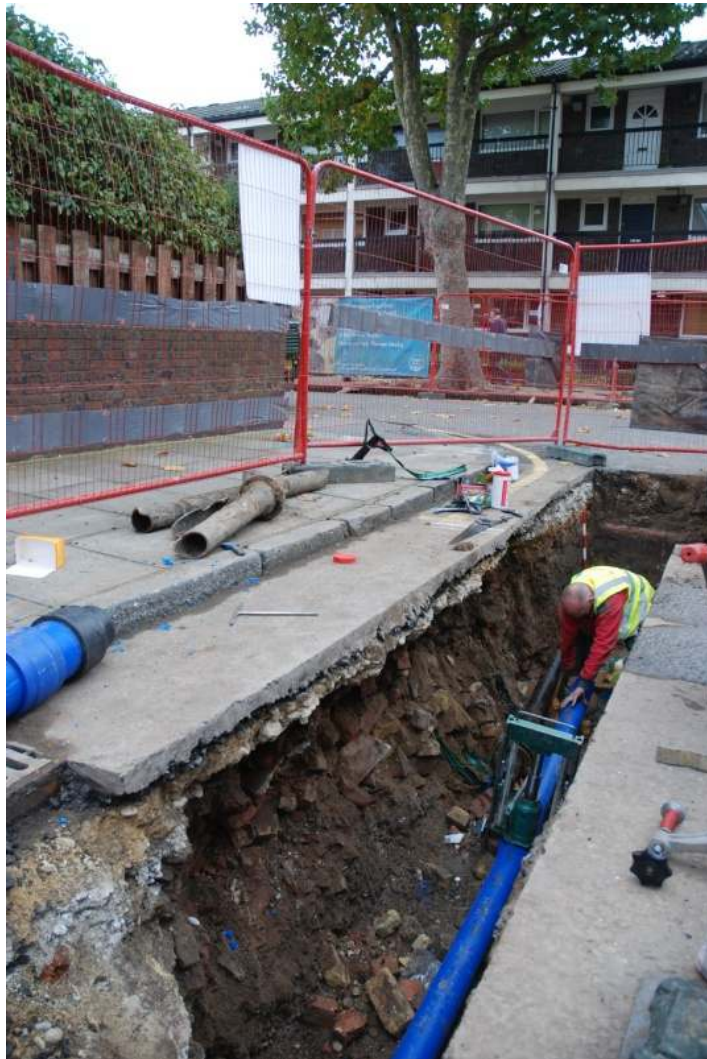
Figure 19: Trenching on Shetland Road at the junction with Stafford Road, looking west.
