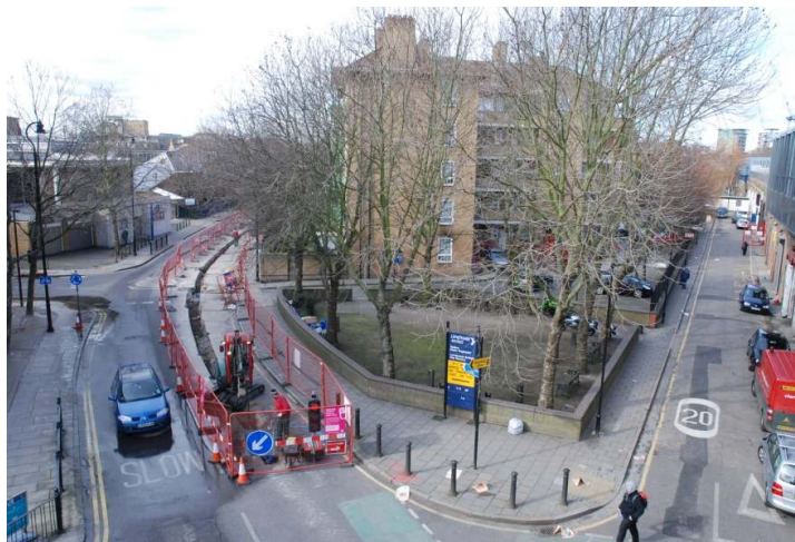
Figure 18: Elevated view of trenching on Limehouse Causeway at the junctions with Trinidad St and Salter Street.
