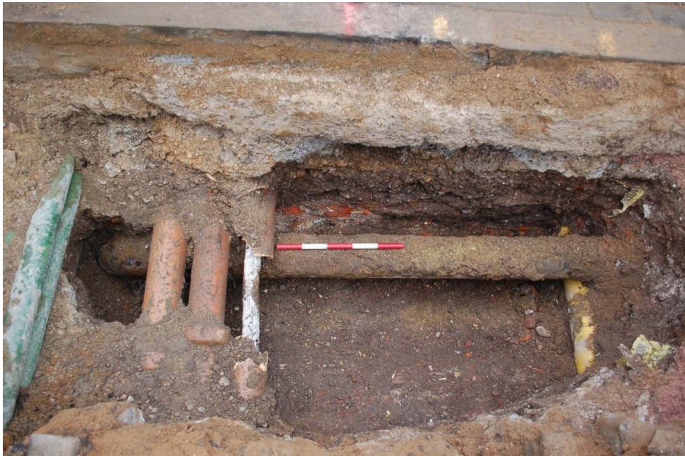
Figure 20: Truncated brick work in trenching on Grenade Street at the junction with Three Colt Street.
