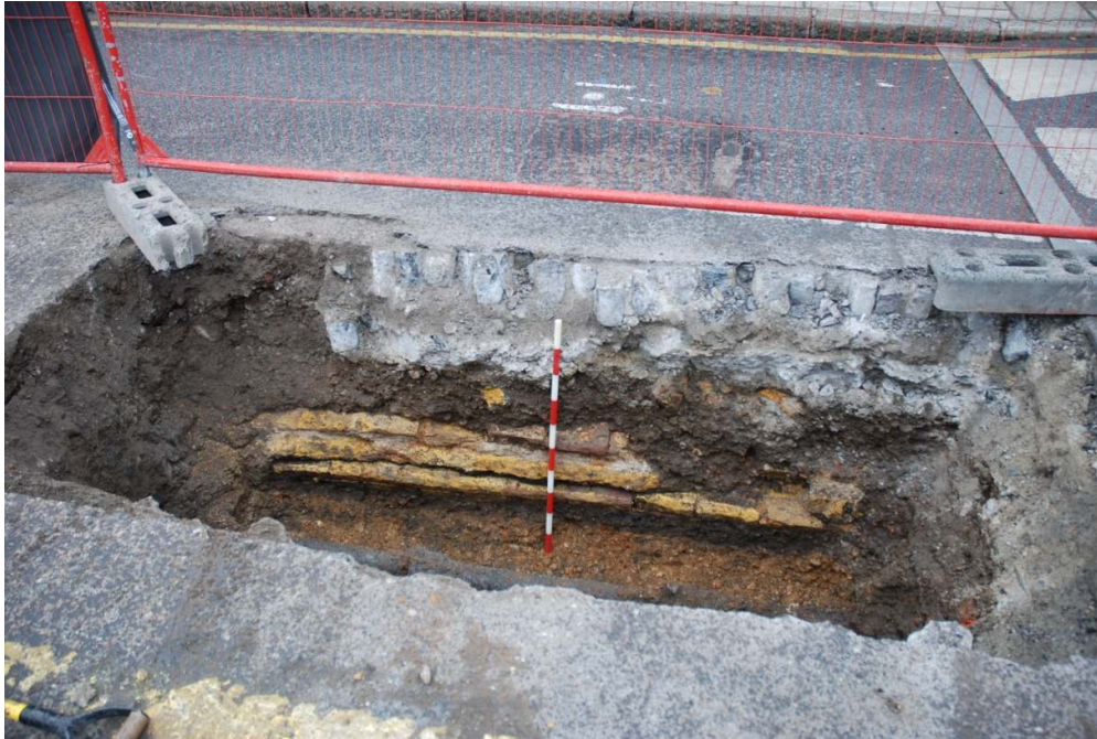
Figure 21: Truncated yellow-stock brick wall in the south facing section of trenching on Grenade Street at the junction with Rich Street.
