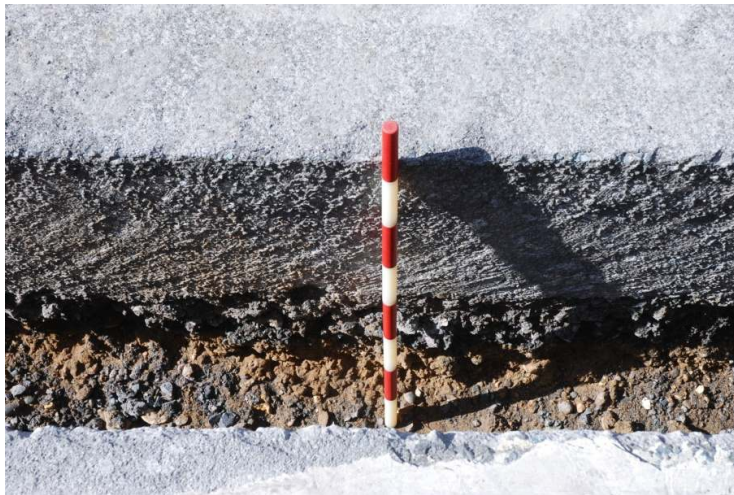
Figure 4: Trenching on the north side of West India Dock Road just south of the East India Dock Road junction.
