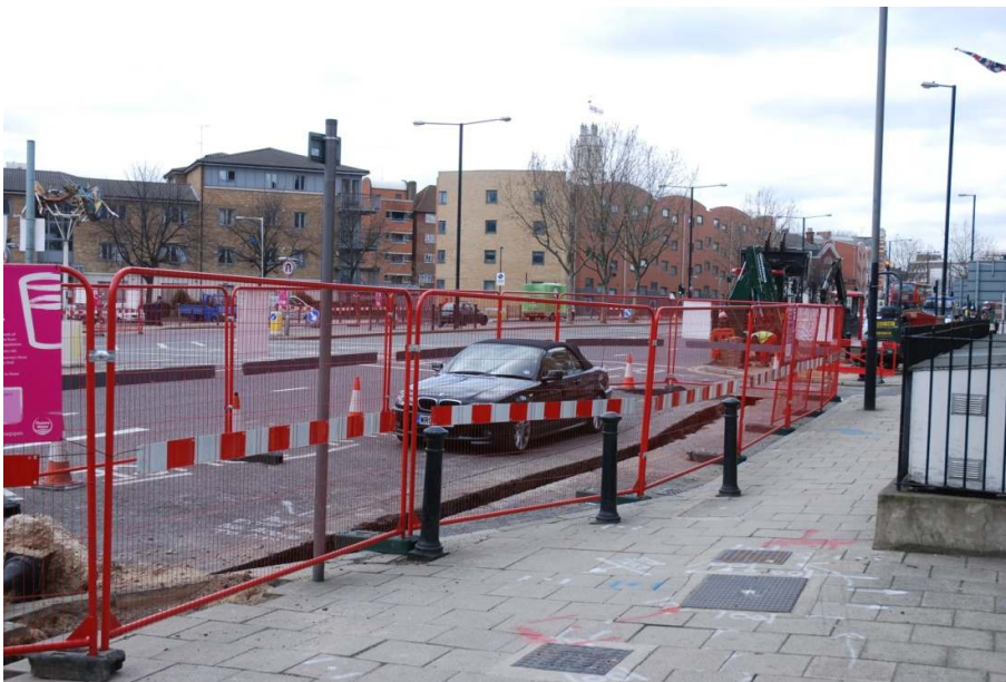
Figure 6: Trenching on the north side of West India Dock Road, immediately north of the Birchfield Street junction.
