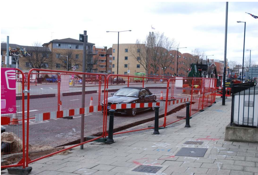
Figure 6: Trenching on the north side of West India Dock Road, immediately north of the Birchfield Street junction.
