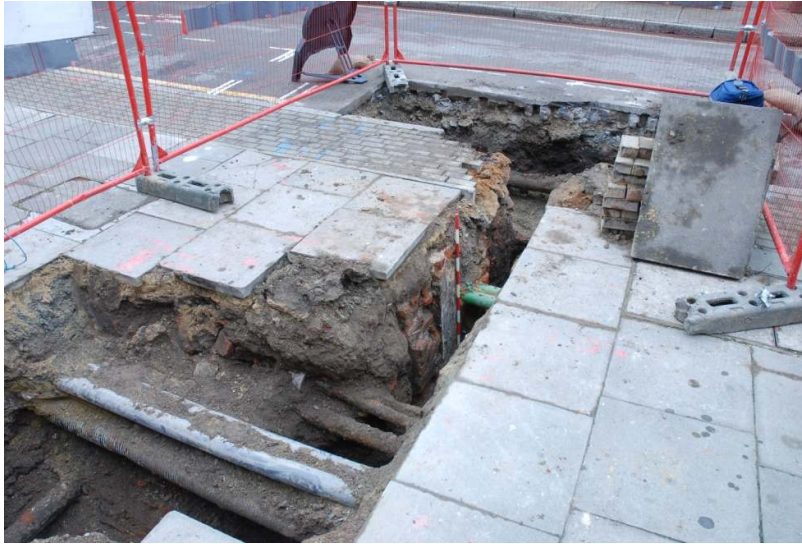
Figure 11: General view of trench north of Grenade St and the railway bridge.
