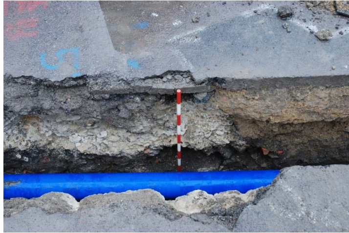
Figure 17: Section of trenching on Limehouse Causeway at the junction with Gill Street.
