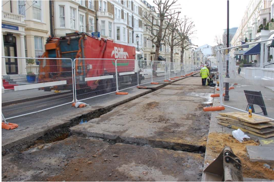
Figure 15: General view of trenching on Penywern Road, looking southwest towards Warwick Road.
