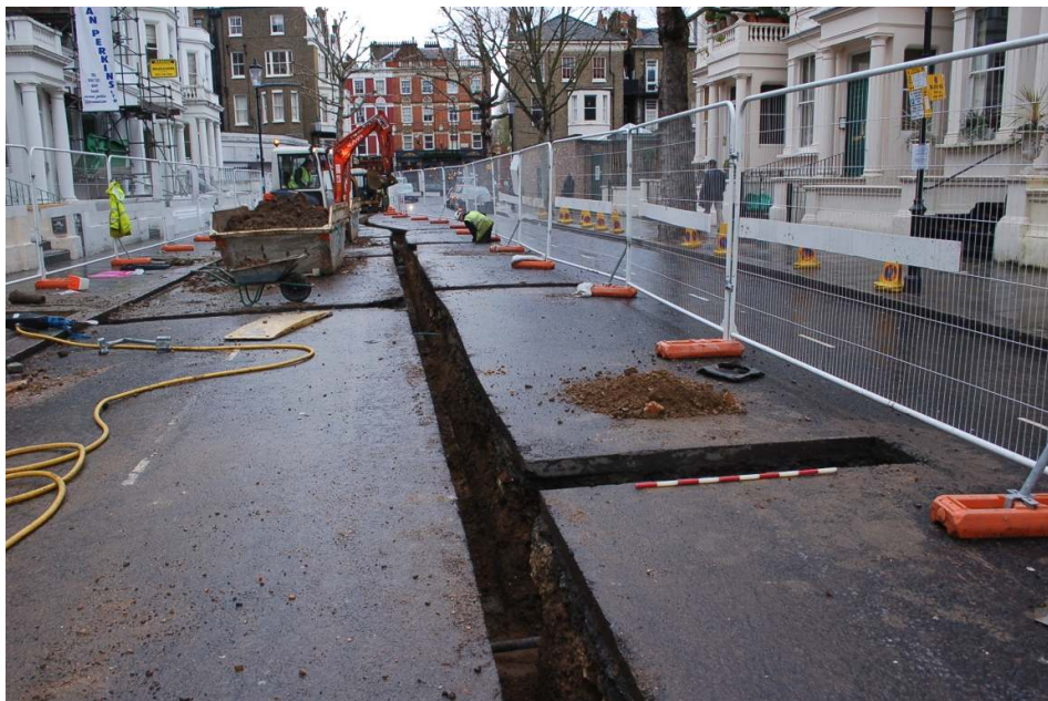
Figure 10: General view of trenching at the northeast end of Penywern Road, looking northeast towards the junction with Earl's Court Road.
