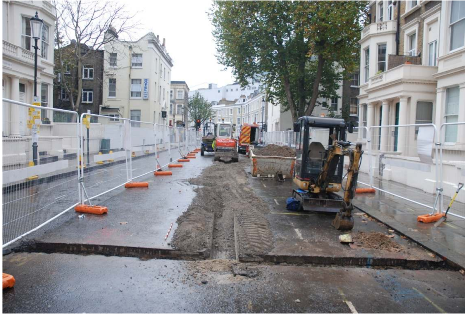
Figure 19: General view of trenching on Penywern Road at the southwest end towards the junction with Warwick Road.
