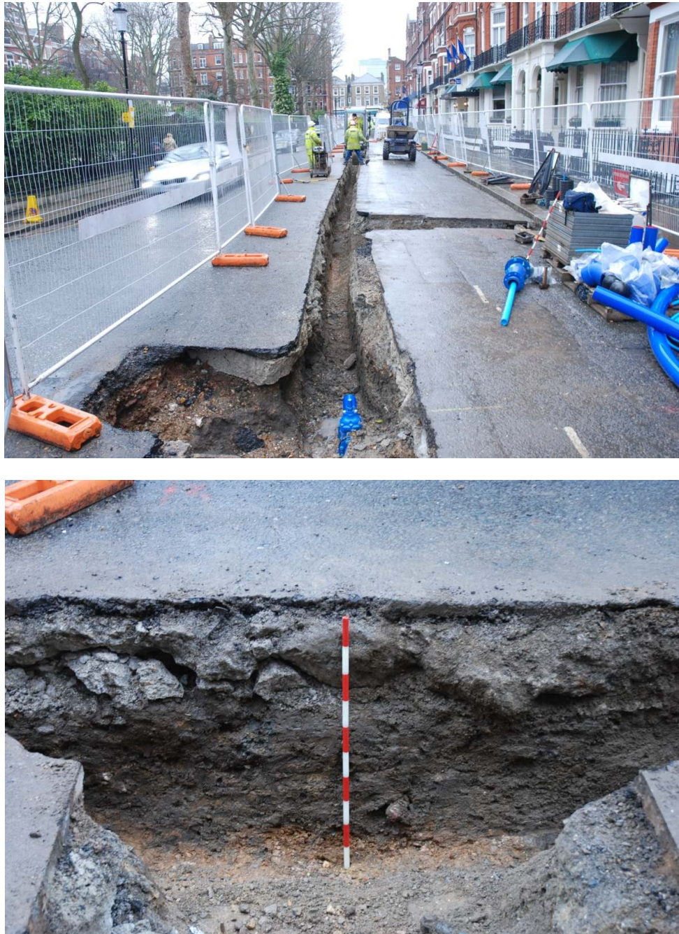
Figure 5: General (view southwest) and section (north-facing) views of Trench 2 on Barkston Gardens (1m scale).
