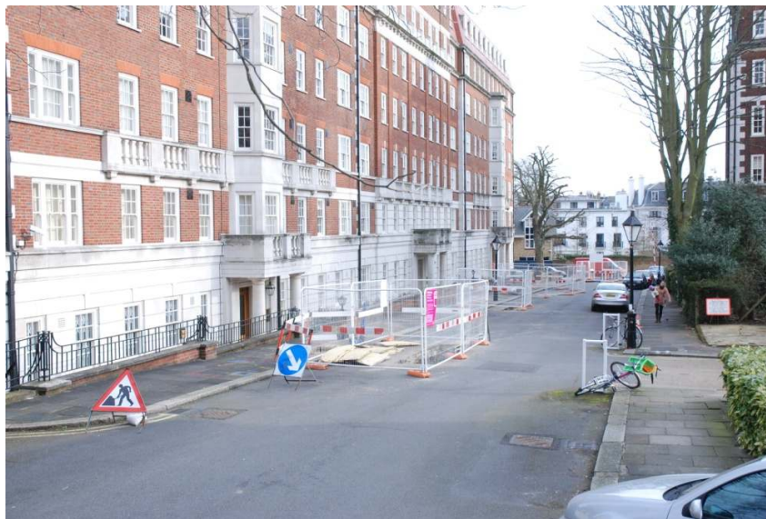
Figure 13: General view of trenching on Sheldrake Place, looking south to the junction with Duchess of Bedford's Walk.
