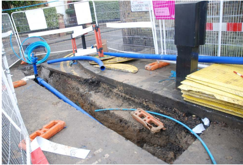
Figure 20: General view of trenching on Campden Hill Square, at the junction with Hillsleigh Road.
