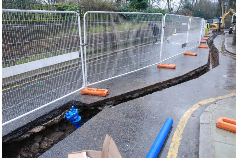
Figure 18: General view of trenching at the west end of Duchess of Bedford's Walk.
