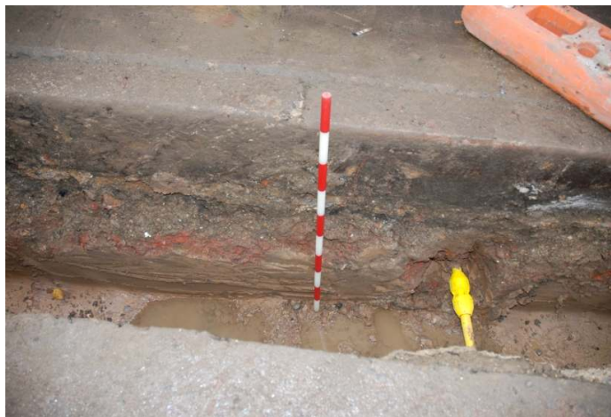
Figure 9: Section of trenching at the south end of Hillsleigh Road (1m scale).
