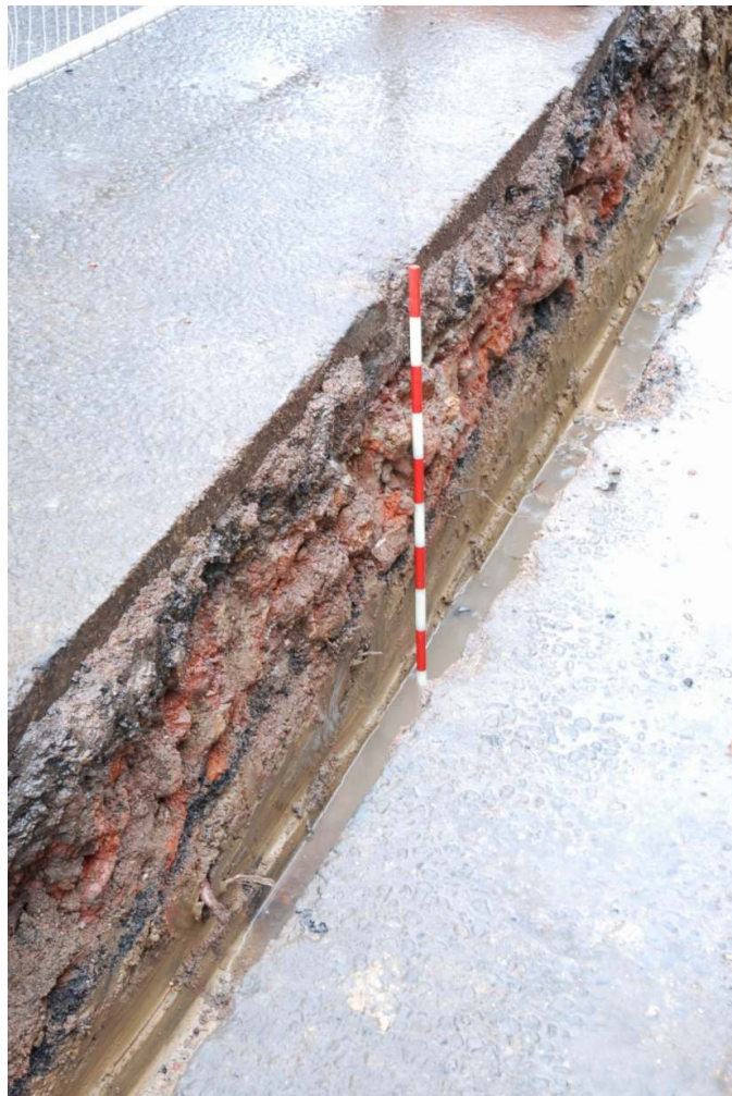
Figure 19: Section of trenching at the west end of Duchess of Bedford's Walk.
