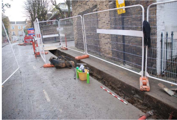
Figure 8: General view of trenching on Hillsleigh Road, looking south to the junction with Campden Hill Square.
