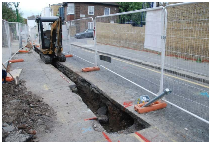
Figure 27: Trenching on Aubrey Road looking north to the junction with Campden Hill Square.
