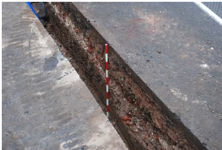
Figure 12: Section of trenching at the north end of Campden Hill Gardens (1m scale).
