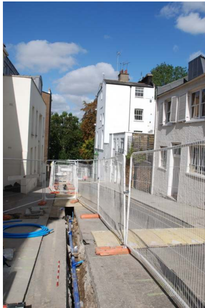
Figure 26: General view of trenching on Aubrey Road looking north to the junction with Holland Park Avenue.
