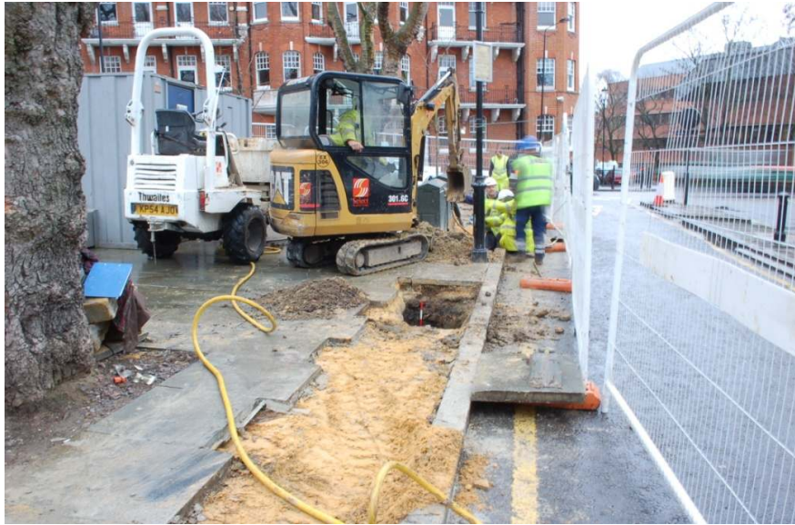
Figure 16: General view of trenching at the east end of Duchess of Bedford's Walk.
