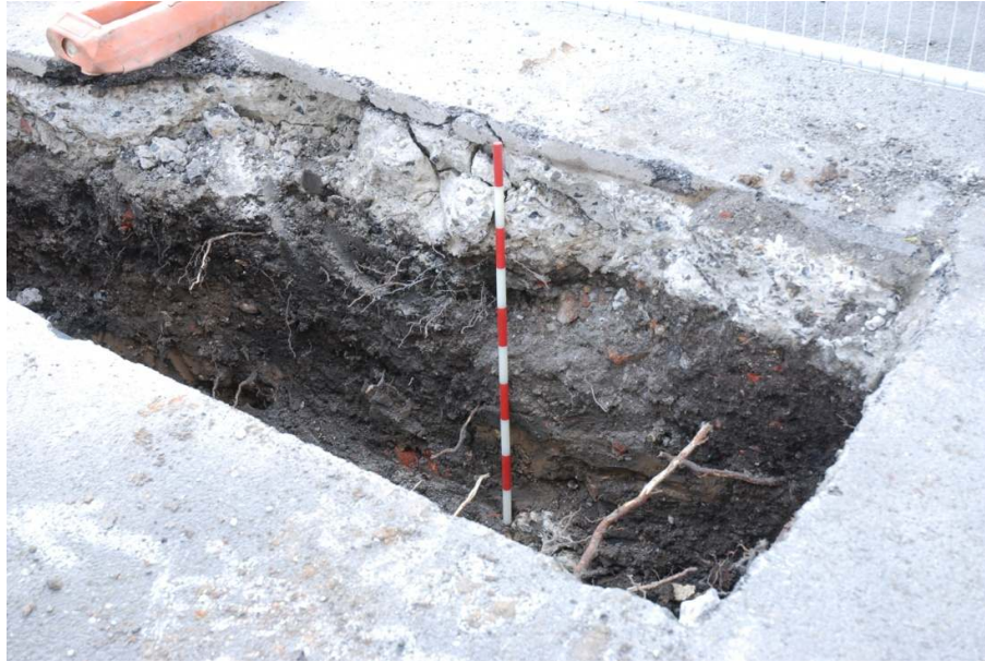
Figure 14: Section of trenching at the south end of Sheldrake Place (1m scale).
