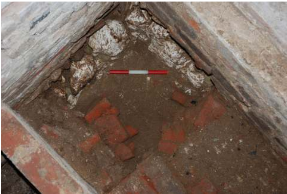
Fig. 87: Photograph of the excavated French drain, in the north-west corner of the dovecote.
