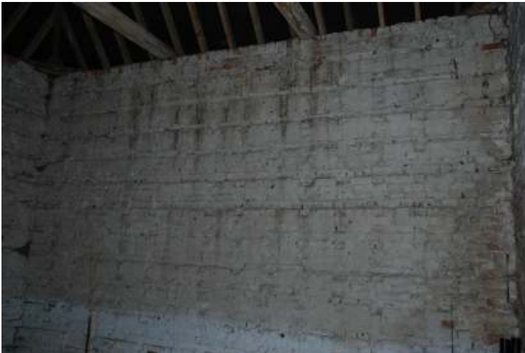
Fig. 64: Photograph of the nesting-holes in the Eastcote dovecote. The recessed line is where the tile 'ledge' would have projected out from; with the three courses of brickwork above this containing the infilled holes and projecting brickwork divisions between the nesting-boxes.
