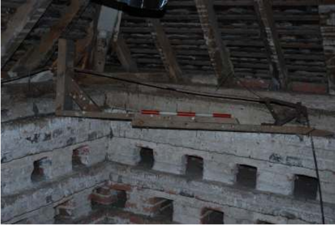
Fig. 152: Photograph showing the wooden contraption in the upper floor of the roof, which connected the bell pull to the bell.
