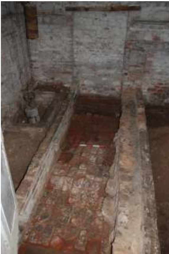
Fig. 127: Photograph showing the ‘ground-floor raising plinths’, taken from the western doorway into the dovecote.
