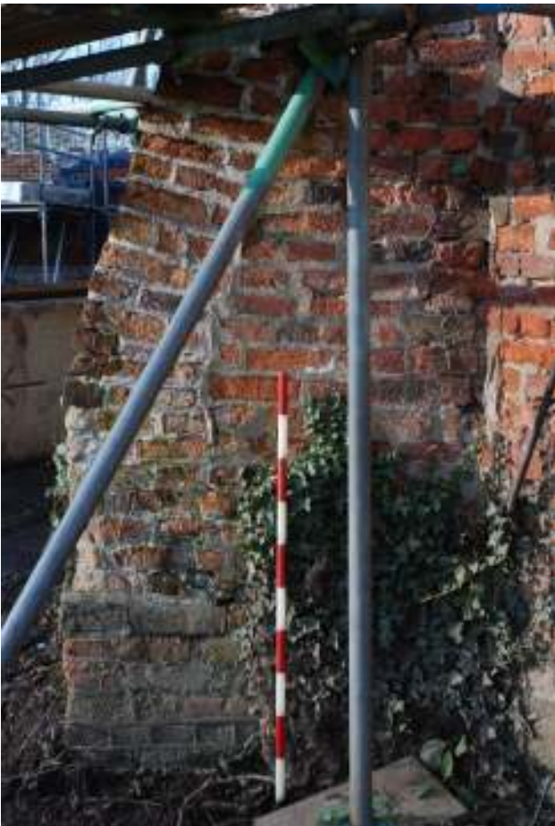
Fig. 98: Close-up photograph of the eastern side of the south-western buttress. This clearly shows the line of the later patching.
