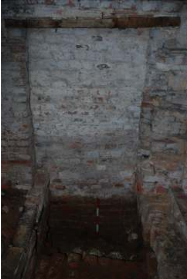
Fig. 121: Photograph of the interior of the blocked-up eastern doorway. This clearly shows how it has been infilled.
