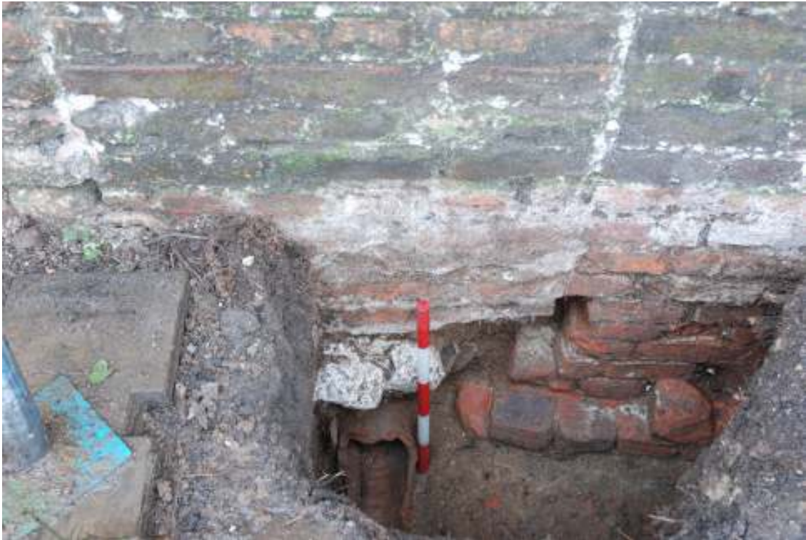
Fig. 90: Photograph of the exterior of the eastern doorway. This shows the drainpipe running through from the inside of the dovecote.
