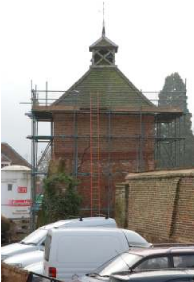
Fig. 50: Photograph of the exterior of the northern wall of the dovecote. The new build is above, and including, the moulded course of brickwork.
