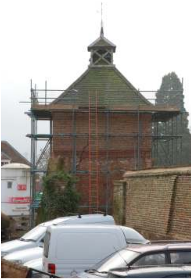
Fig. 19: Photograph of the exterior northern wall of the dovecote. The original build was up to the lower part of the moulded courses of brickwork.
