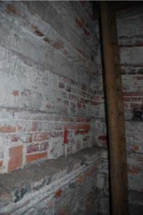
Fig. 62: Photograph of the nesting-holes in the south-west corner. The lower nesting-holes are part of the original build (tile and dentil courses), whereas the upper nesting-holes are part of the rebuild (brick ledges). The scale is standing at the rebuild level and the highest point of the original walls.
