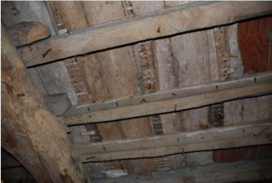
Fig. 105: Photograph of common joists on the ground floor, supported by more substantial north-south ceiling beams.
