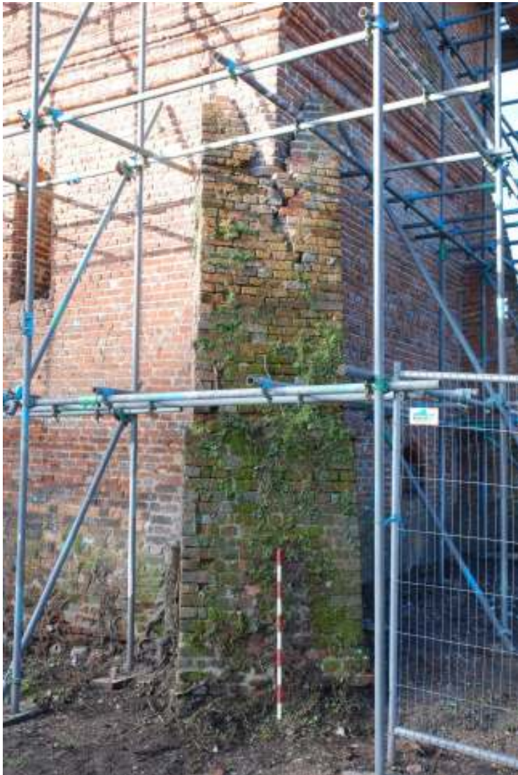
Fig. 94: Photograph of the front of the south-eastern buttress. This clearly shows the buttress being splayed around the dovecote wall. The 'step' out, just beneath the scaffolding, and different patching beneath this can also be seen.
