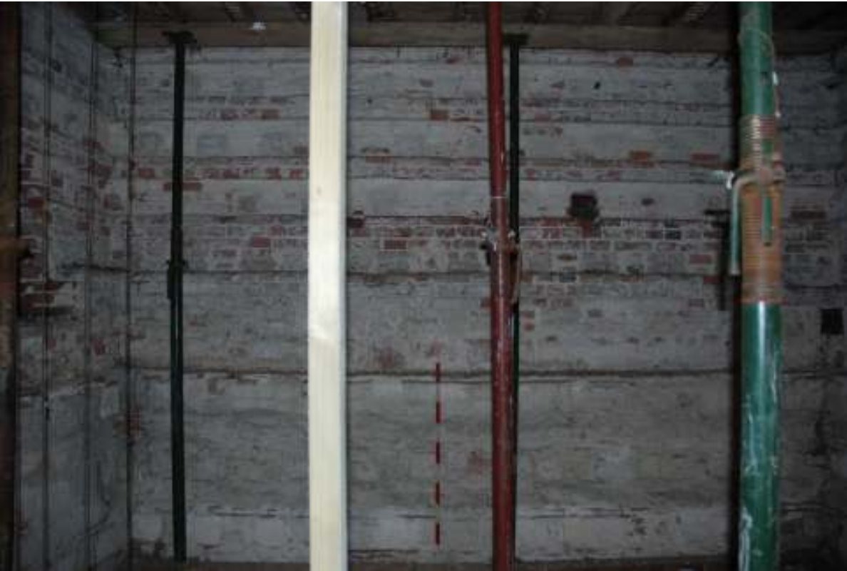
Fig. 59: Photograph of the interior eastern wall – first floor. The rebuild is from c.0.1m above the top of the scale, where the nesting holes are different.
