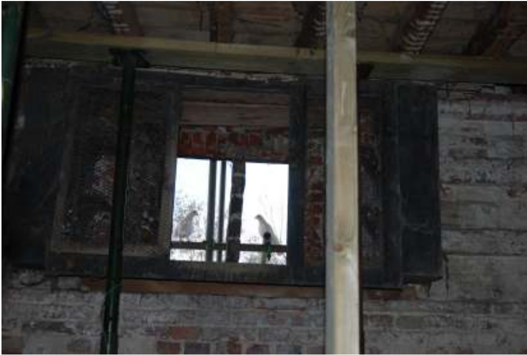
Fig. 77: Photograph of the window in the western wall (from the inside). Two doves are perched on the scaffolding outside this window.
