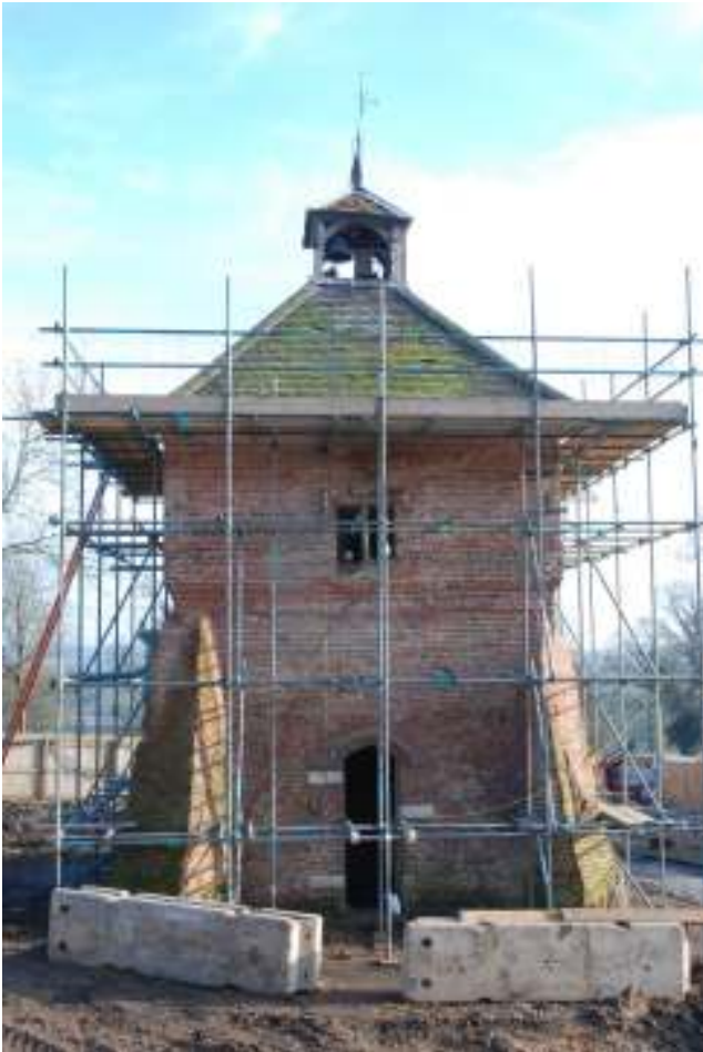
Fig. 68: Photograph of the exterior of the western wall of the dovecote. This is all part of the rebuild, excluding the later doorway.
