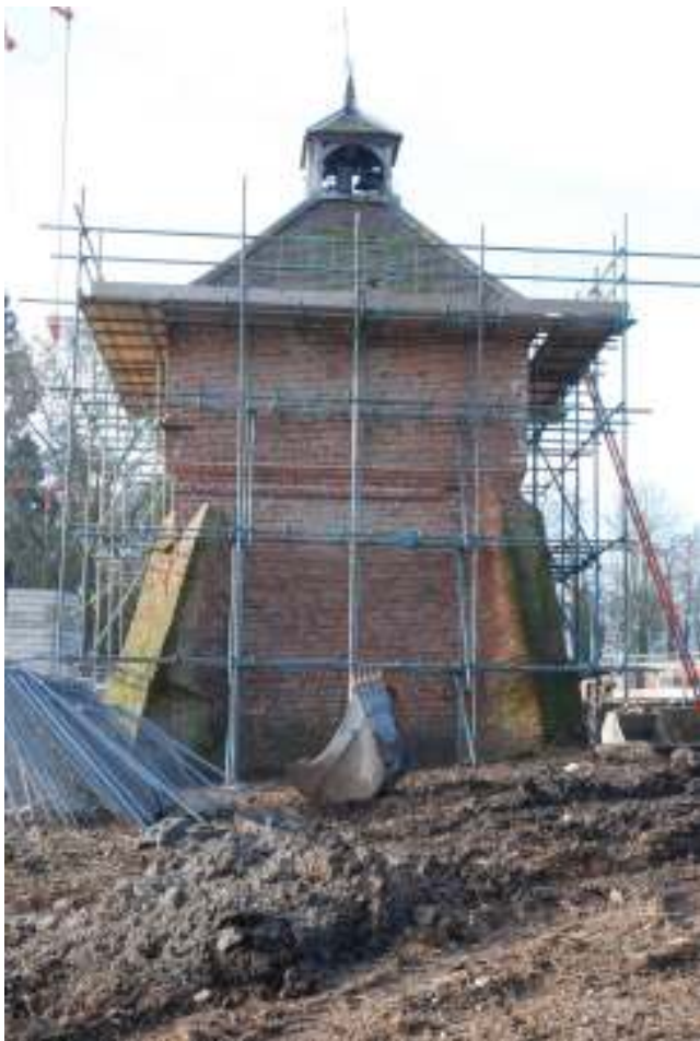
Fig. 20: Photograph of the exterior eastern wall of the dovecote. The original build was up to the lower part of the moulded courses of brickwork. Sadly, the blocked doorway is directly behind the machine bucket in this photograph.
