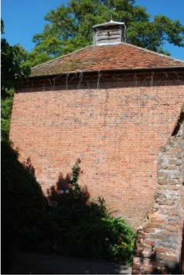
Fig. 52: Photograph of the exterior of the dovecote at Eastcote, clearly showing its regular 'Flemish' bond.
