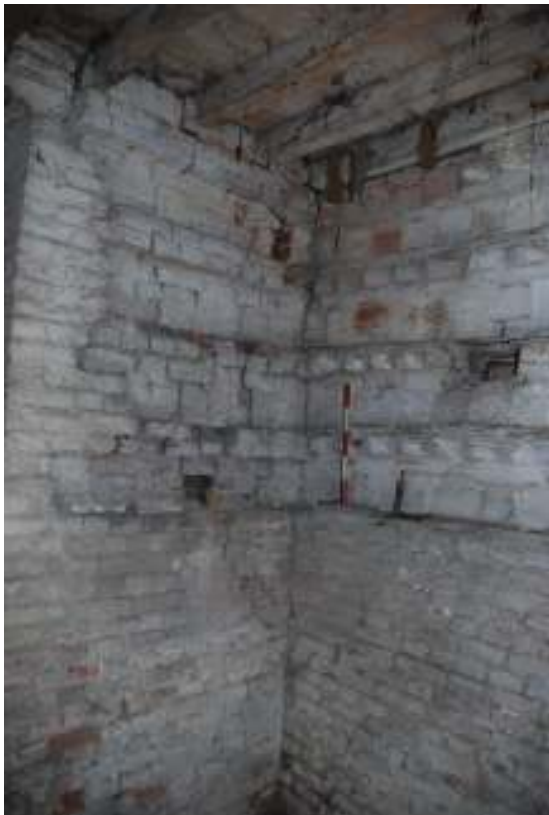
Fig. 48: Photograph of the corner of the northern and western walls (ground-floor). This shows how the lower re-facing of the northern wall runs behind the lower part of the western wall.
