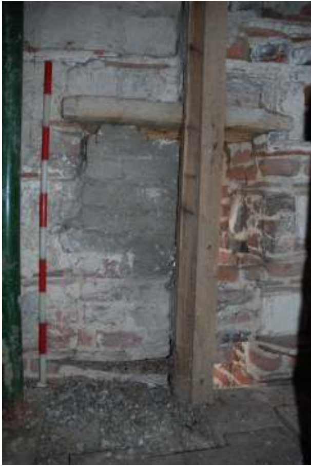
Fig. 33: Photograph of the window in the southern wall of the dovecote (from the inside). This clearly shows the timber lintel, going into the nesting holes either side of it, with no indication that the window (or lintel) was inserted at a later date.
