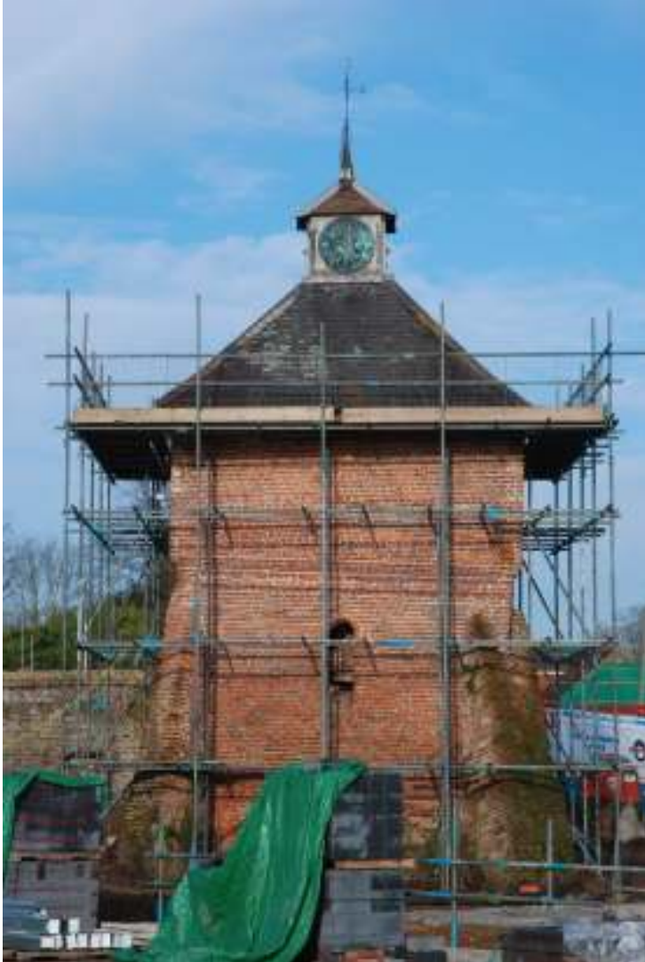
Fig. 18: Photograph of the exterior southern wall of the dovecote. The original build was up to the lower part of the moulded courses of brickwork, and included the southern window.
