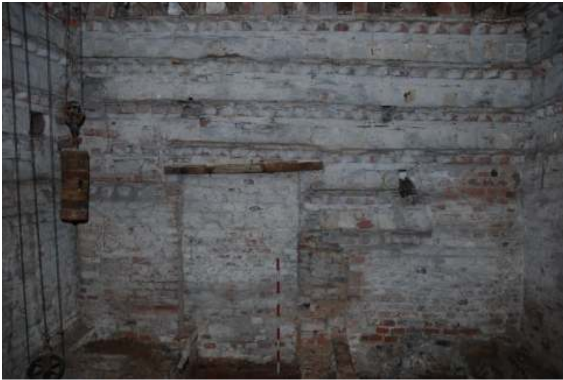
Fig. 26: Photograph of the interior eastern wall – ground floor. Original build visible from c.100mm above the scale (battered re-facing below this, with the original eastern doorway (now blocked-in). See fig. 47 for clear explanation of which parts are part of the later battered re-facing.
