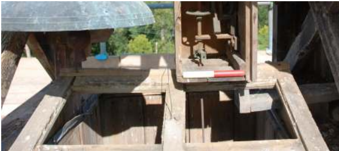
Fig. 156: Photograph of the remaining wooden frames at the base of the cupola, which would have held glass and prevented doves from entering the structure.
