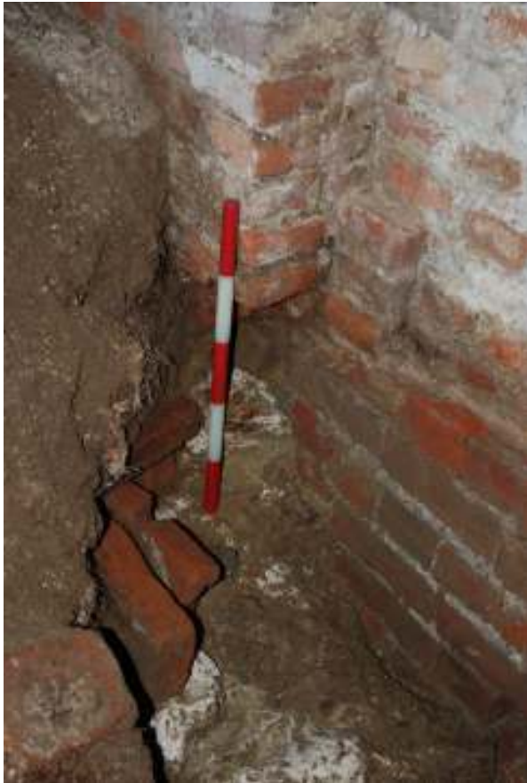
Fig. 45: Photograph of the northern side of the eastern doorway. This shows the 'gap' between the existing (re-faced) wall and the earlier wall, at the base of the wall.
