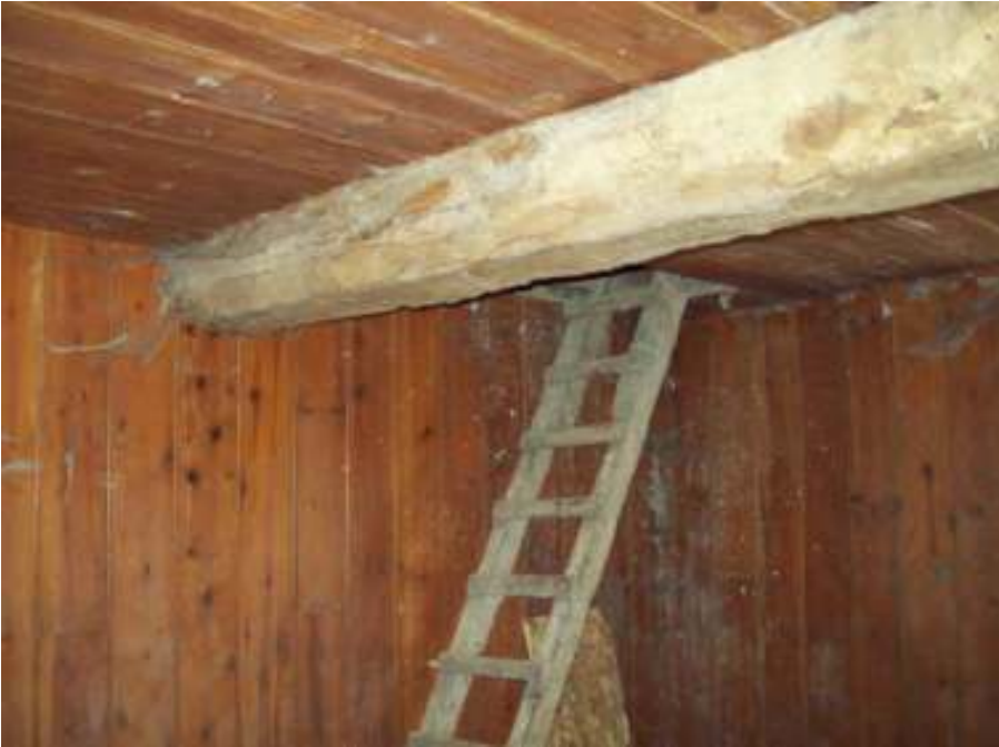
Fig. 160: Photograph supplied by Clancy Docwra Developments Ltd which shows the wooden panelling of the interior of the dovecote, ground floor.
