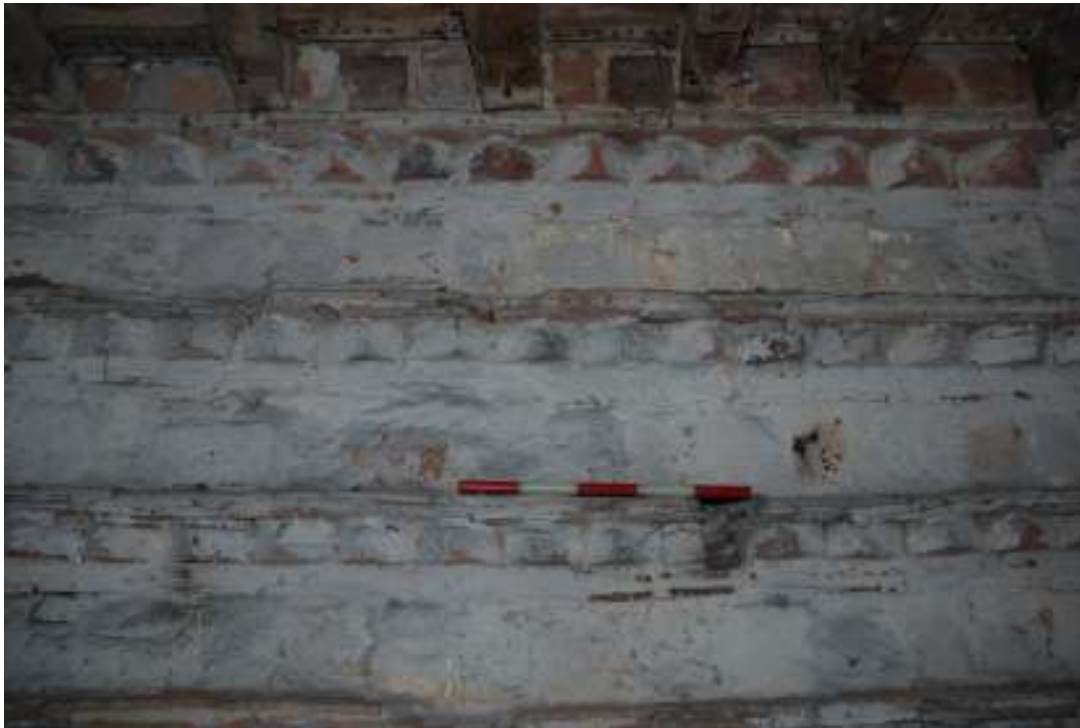
Fig. 28: Photograph of blocked nesting holes in the original build (eastern wall, ground floor). These are sandwiched between two tile courses and a dentil course of brickwork.
