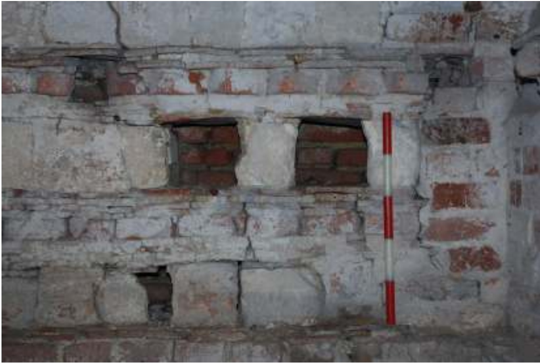
Fig. 29: Photograph of nesting holes in the original build (eastern wall, ground floor) – with some of these opened up to show the interiors.
