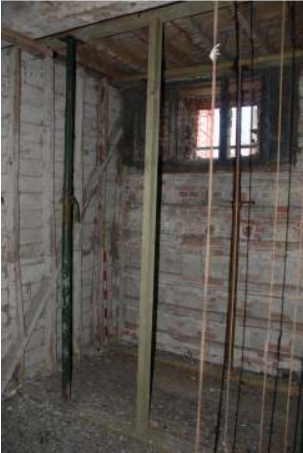
Fig. 70: Photograph of the interior western wall of the dovecote – first floor. This is all part of the rebuild.
