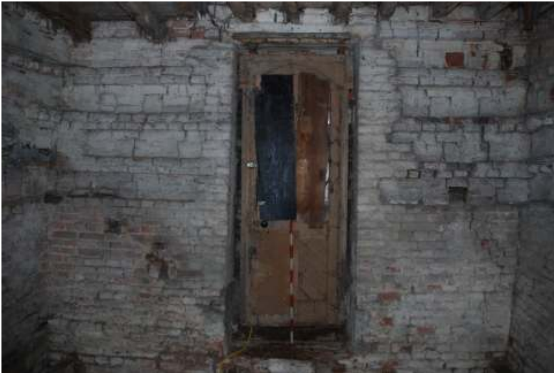
Fig. 69: Photograph of the interior western wall of the dovecote – ground floor. This is all part of the rebuild.
