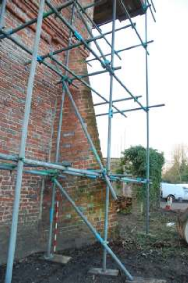
Fig. 91: Photograph of the southern side of the north-eastern buttress. This clearly shows the grey mortar that has attached the buttress onto the main dovecote structure.
