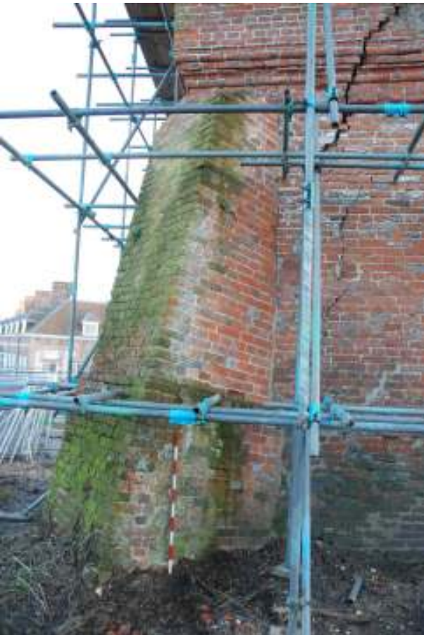
Fig. 92: Photograph of the northern side of the north-eastern buttress. This clearly shows the buttress overlapping the moulded course of brickwork.
