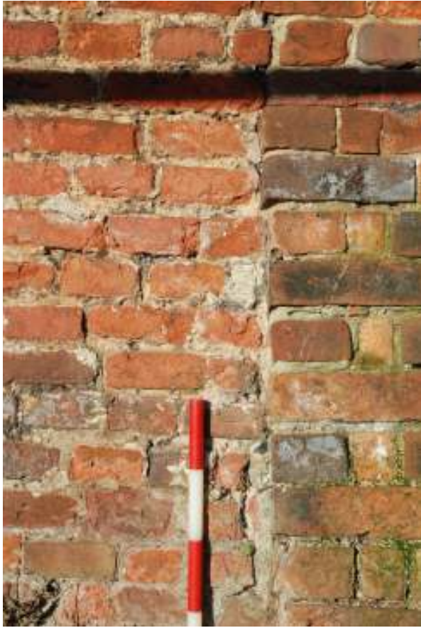
Fig. 129: Close-up photograph of the patching on the southern wall. This clearly shows the difference between the original wall (left side of photo) and the patching (right side of photo).
