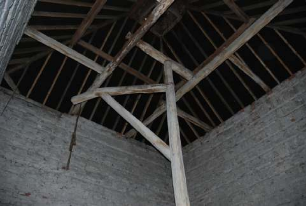
Fig. 81: Photograph of the interior roof construction and potence in the dovecote at Eastcote.
