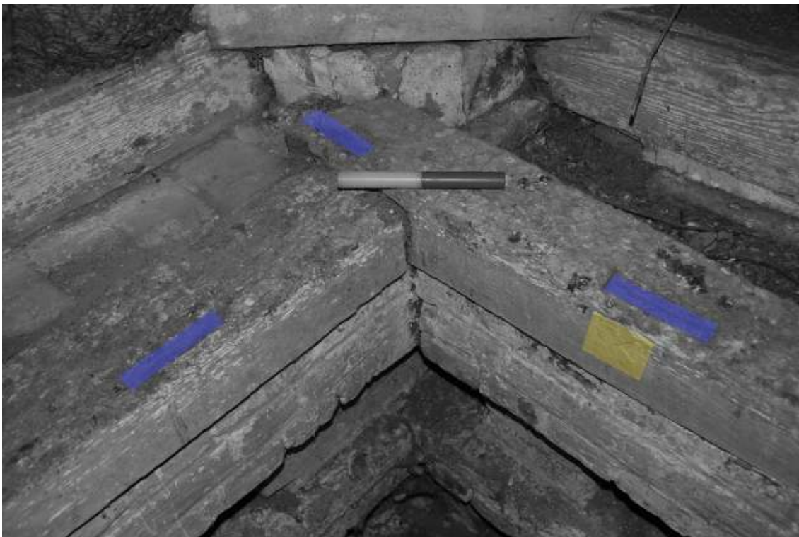
Fig. 80: Annotated photograph of the earlier timber along the top of the wall (south-east corner of the dovecote). Three mortices can clearly be seen (highlighted in blue), two on the right hand piece of timber and cut away behind the scale by the later roof construction. One carpenter's mark ('X') is visible on the right-hand timber (highlighted in yellow).
