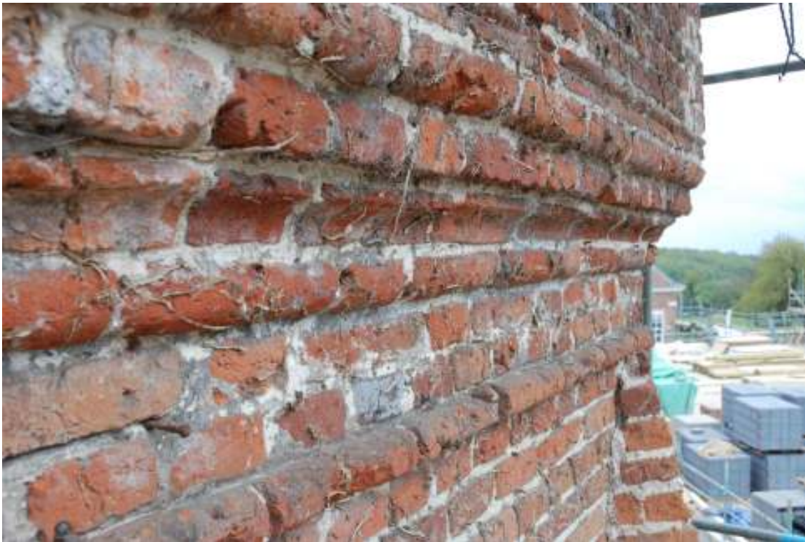
Fig. 65: Photograph of the moulded courses of brickwork, at the southern corner of the western wall.
