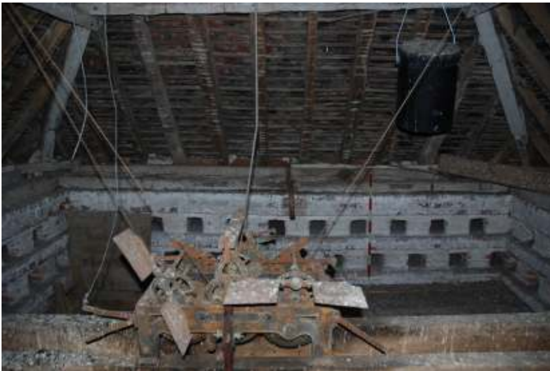
Fig. 71: Photograph of the interior western wall of the dovecote – second floor. This is all part of the rebuild.
