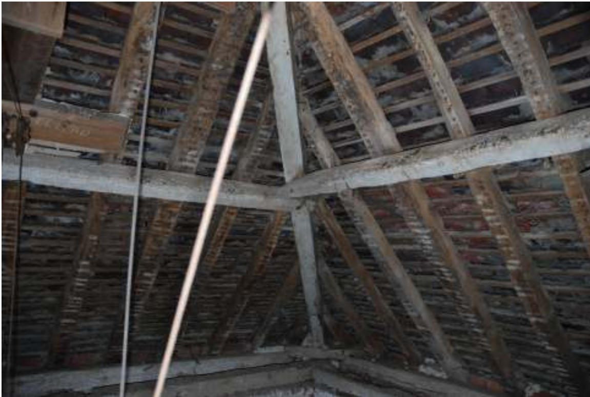
Fig. 118: Photograph of a corner of the interior roof of the dovecote. This clearly shows a hip-rafter; purlins; rafters; and lathes.
