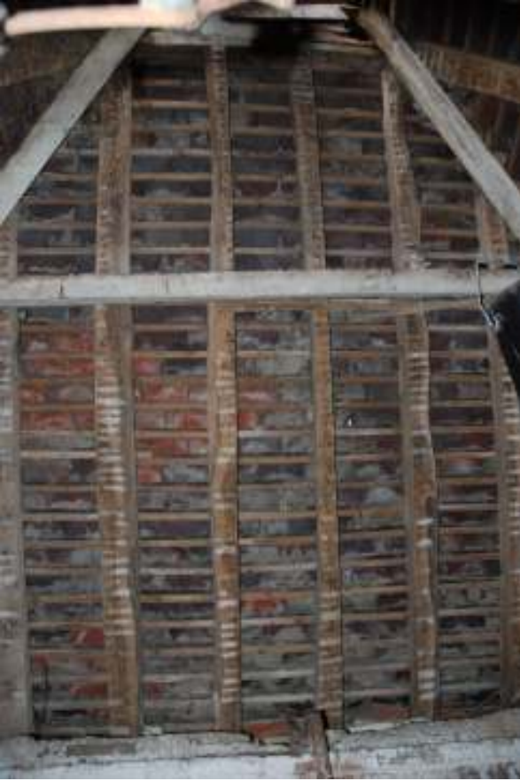
Fig. 119: Photograph of the interior roof of the dovecote. This clearly shows the variation in size of the common rafters, and extremely regular horizontal laths (to hold the tiles).
