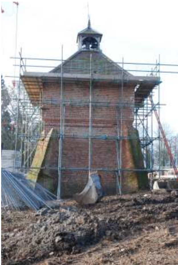
Fig. 51: Photograph of the exterior of the eastern wall of the dovecote. The new build is above, and including, the moulded course of brickwork.
