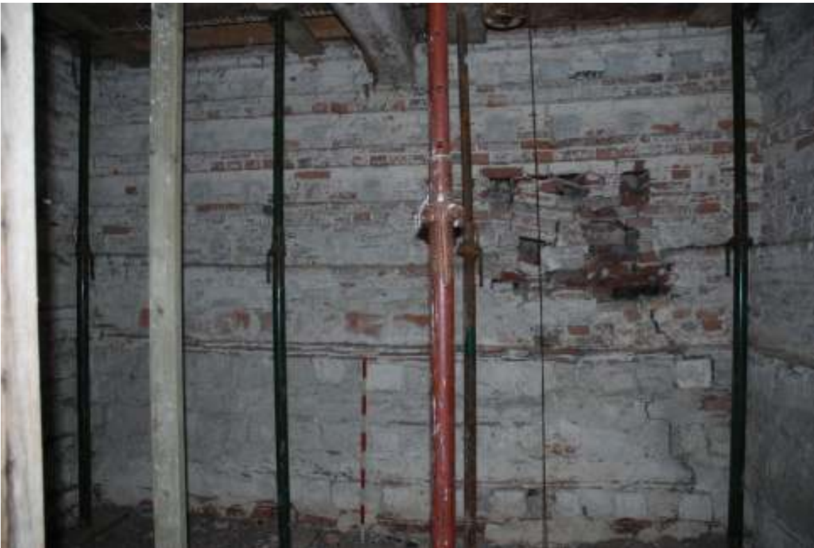
Fig. 56: Photograph of the interior northern wall – first floor. The rebuild is from c.0.2m above the top of the scale, where the nesting holes are different.
