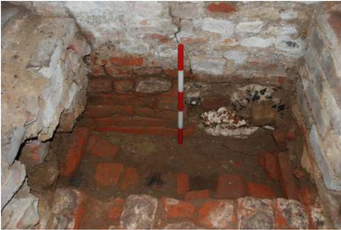
Fig. 39: Photograph of the small area of brick foundations observed in the western wall, continuing to the left of the frame behind the much later ground-raising plinths. This is possibly evidence for an earlier door in this wall.
