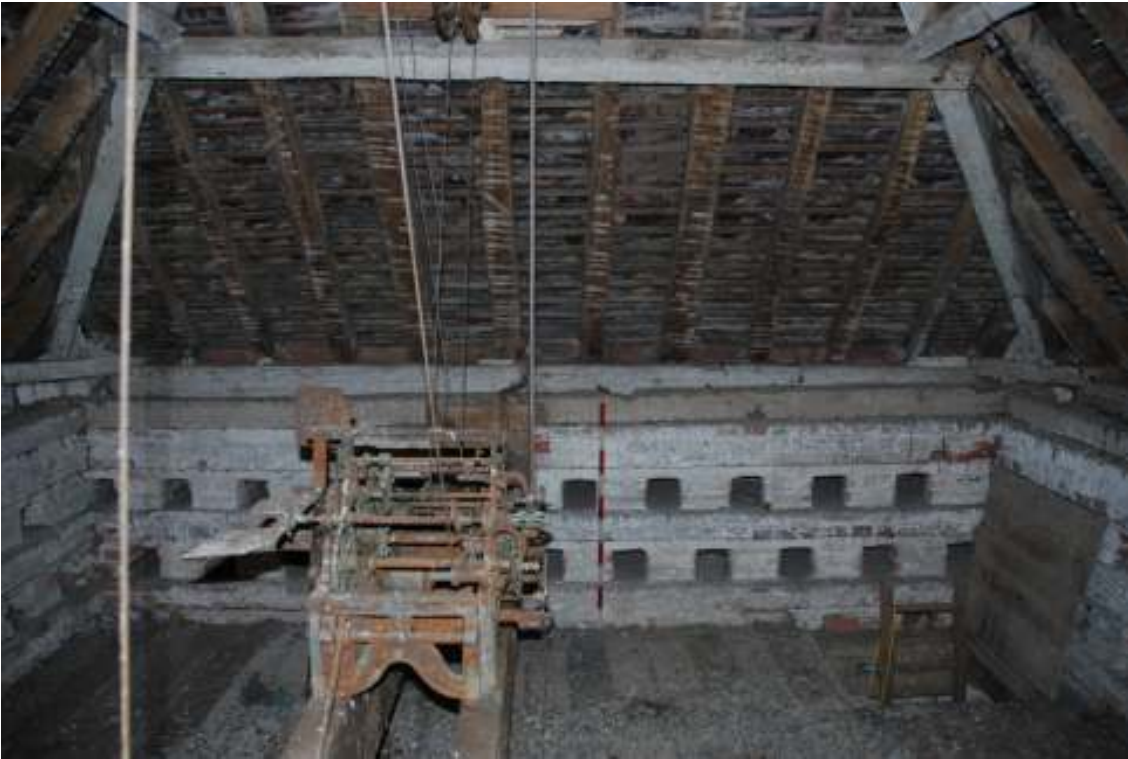
Fig. 55: Photograph of the interior southern wall – second floor, with nesting-holes still open. This is all part of the rebuild.
