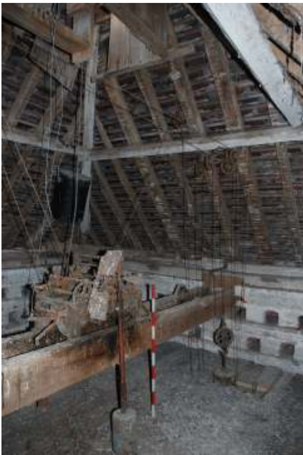
Fig. 139: Photograph showing the series of wires, pulleys, etc, connecting the clock mechanism (striking and chiming train) to the cupola.
