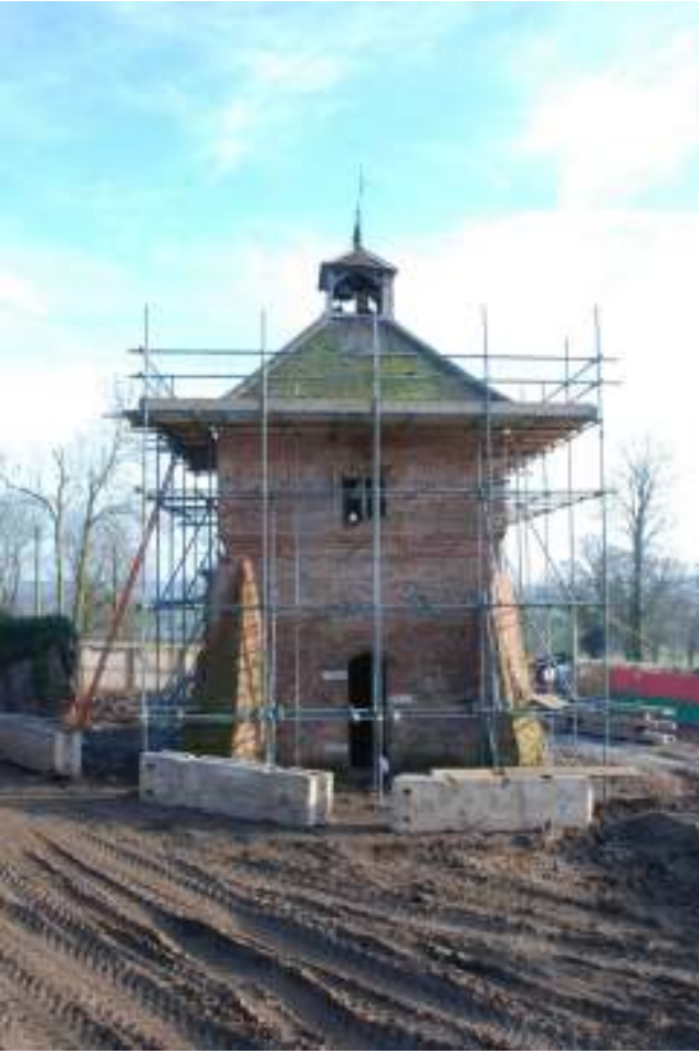
Fig. 30: Photograph of the exterior western wall of the dovecote. The apparent 'jettied' construction of the structure (with the part above the moulded courses clearly sticking out further than the lower part of the structure) provides a possible indication of an earlier timber jettied structure.
