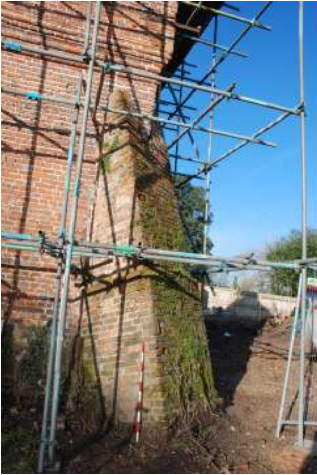
Fig. 95: Photograph of the western side of the south-eastern buttress.
