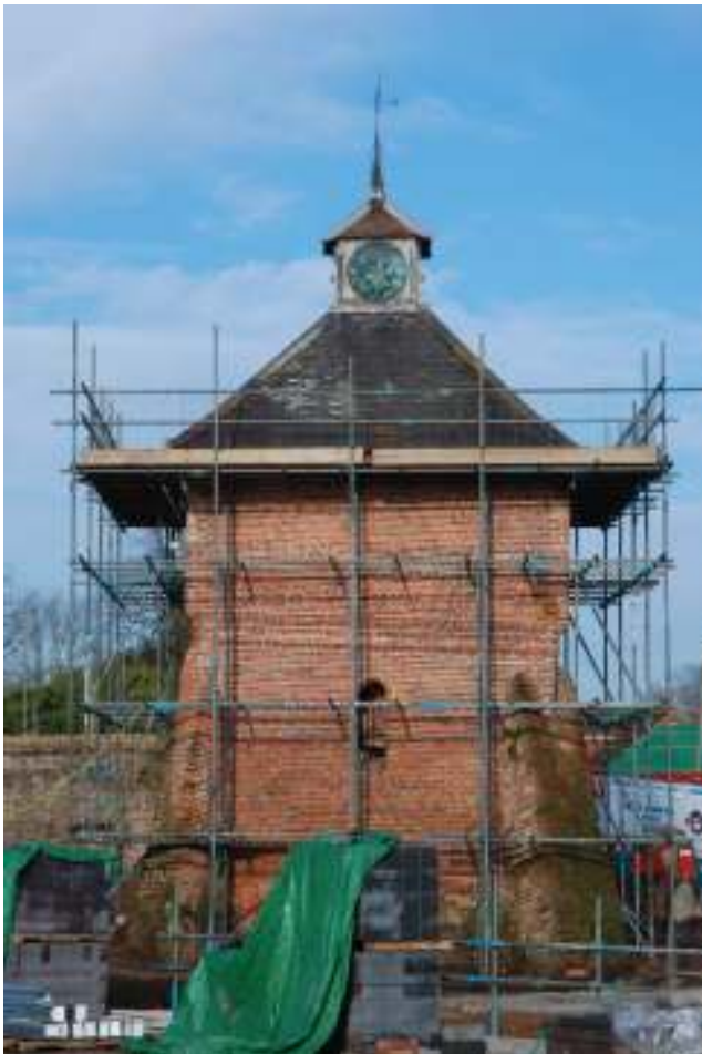
Fig. 49: Photograph of the exterior of the southern wall of the dovecote. The new build is above, and including, the moulded course of brickwork.
