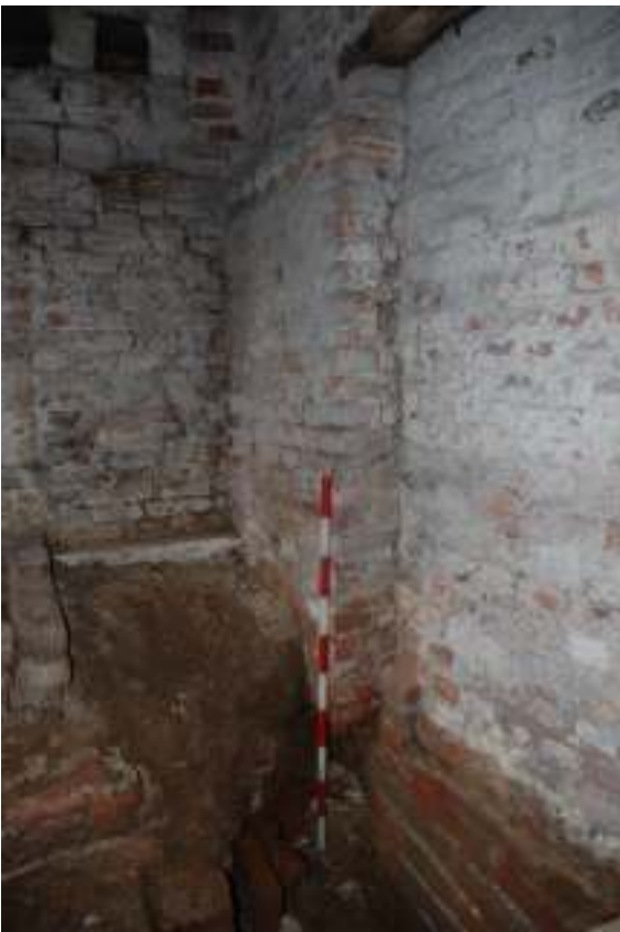
Fig. 44: Photograph of the northern side of the blocked-up eastern doorway. This shows the 'gap' between the existing (re-faced) wall and the earlier wall.
