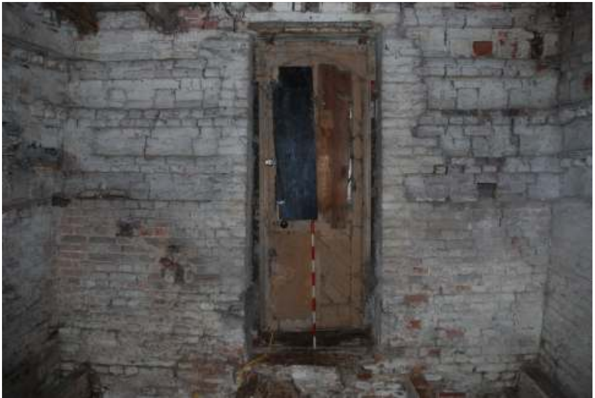
Fig. 125: Photograph of the interior of the western doorway. This clearly shows how it was inserted at a later date, with the nesting-holes surrounding the doorway having partially been cut away and bricked over.
