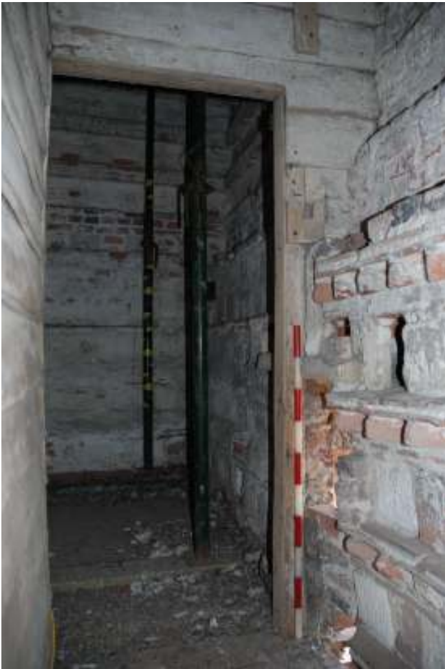
Fig. 108: Photograph from inside the wooden chamber, showing how the tile/dentil courses and nesting-holes are not covered over / blocked-up within the chamber; but are in the main first floor room.
