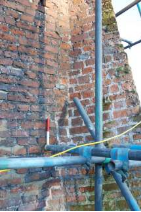
Fig. 102: Photograph of the eastern side of the north-western buttress. This clearly shows how the buttress is 'keyed-in' to the main dovecote wall.
