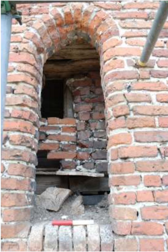
Fig. 110: Photograph of the southern window, clearly showing the two separate phases of blocking (along the line of the internal wooden chamber).
