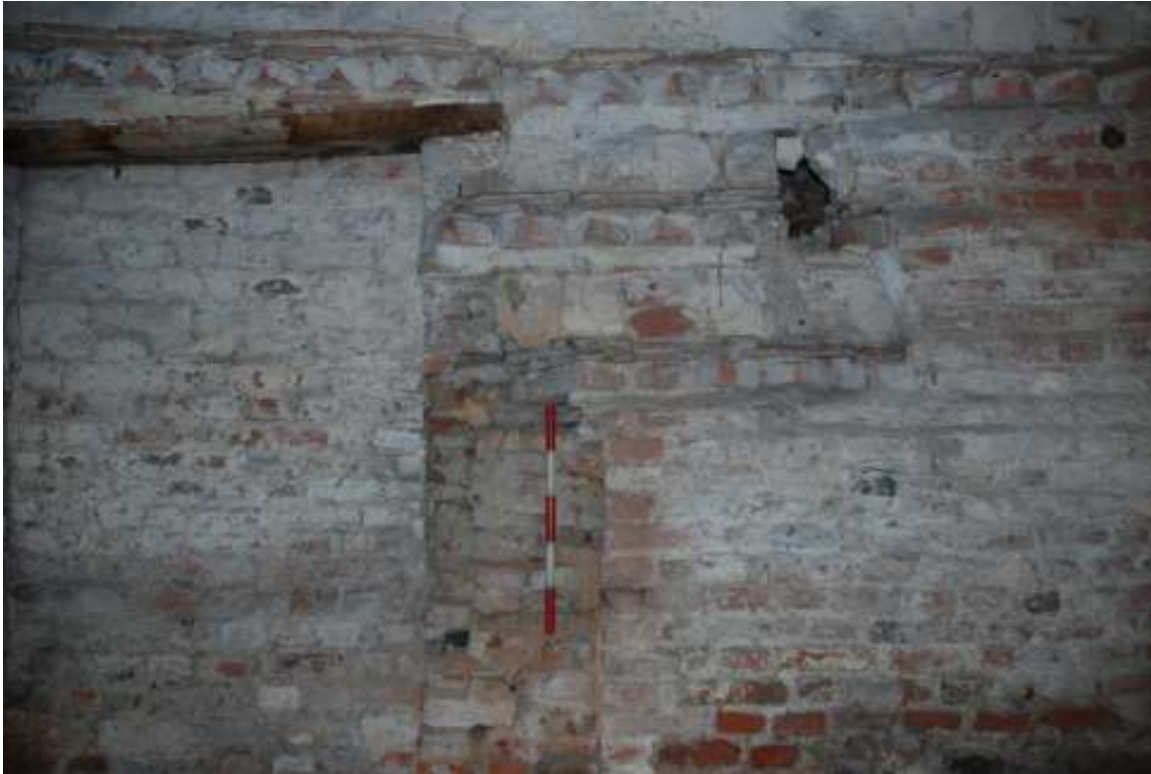
Fig. 46: Photograph of the southern side of the eastern doorway. This shows the small line of blocked nesting holes (just above the scale) that exist at this height in only this small area, before they are covered up by the re-facing (to the right of the photo).
