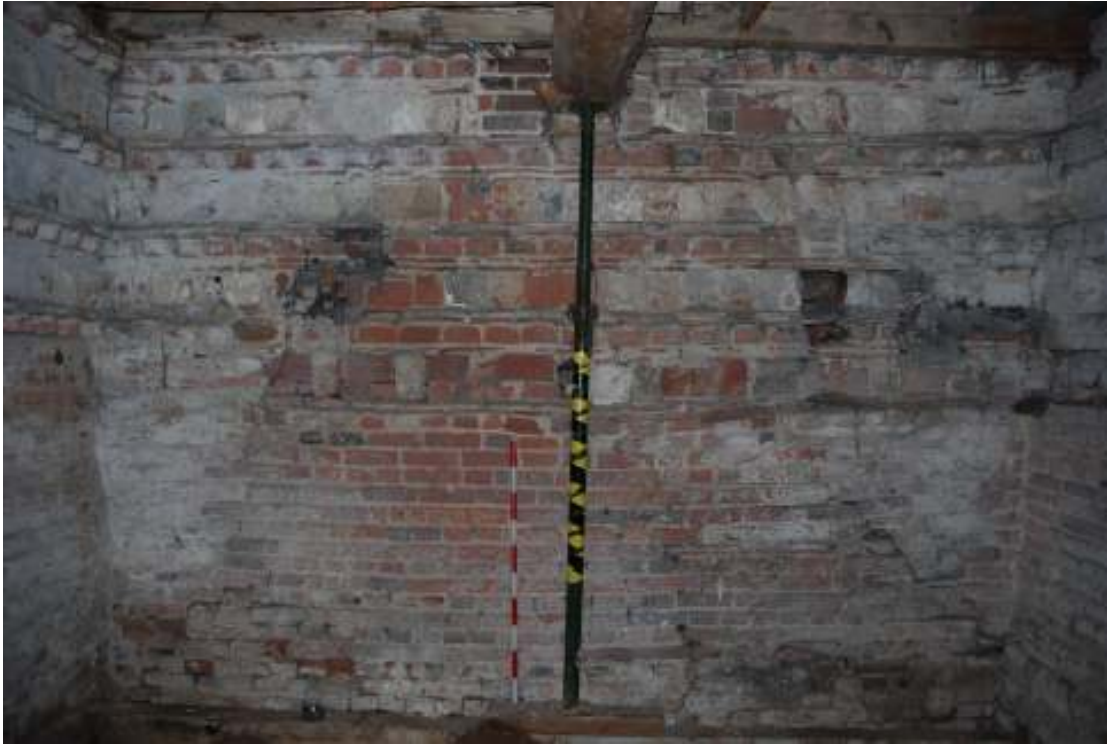
Fig. 22: Photograph of the interior southern wall of the dovecote – ground floor. Original build visible from c.100mm above the scale (battered re-facing below this). Rows of nesting-boxes are visible, although the holes themselves have almost all been blocked.
