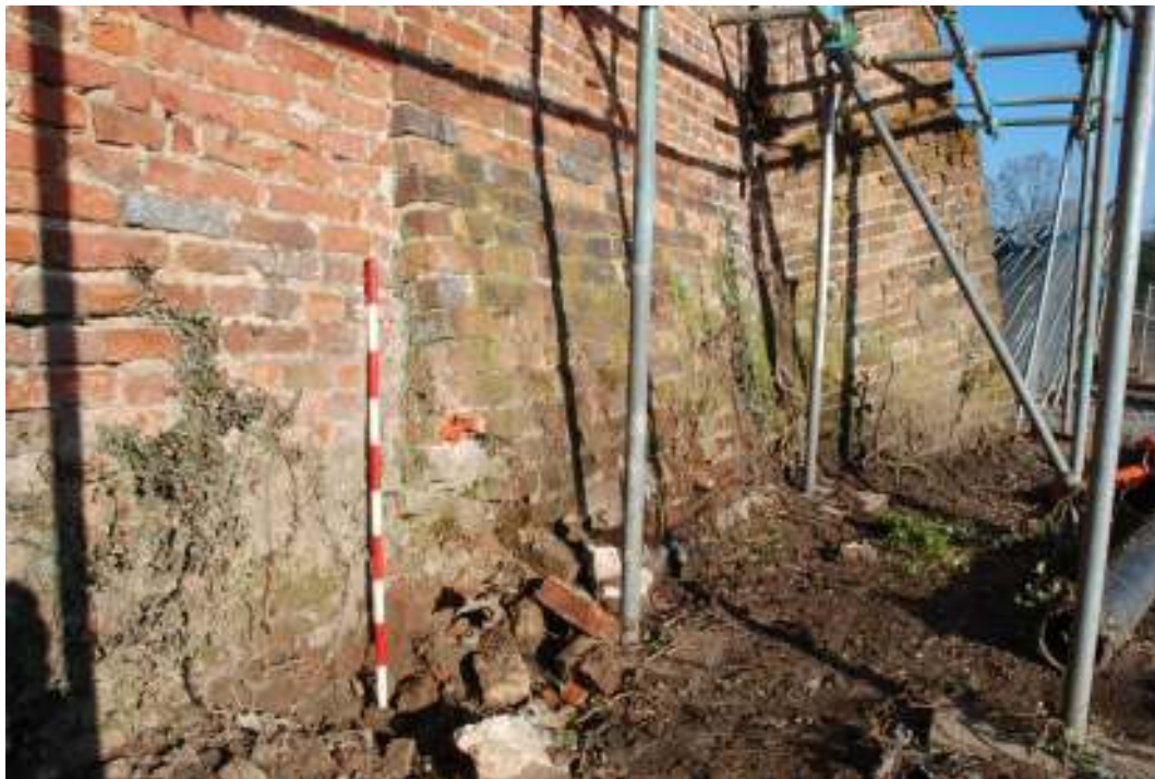
Fig. 128: Photograph of the southern wall of the dovecote, clearly showing the area of ‘patching’ running up to the south-eastern buttress.
