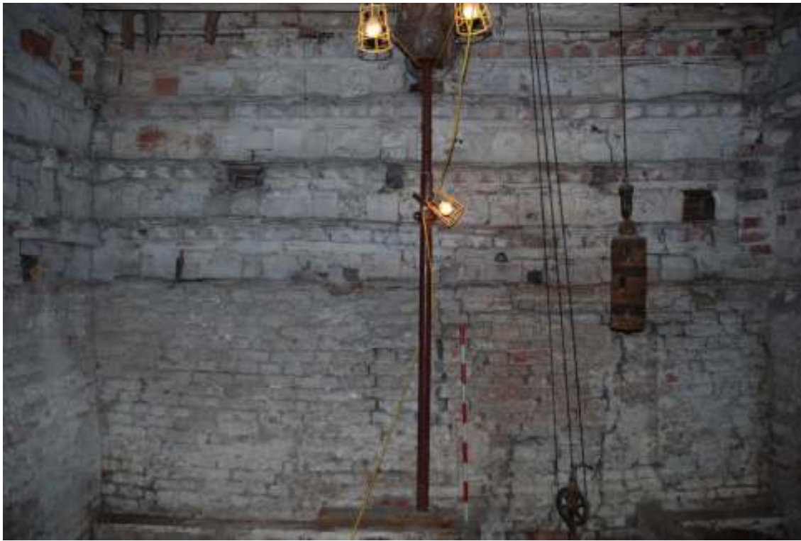
Fig. 24: Photograph of the interior northern wall of the dovecote – ground floor. Original build visible from c.100mm above the scale (battered re-facing below this). Rows of nesting-boxes are visible, although the holes themselves have almost all been blocked.
