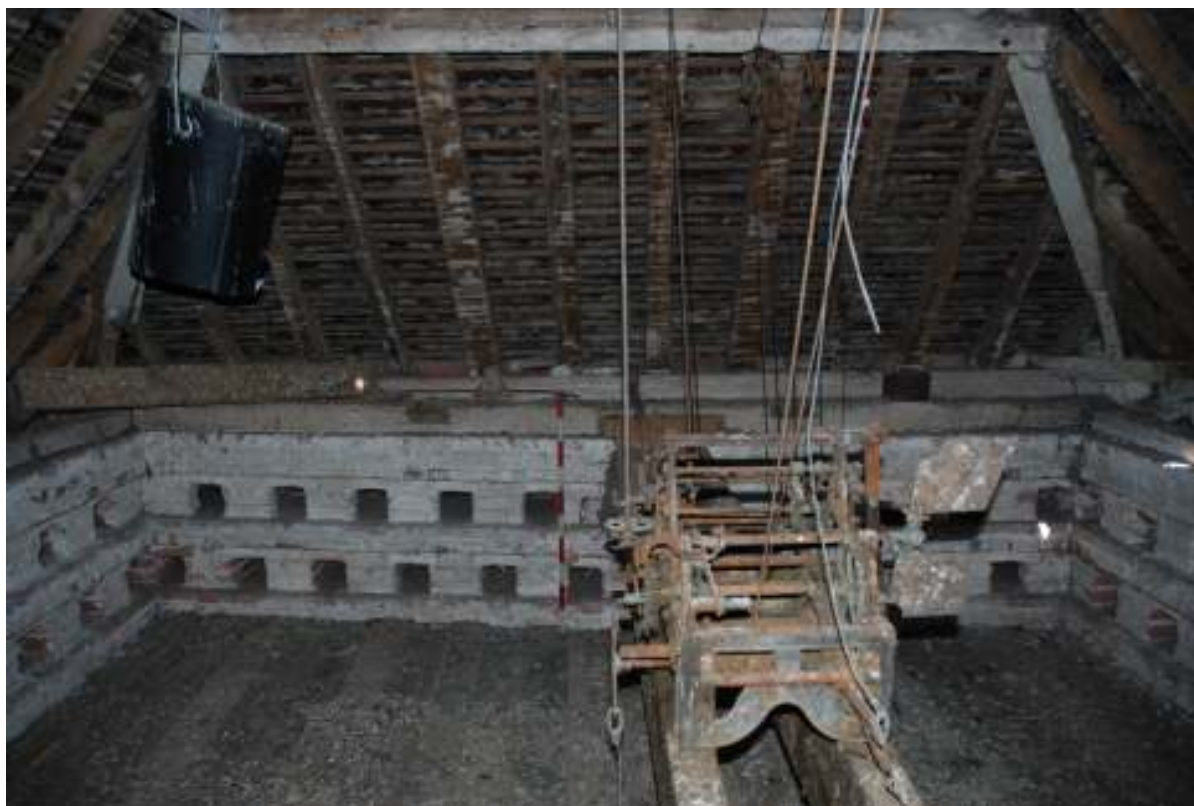
Fig. 58: Photograph of the interior northern wall – second floor. This is all part of the rebuild.
