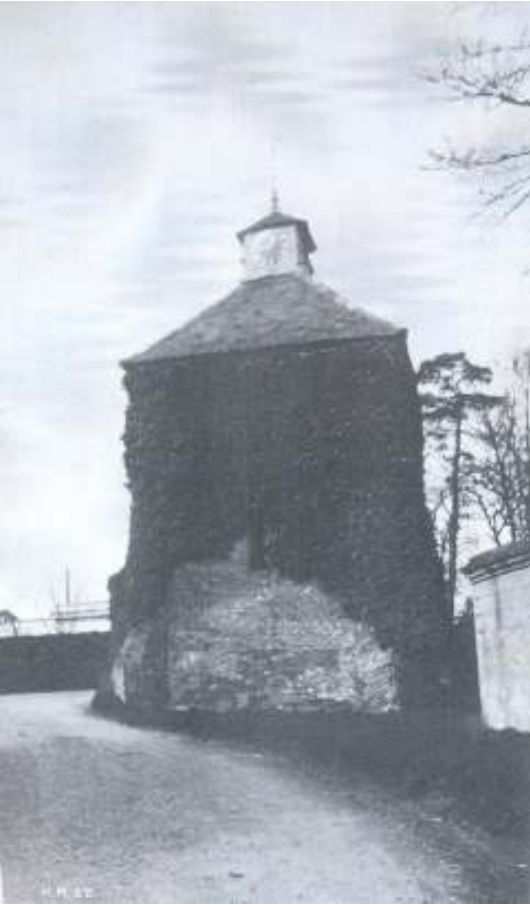
Fig. 8: 1923 photograph of the southern side of the dovecote, clearly showing the existing southern window; roof; cupola; and clock-face.
