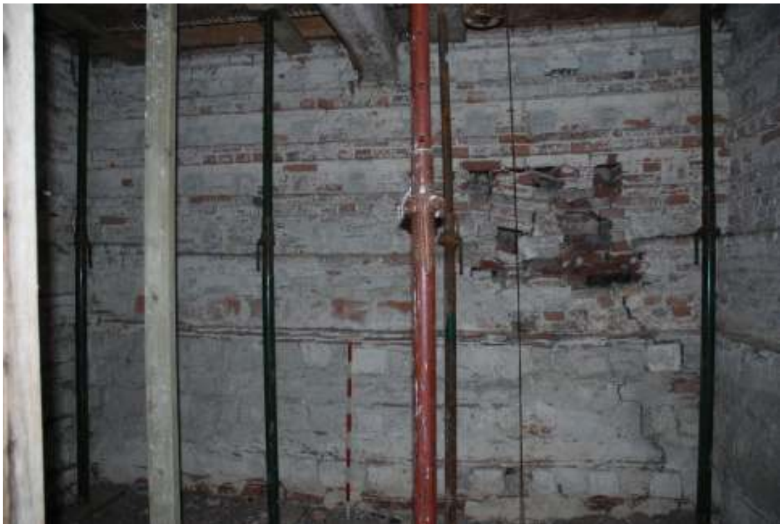
Fig. 25: Photograph of the interior northern wall of the dovecote – first floor. Original build up to c.200mm above the top of the scale, after which the nesting holes are distinctly different. A few unblocked holes are visible in the damaged area to the upper right of the photo.
