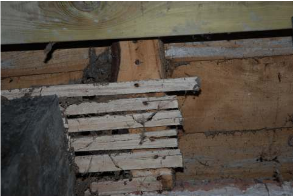
Fig. 112: Photograph showing some remaining patches of lath-and-plaster, on the first floor.
