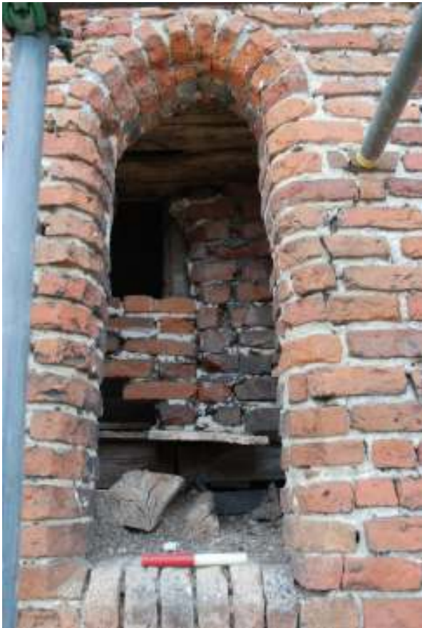
Fig. 32: Photograph of the window in the southern wall of the dovecote (from the outside). This shows its construction, including the Tudor arch with chamfered bricks.
