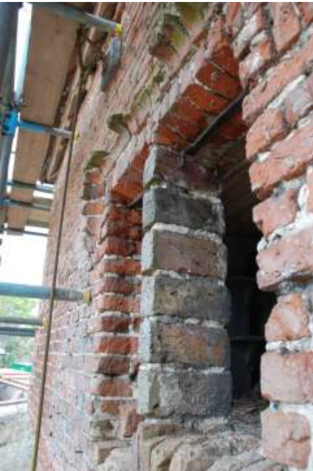
Fig. 76: Photograph of the window in the western wall (from the outside). This clearly shows the hood around the top of the window, the later mullion down the centre of it, and the chamfered bricks surrounding the window.
