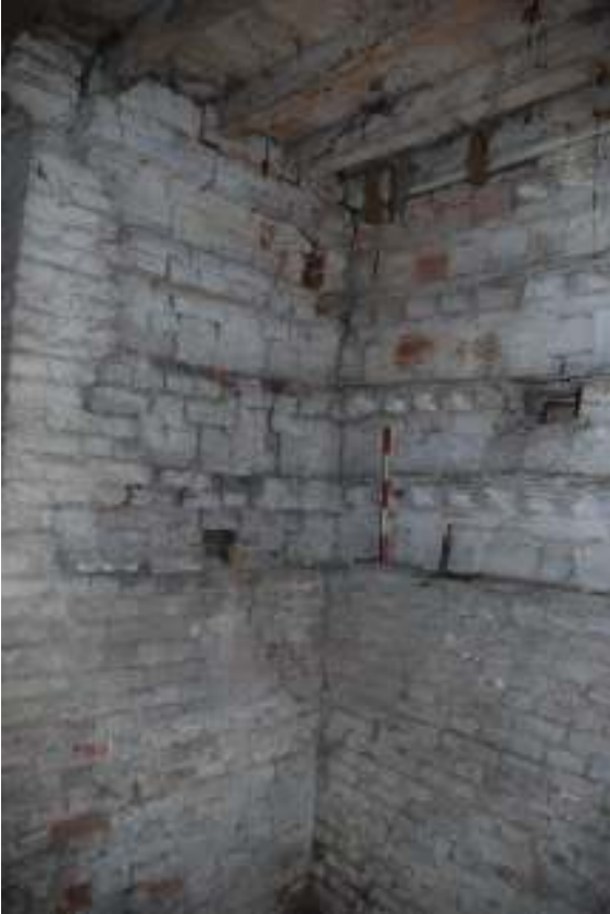
Fig. 74: Photograph of the north-west corner of the dovecote (ground floor). This shows how the northern wall is butted up against the western wall.
