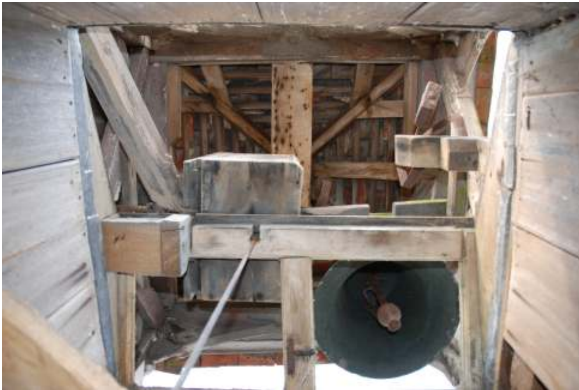
Fig. 141: Photograph up into the cupola. The striking hammer can be seen in the top right of the frame.
