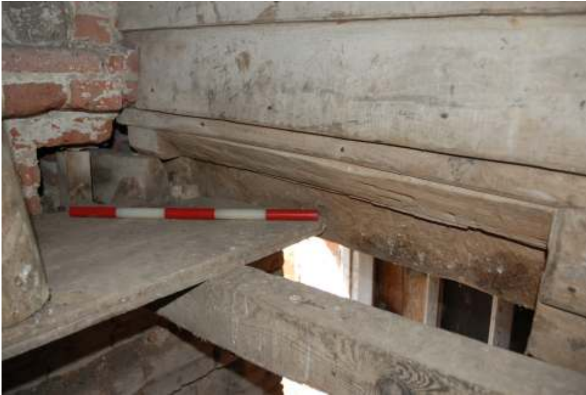
Fig. 109: Photograph showing the 'cut away' beam at the northern base of the chamber, where the earlier ladder up from the ground floor would presumably have stood.
