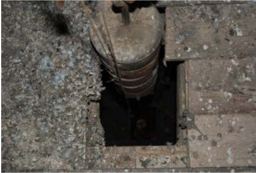
Fig. 146: Photograph of the chiming train weight, hanging down through the first-floor.
