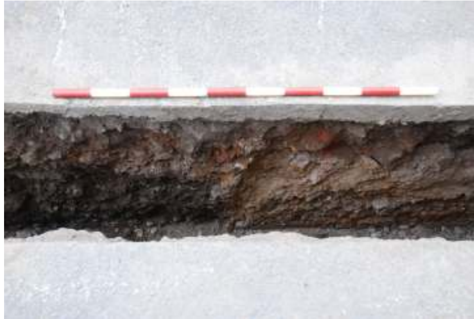
Fig.18: East facing section of Trench 6 showing made ground deposits to the right of the frame and construction cut and backfill for the underground rail tunnel to the left
