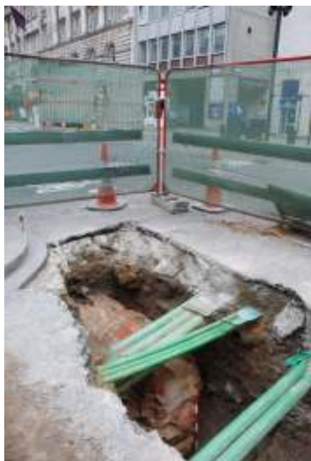
Fig.13: Trench in southern carriageway of junction with London Wall and Moorgate, facing NE
