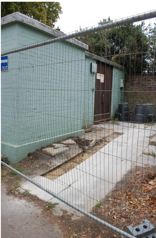
Fig 12 Total impact of groundworks at the Herbarium, representing surface clearance at the southern end and cutting of the adjacent paving slabs.
