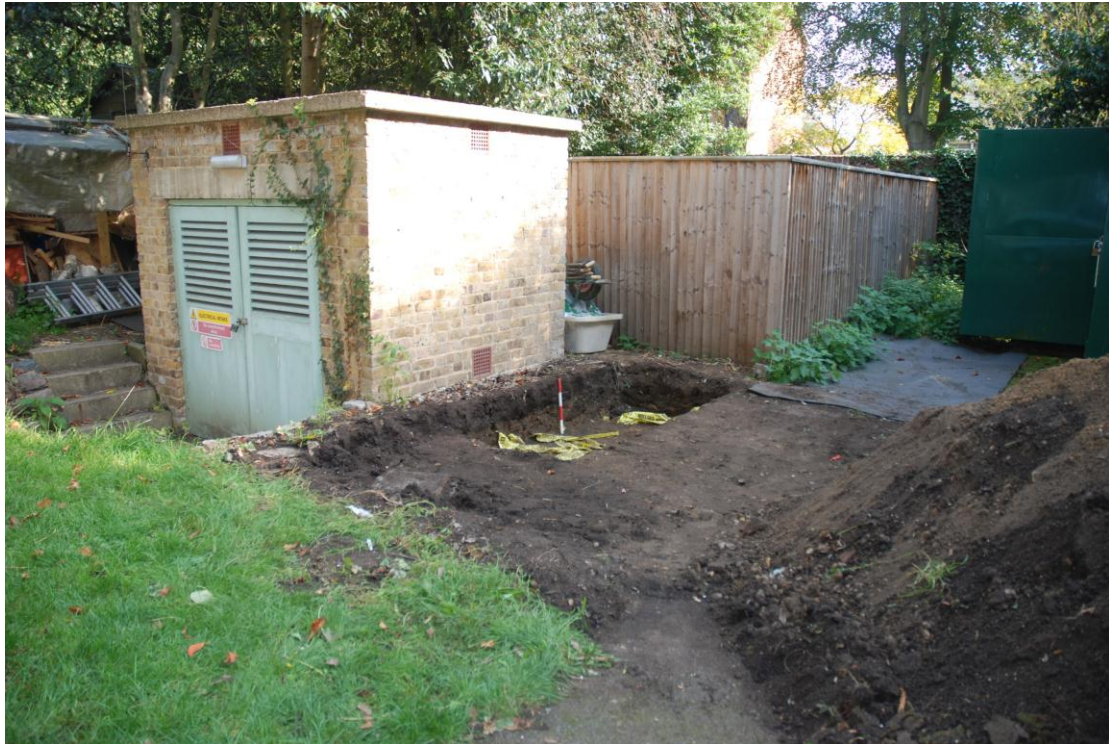
Fig 18 Location of the VO unit at the MNG Switch Chamber (after excavation).
