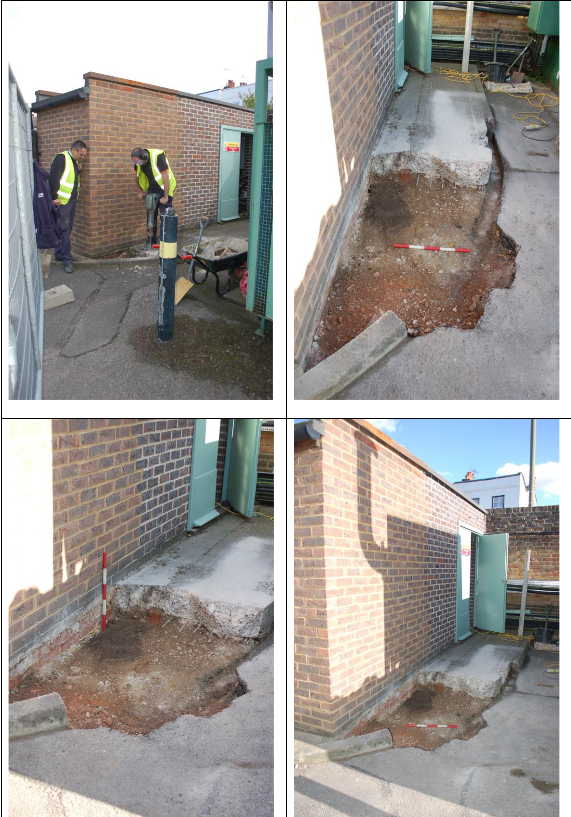
Fig 14 General images of the Jodrell Laboratory VO Unit under excavation. Top left: removal of the concrete slab to the required concrete foundation depth. Top right and below: after concrete removal to required depth the underlying deposits were also revealed to be tarmac and concrete, therefore, no impact on possible buried archaeological deposits.
