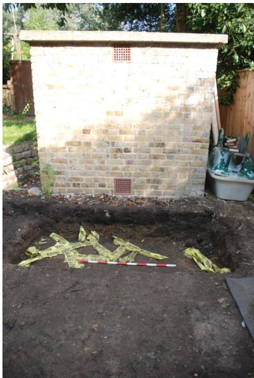
Fig 21 After ground reduction for the VO Unit. Excavation depth in the area was a maximum of 420mm on the northern side of the trench and 300mm on the eastern side. The works did not penetrate the overlying recent topsoil in this area and at the base of the trench a series of modern electrical cable runs were noted. At this location also, the groundworks only represent surface clearance and any archaeological deposits are not affected by these works.
