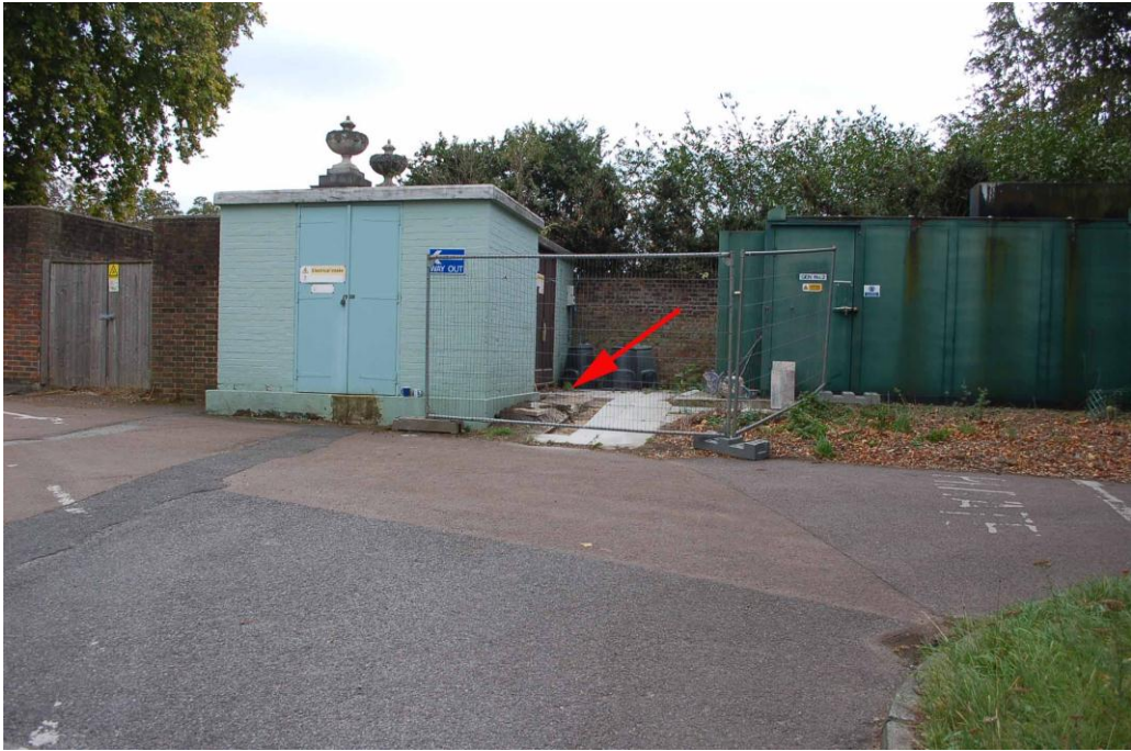
Fig 9 Location of the VO unit at the Herbarium Switch Chamber.
