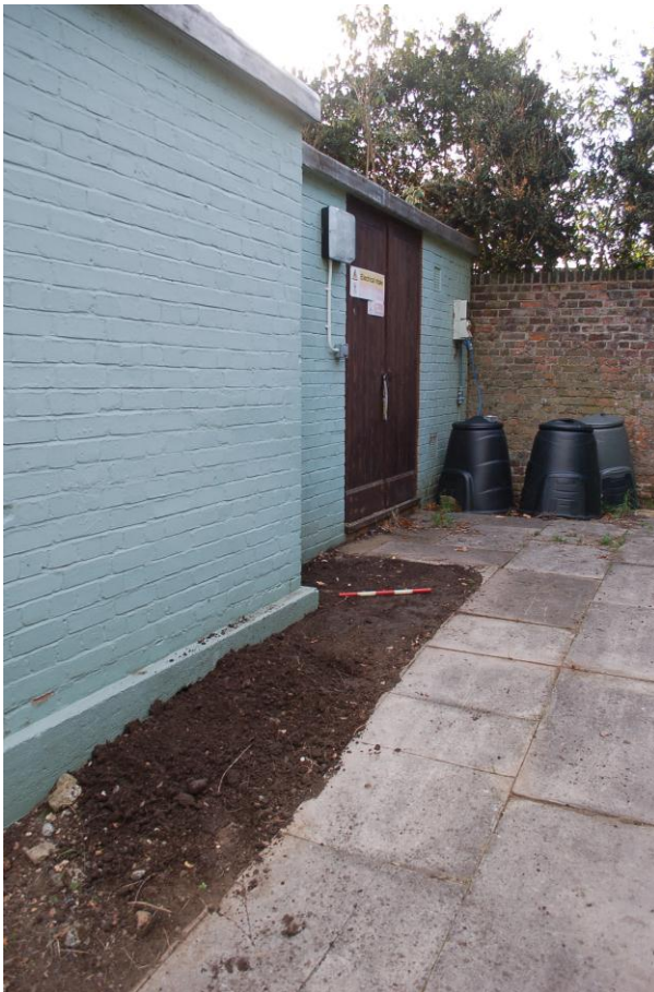
Fig 10 After completion of ground reduction of 25mm in depth at the southern end (near the scale 0.5m).
