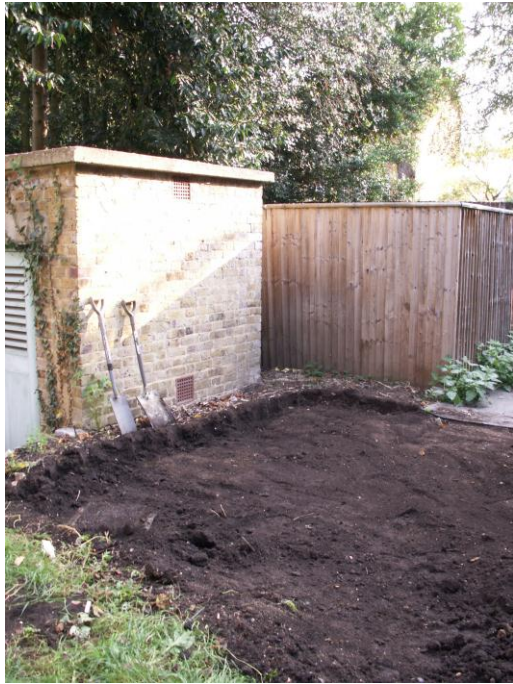
Fig 20 Clearance of mounded soil and compost in the area of the new VO chamber.
