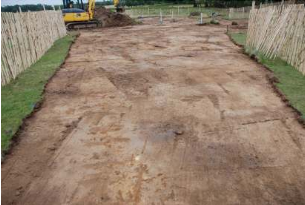
Fig.11: Topsoil strip of Lower Pen ponds area taken from westernmost tip facing ESE
