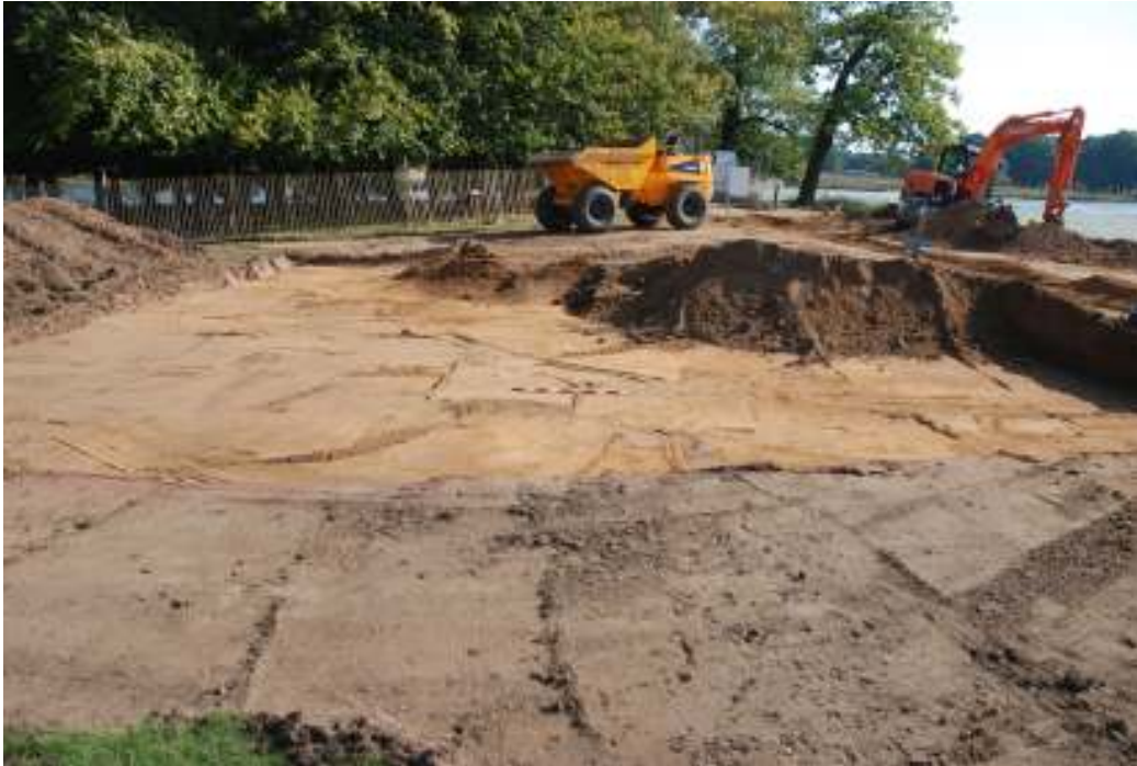
Fig.25: Reduced dig on grassed area, north of path by Pen Pond. Facing E
