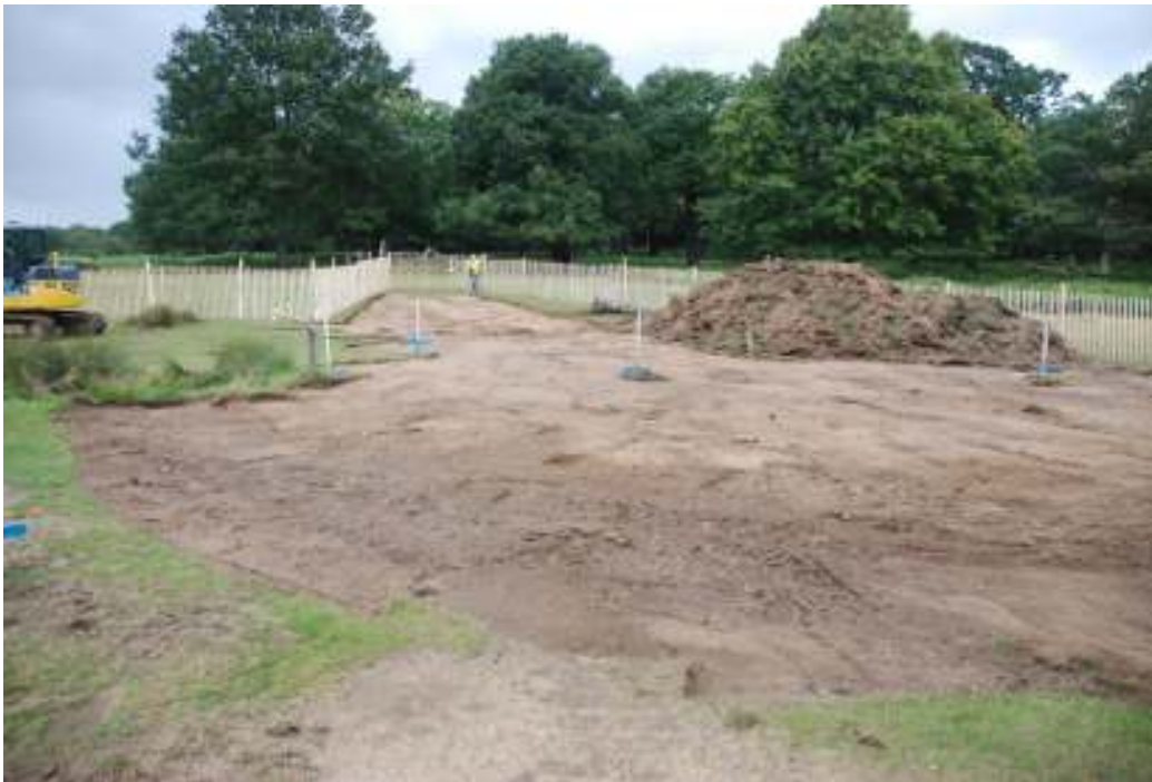
Fig.10: Topsoil strip of central area, made-ground in foreground forming base of existing gravel path
