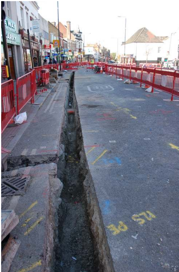
Fig. 17: Photograph of a further stretch of trenching along Plumstead High Street (trench 12), looking west.
