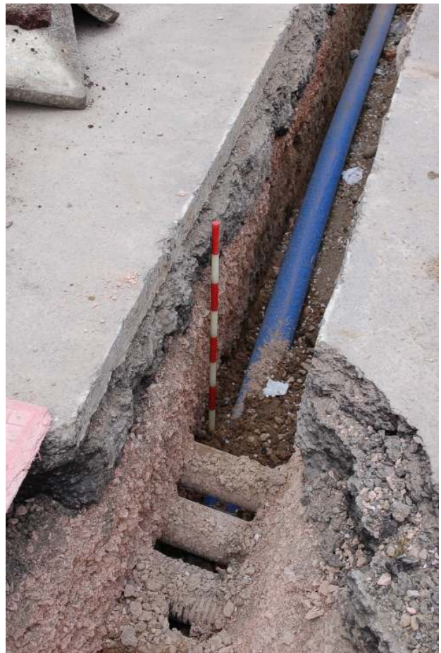
Fig. 16: Photograph of part of the trenching along Plumstead High Street (trench 10), showing the depths of modern MOT-Type 1 road make-up layers (the pink material).
