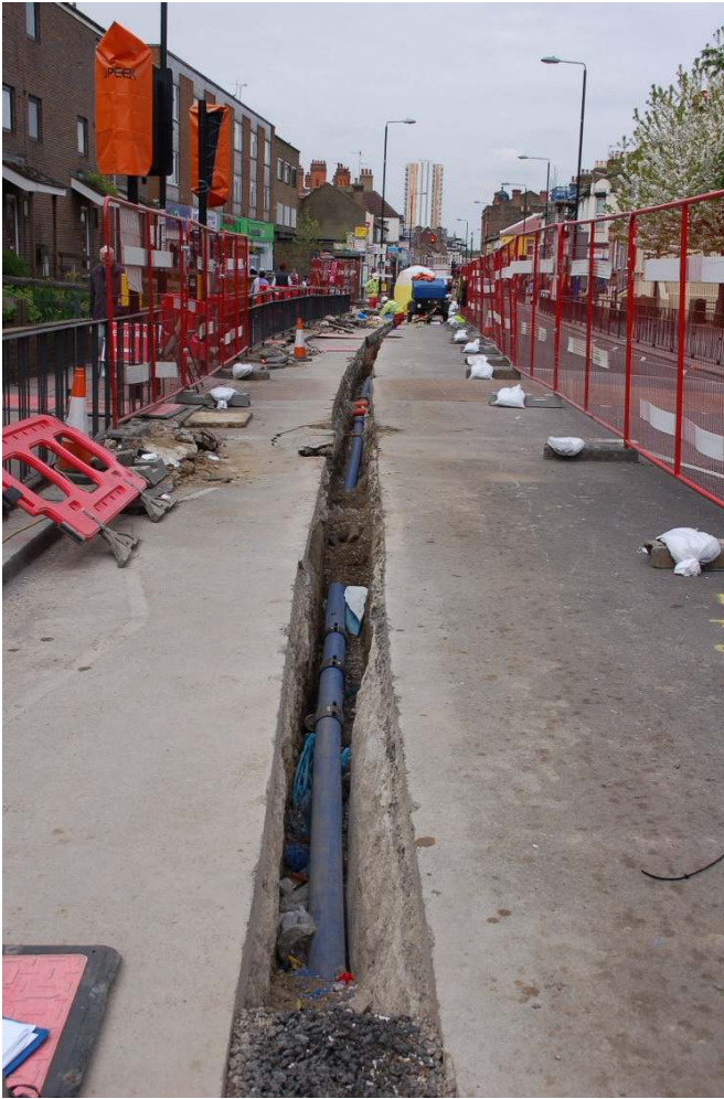
Fig. 15: Photograph of part of the trenching along Plumstead High Street (trench 10), looking west.
