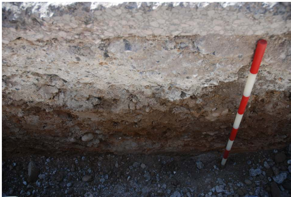
Fig. 18: Photograph of a section in the trenching along Plumstead High Street (trench 13), showing the modern road-surface overlying service backfill.
