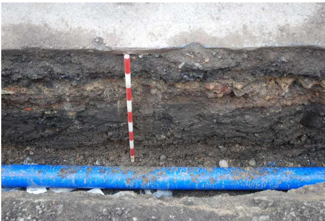
Fig. 12: Photograph of the section in the trench in Hartville Road (trench 1), clearly showing the modern road-surface overlying the black clay-silt deposit and silty gravels towards the base of the trench.
