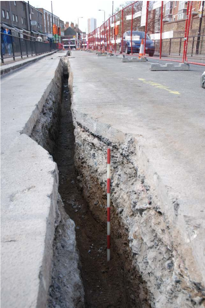
Fig. 14: Photograph of part of the trenching along Plumstead High Street (trench 9), looking west, showing a huge depth of modern road-surface / concrete, overlying sandy-silt and gravels.
