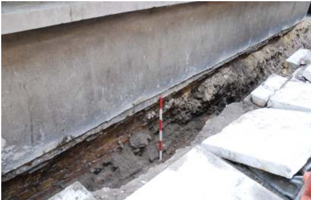
Fig.58: Graveyard Wall footings exposed on St. Peter's Alley, 21 st September 2010. View to South-east
