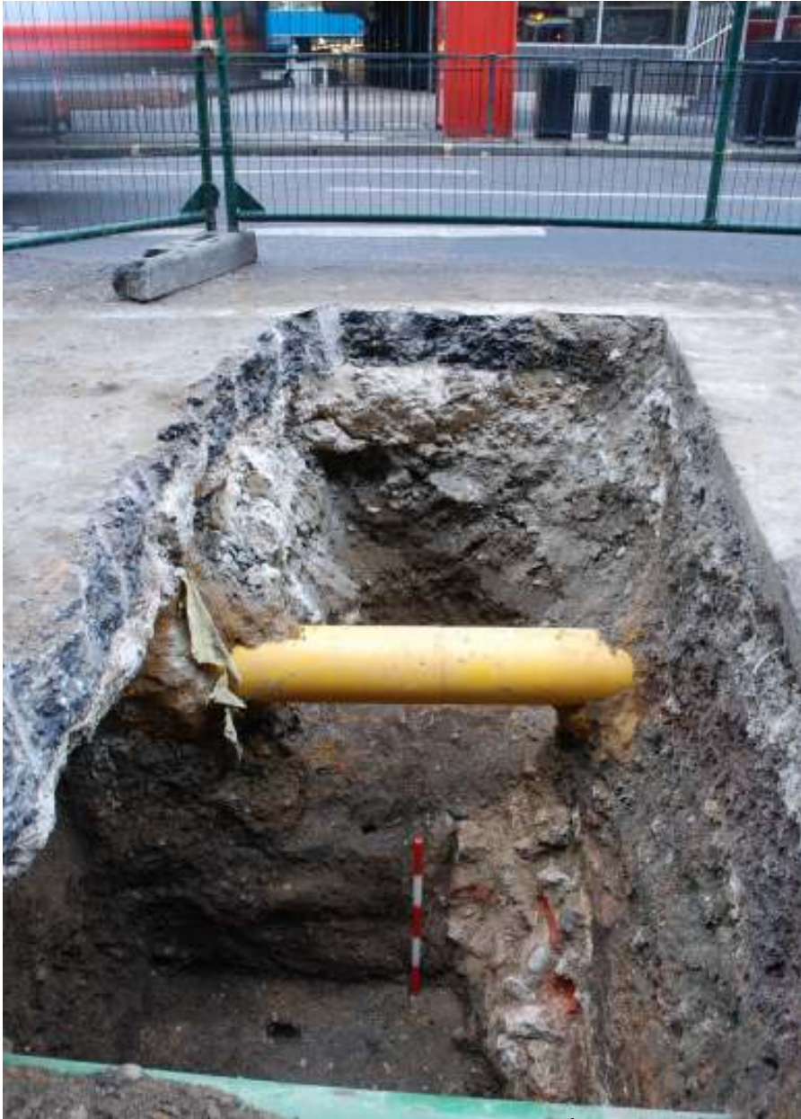
Fig.29: Masonry exposed in Aldgate High Street 14 th December 2010, note facing by 0.5m scale and rubble core extending into section, facing N
