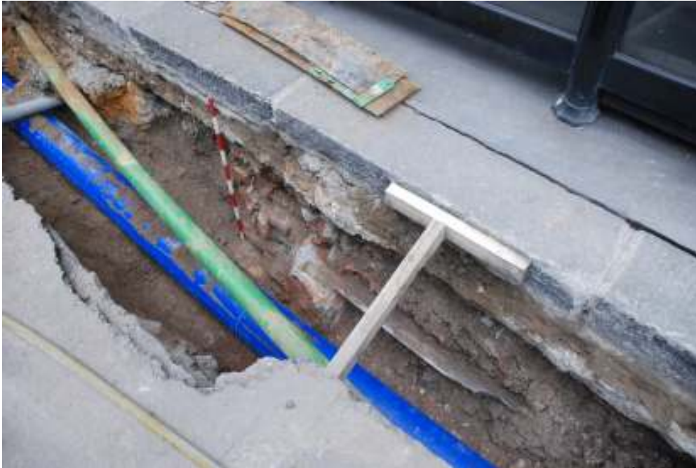
Fig.44: Concrete sloping roofed cellar recorded on Leadenhall Street, 11 th October 2011, facing SSE
