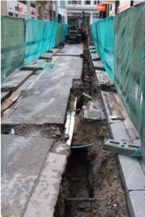
Fig.34: Cullum Street, 22 nd June 2011, facing W. Shot illustrating the presence of numerous services
