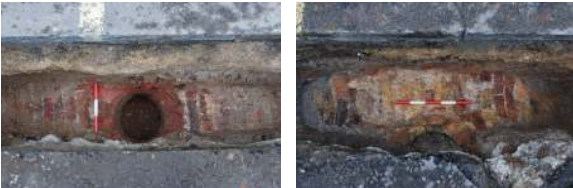
Fig.23: Brick-built coal cellars and their associated coal-chutes for filling. Overhead view from North side of trench
