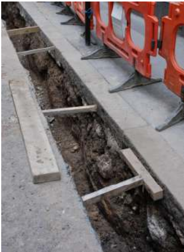
Fig.31: SE end of trench with exposed coal cellars to right of frame, 22 nd March 2011
