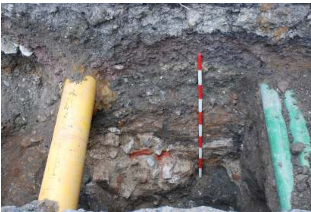
Fig.28: Masonry remains in trenching on Aldgate High Street, 14 th December 2010, facing E
