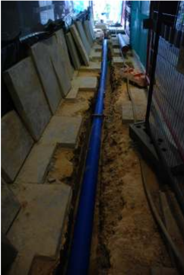
Fig.56: Pope's Head Alley, 14 th July 2011. Facing N, concrete in west section visible in right of frame
