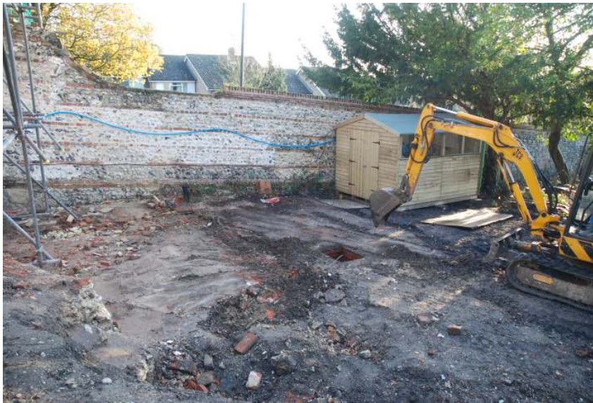
Fig 13 General view of the site strip works to the east of the Lodge building, looking southeast and showing a level concrete terrace appearing.
