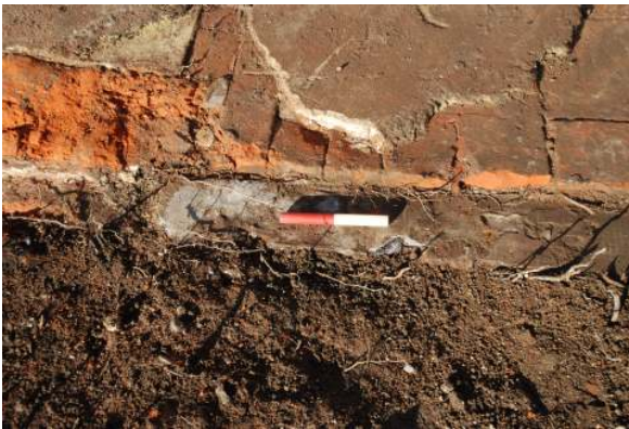
Fig 19 Detail of the slate damp proof course on the exterior face of the apsidal ended wall.
