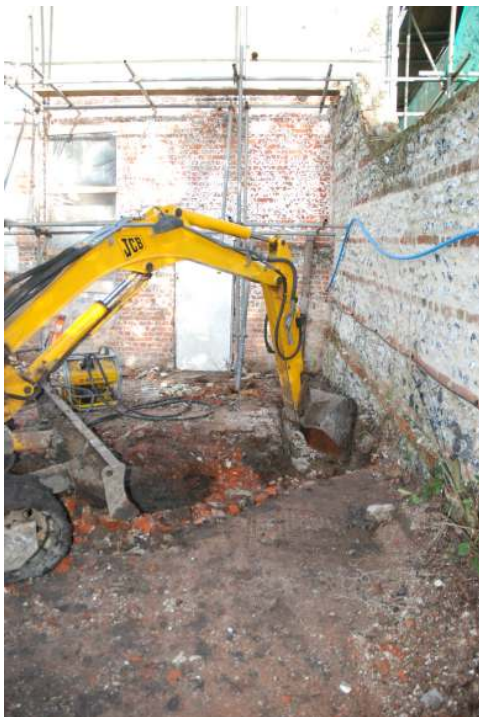
Fig 27 Excavation of footing Trench 2 adjacent to the lodge and the high garden wall site boundary, looking north ( cf. Fig 11).
