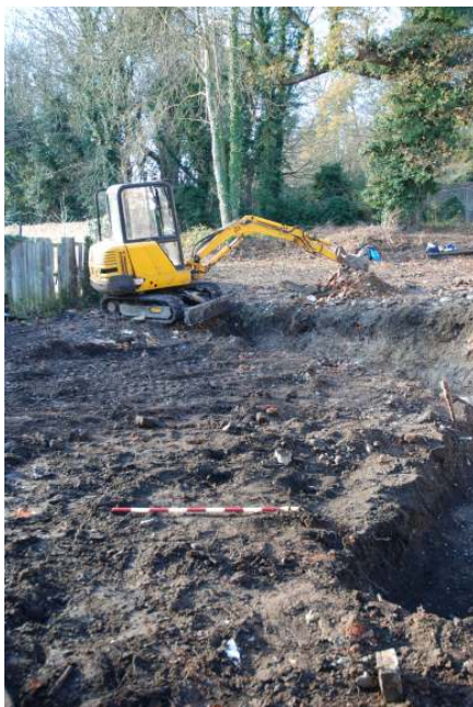
Fig 22 General view of the excavation of the northernmost east to west running footing, Trench 1, looking NNE ( cf. Fig 11)
