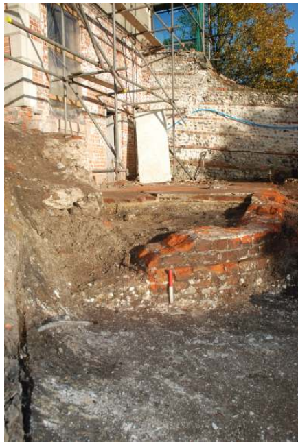
Fig 23 Excavation of footing Trench 1, looking east, with Trench 3 visible to the south (right). At the eastern end of Trench in the area adjacent to the 20cm scale the top of the natural chalk is at approximately +88.1m OD. This is 1.9m below the general level of the site at the entrance near the lodge and 1.2m below the level of the elevated garden area to the left of the image. This significant drop in height shows the comparative levels of the site either side of the garden wall, after the wall was removed. The wall can be seen running along the line of footing trench 2 and cutting the apsidal ended wall.
