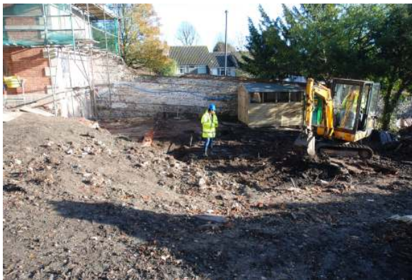
Fig 20 General view of watching brief soil strip works across the new build footprint, only made ground deposits were encountered in the footprint area beyond the brick and tile features of the terrace area adjacent to the lodge building.
