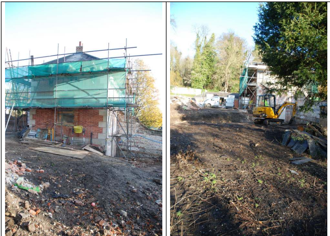
Fig 12 General views of 2 Lion Lodge and the general site area. Left: looking east, from the higher ground to the north. Modern made ground deposits were exposed across the site are to a general depth of circa 200mm to 500mm below current ground surface. No deeper soil strip was required for the redevelopment. The slope of the site can be seen to the right of the image. Right: general view of the soil strip works looking north.
