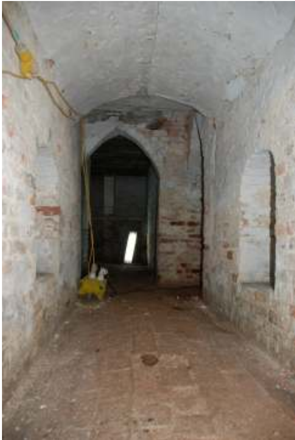
Fig. 103: Photograph of the small passageway to the west, looking towards the earliest part of the cellars. The line in the wall-build and roof construction can be seen towards the end of this passageway, reflecting the start of the extension.
