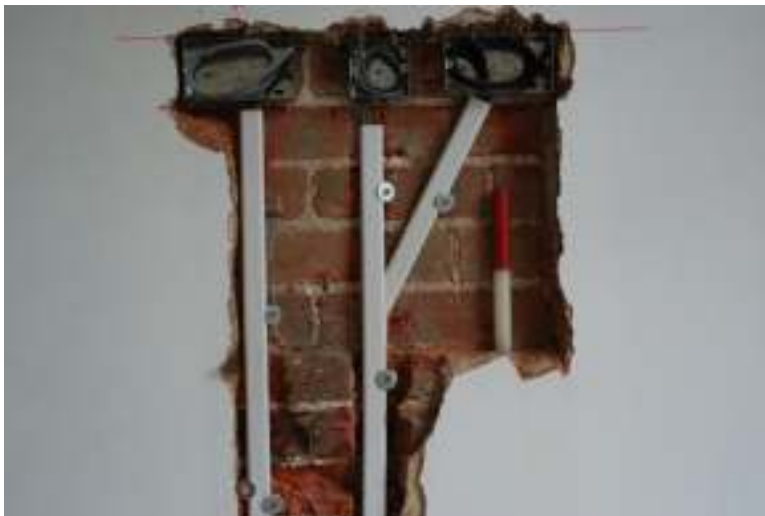
Fig. 58: Close-up photograph of the patch of the external earlier western wall, showing the step-in in the brickwork (the scale is resting on this).
