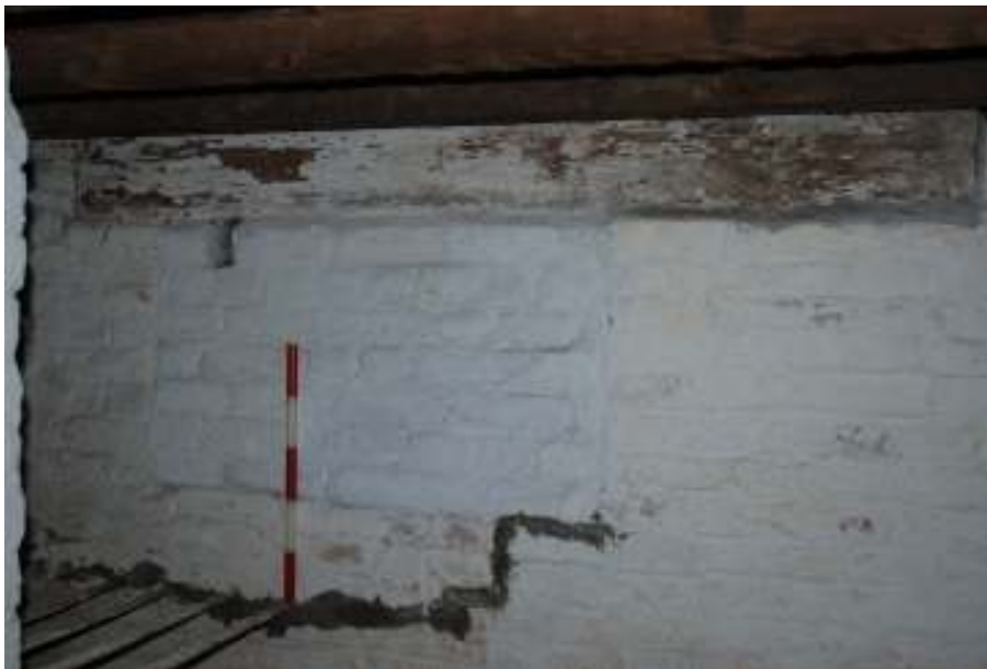
Fig. 96: Photograph of the blocked-up high window in the eastern wall of the southern-most room, and overlying timber lintel.
