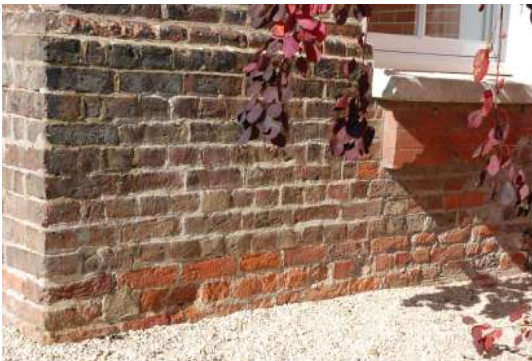
Fig. 27: Photograph of the lower three courses of brickwork on the southern part of the eastern wall. This is clearly red-brick, in English bond, and is therefore part of the original earlier 17 th Century house.
