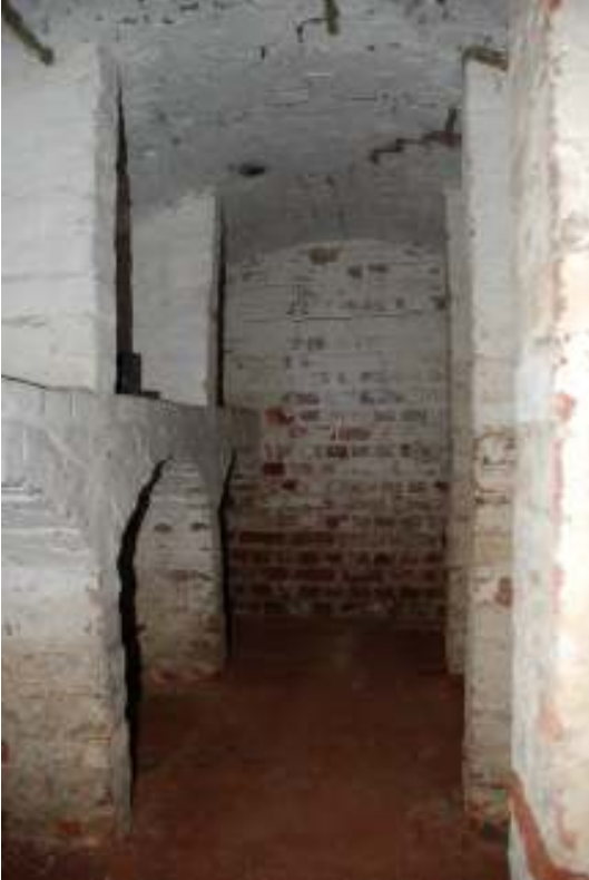
Fig. 111: Photograph of the first room on the right (on entering the cellar), with the bays / shelving that are original to this build on the left.
