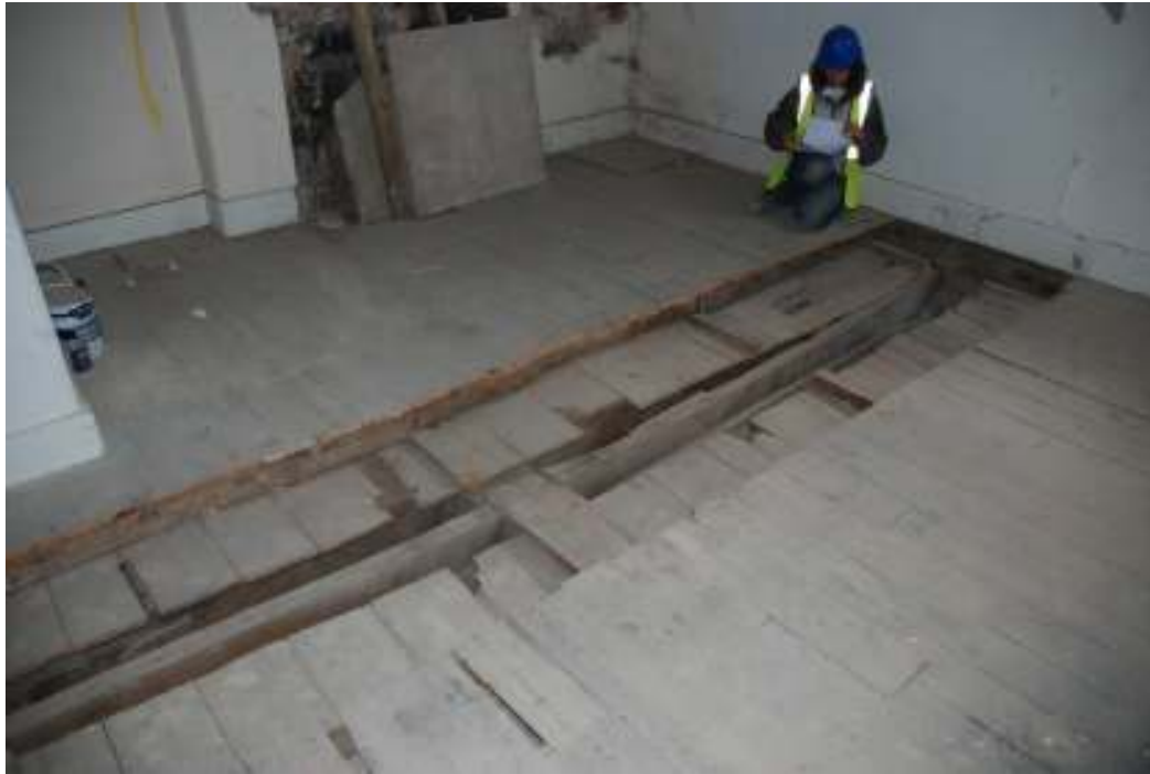
Fig. 129: Working shot of room S7 (southern side of house). This shows how the modern floor has been cut away to reveal the earlier timbers (including floorboards and an exposed joist in the centre), looking south-east.
