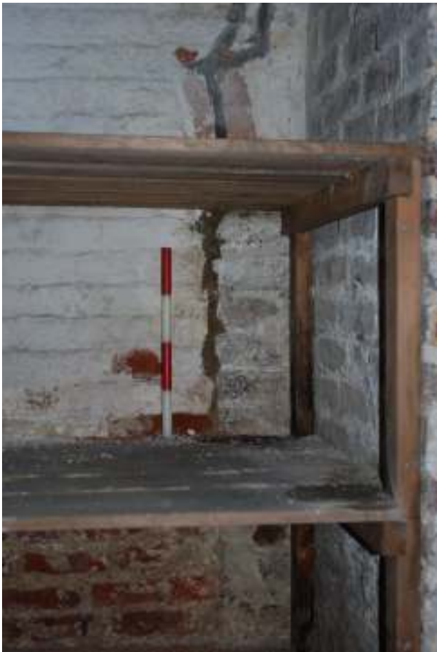
Fig. 93: Close-up photograph showing part of the blocked-up doorway, behind the brick partition / column. The brick arch is immediately above the uppermost shelf.
