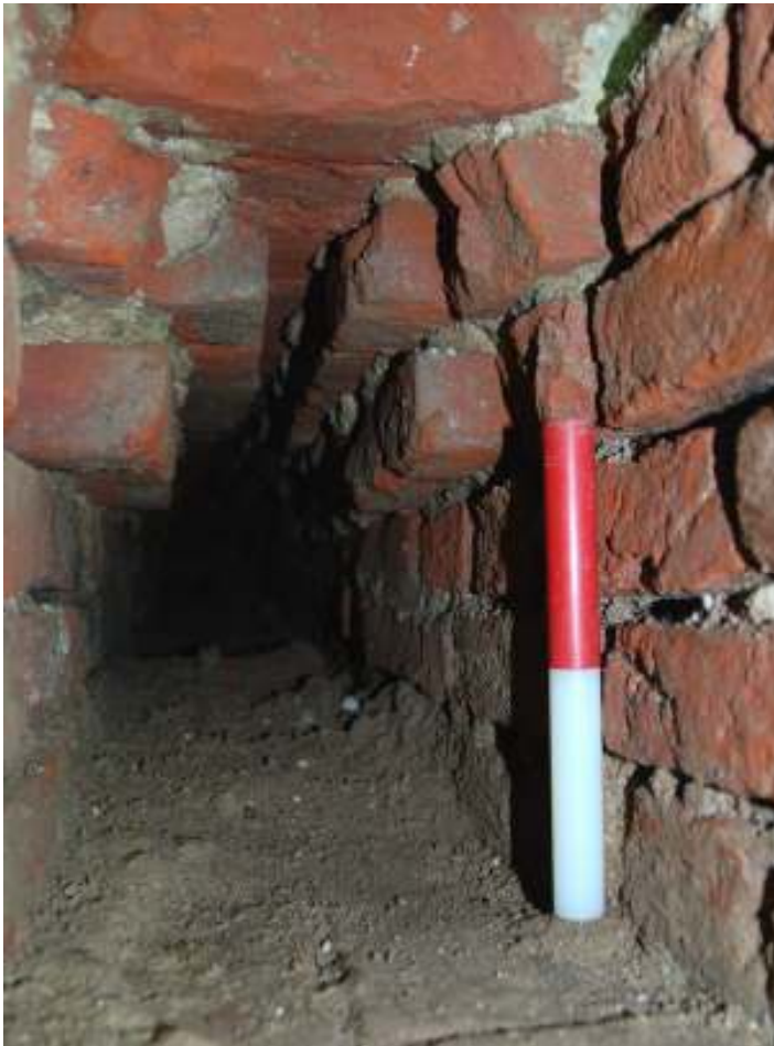
Fig. 40: Photograph of the interior of drain (101), showing its corbelled construction where it runs through wall (100).
