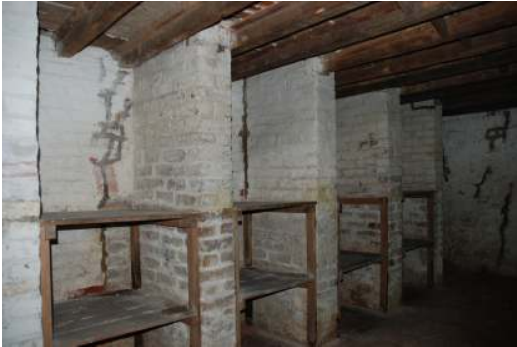
Fig. 92: Photograph of the southern wall of the earliest southern-most room of the cellar. The remains of a blocked-up doorway are visible in the foreground, on the wall behind one of the later brick columns / partitions.
