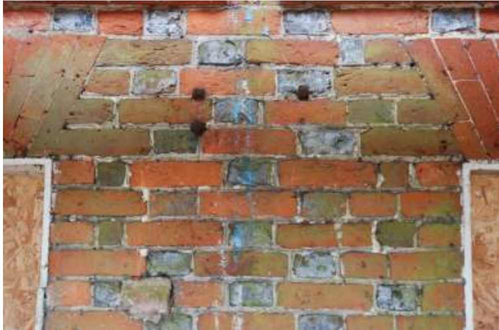
Fig. 20: Photograph of the checkerboard brickwork, included in the façade on the northern frontage.
