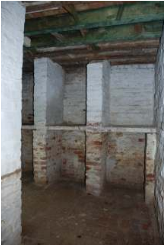
Fig. 116: Photograph of the brick bays / shelves in the central room of the cellar, taken from the entrance into this room.
