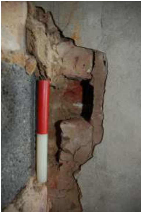
Fig. 54: Photograph showing the internal face of the earlier western wall, exposed in the 'secret' cupboard' in the dining room.
