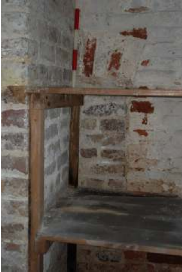
Fig. 94: Close-up photograph showing the western part of the blocked-up doorway, clearly showing the brick arch over the top of the door.
