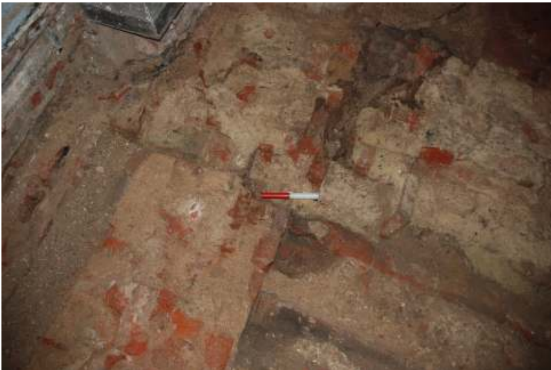
Fig. 47: Close-up photograph of wall (109) (bottom of the image) abutting wall (107) – clearly showing the different materials and mortars used.
