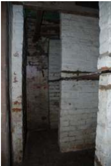
Fig. 115: Photograph of the brick bays / shelves in the small room in approximately the centre of the cellar.
