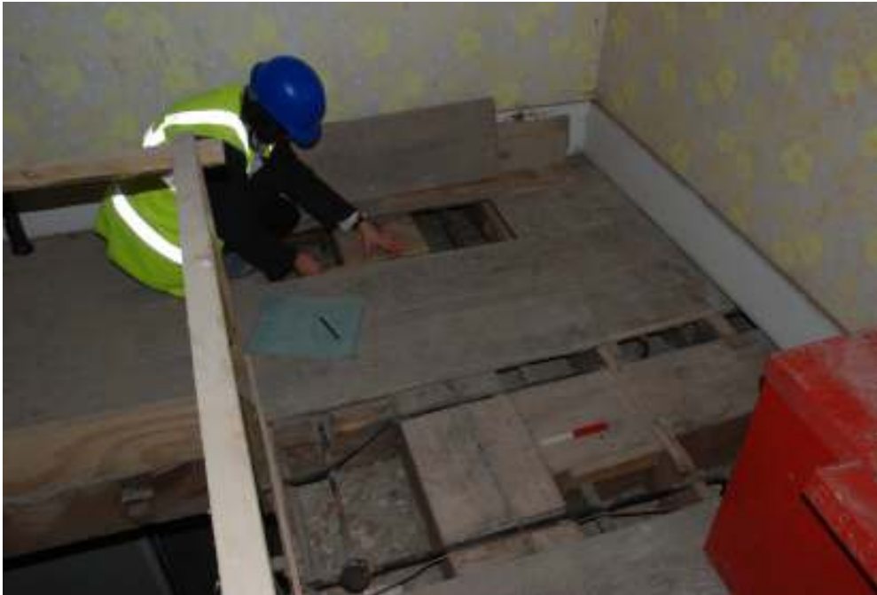
Fig. 142: Working shot showing the measuring of timbers in the south-west corner of room S21.
