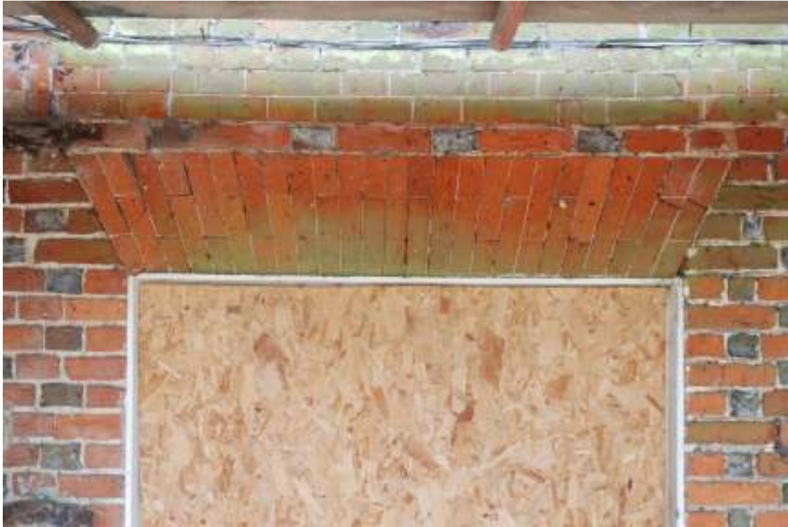
Fig. 21: Photograph of the gauged brickwork above the ground-floor windows in the façade on the northern frontage.
