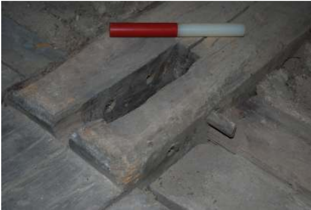
Fig. 136: Detail of above figure showing floorboards and pine skins either side of change in level of timber 2, plus mortise with one surviving peg. Facing south-east (0.2m scale).
