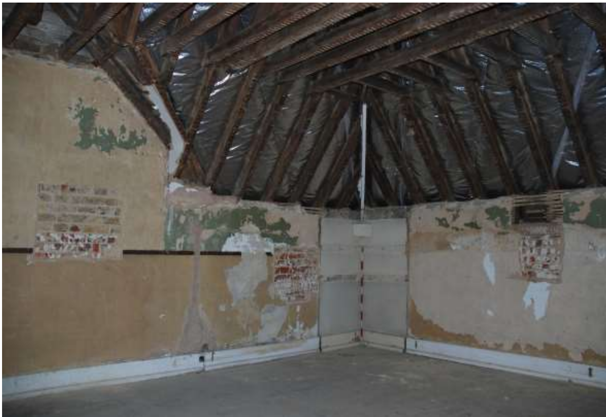
Fig. 95: General photograph of the upper engine room (S13), looking south-east. Areas of the original lime-washed brickwork can be seen beneath the later rendering.
