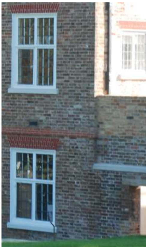
Fig. 55: Northern frontage, ground-floor wall. This appears to continue further to the west (beyond the western end of the house at the upper levels) with no break in construction, and suggests that the western rooms were constructed at the same time as the main house.
