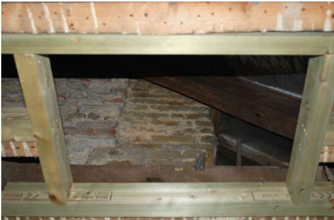
Fig. 247: Photograph, taken from S12, of the yellow stock-brick chimney, facilitating the fireplace in room F16, and possibly one in room F15 (later inserts). The chimney abuts the original red brick wall to the left (south).
