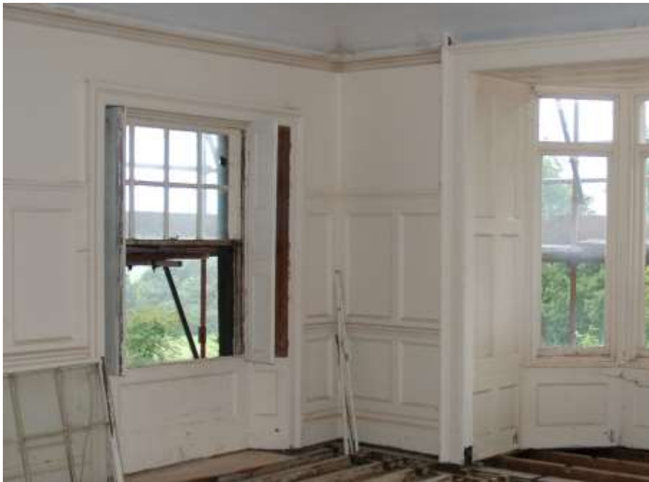
Fig. 218: Photograph of the new window (on left of the frame) in the Pink Bedroom (F5).
