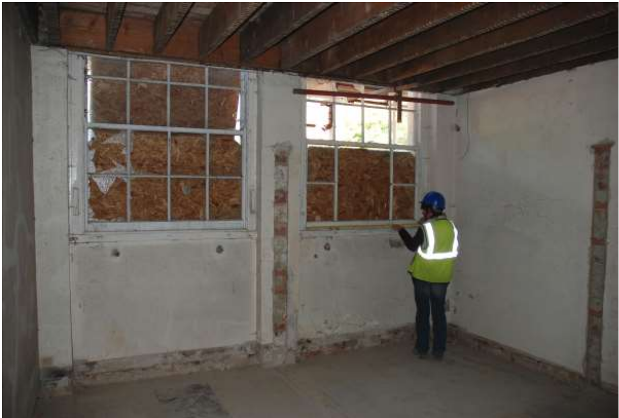
Fig. 97: Photograph of the large windows in the lower engine room. The top sections are obscured by the later floor insertion. The wall to the right is also a subsequent addition.
