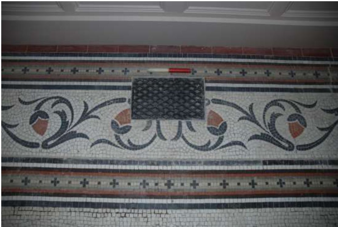
Fig. 157: Photograph depicting the heating grate set within the entrance hall mosaic floor.
