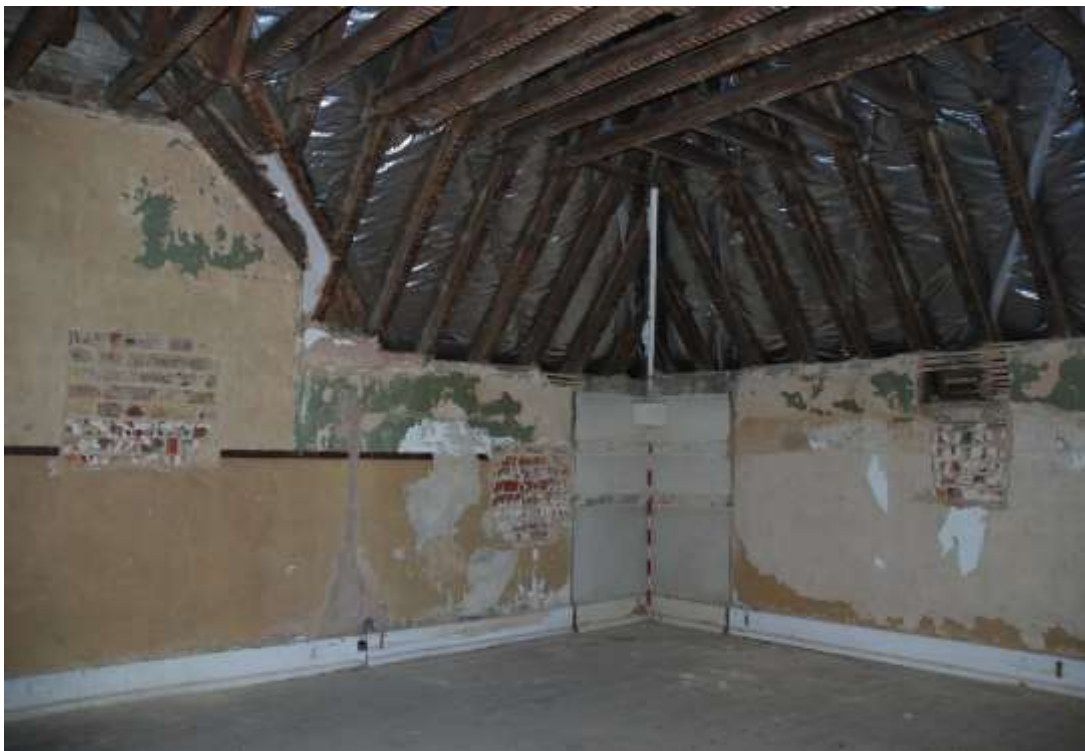
Fig. 245: Photograph of the upper engine room showing the later plastering / rendering of the wall, removed in three areas to show the underlying lime-washed brickwork.
