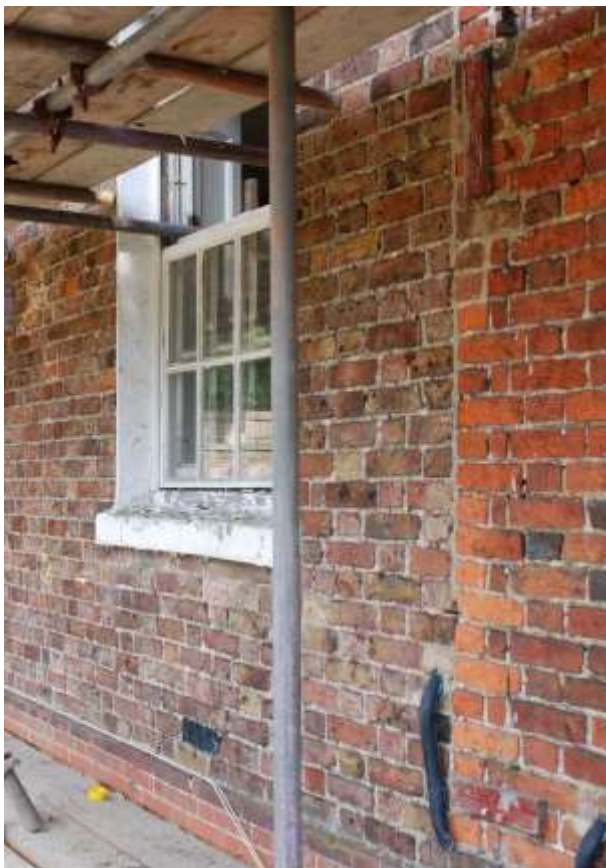
Fig. 31: Close-up view of the line between the red-brick of the 'earlier' house and the grey-brick of Partridge's extension (southern frontage).
