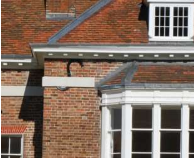
Fig. 170: The S-shaped tie rod, inserted at the same time as Captain Tarleton's eastern extension.
