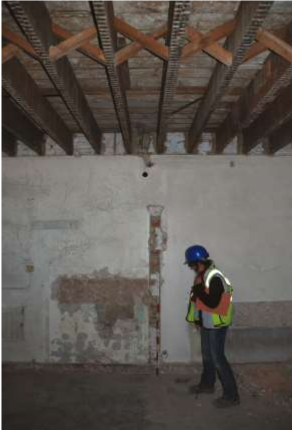
Fig. 246: Photograph of the lower engine room, showing the herringbone strutting of the roof.
