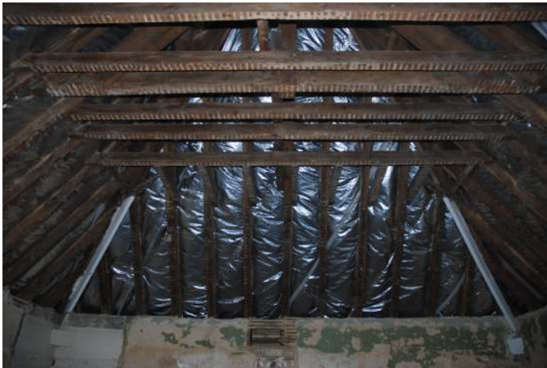
Fig. 104: General photograph of the roof of the engine room. The original level / base of the roof trusses was c.350mm below the top of the now-rendered walls.
