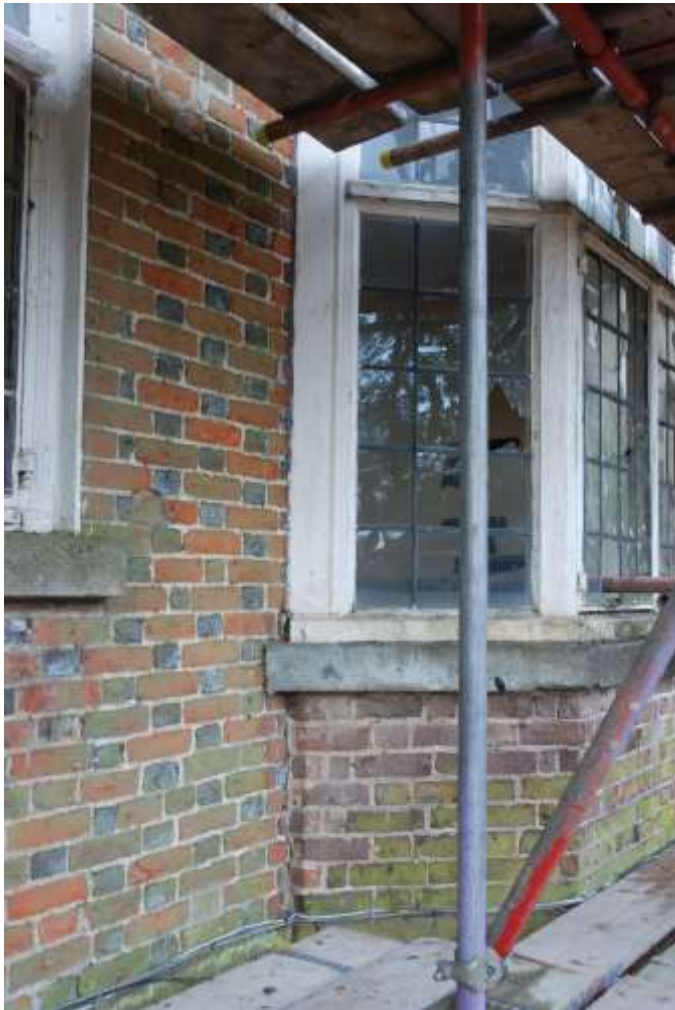
Fig. 39: The bay-window on the northern frontage, outside room F22. The brickwork of the bay window is built clearly abutting the earlier façade brickwork.
