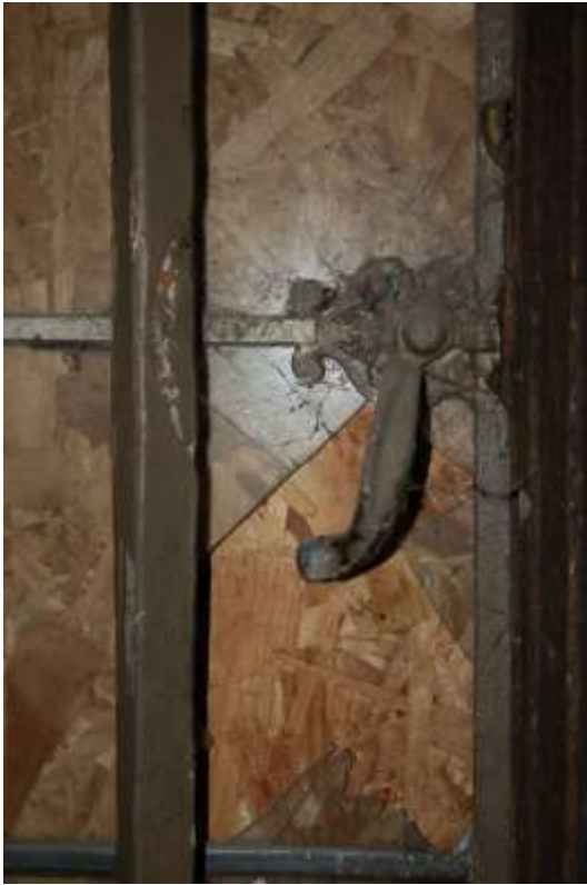
Fig. 35: Window catch on metal frame in the entrance hall (G22) – in the 'early' part of the house but clearly replaced during Partridge's rebuild.
