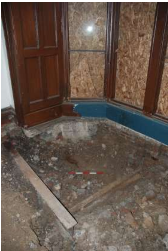
Fig. 252: Photograph of the RSJs and concrete under the library floor, to support the structure.
