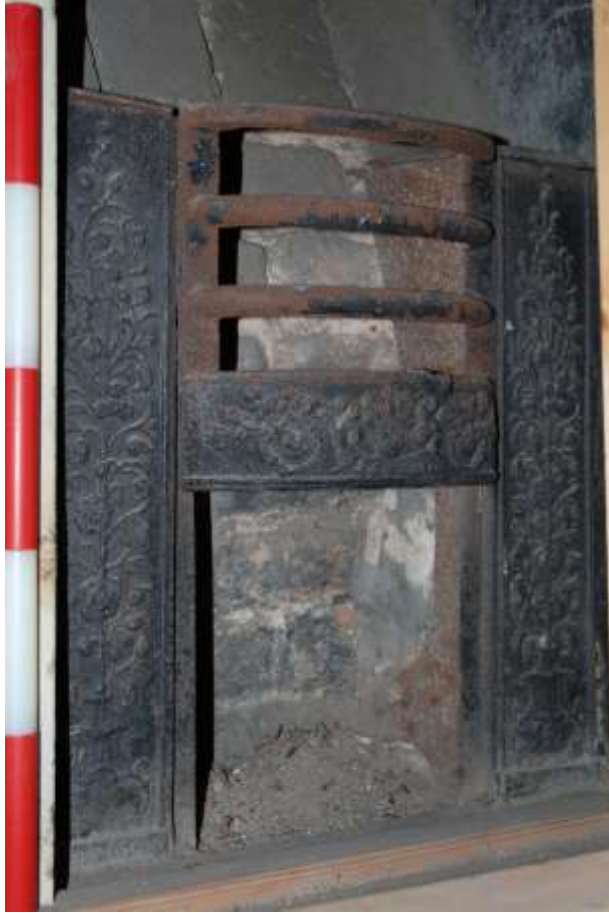
Fig. 82: Close-up view of fireplace in room S16. The central section is the same design as S12 (fig. 79), but with different side panels.
