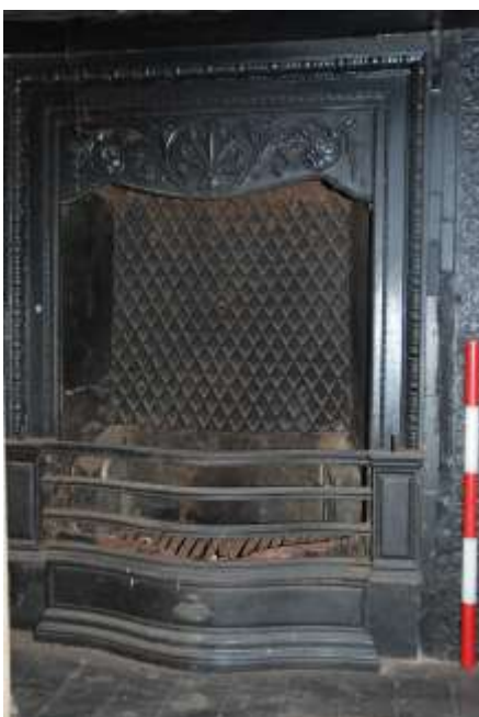
Fig. 178: Detail of the grate of the western fireplace in the Drawing Room.
