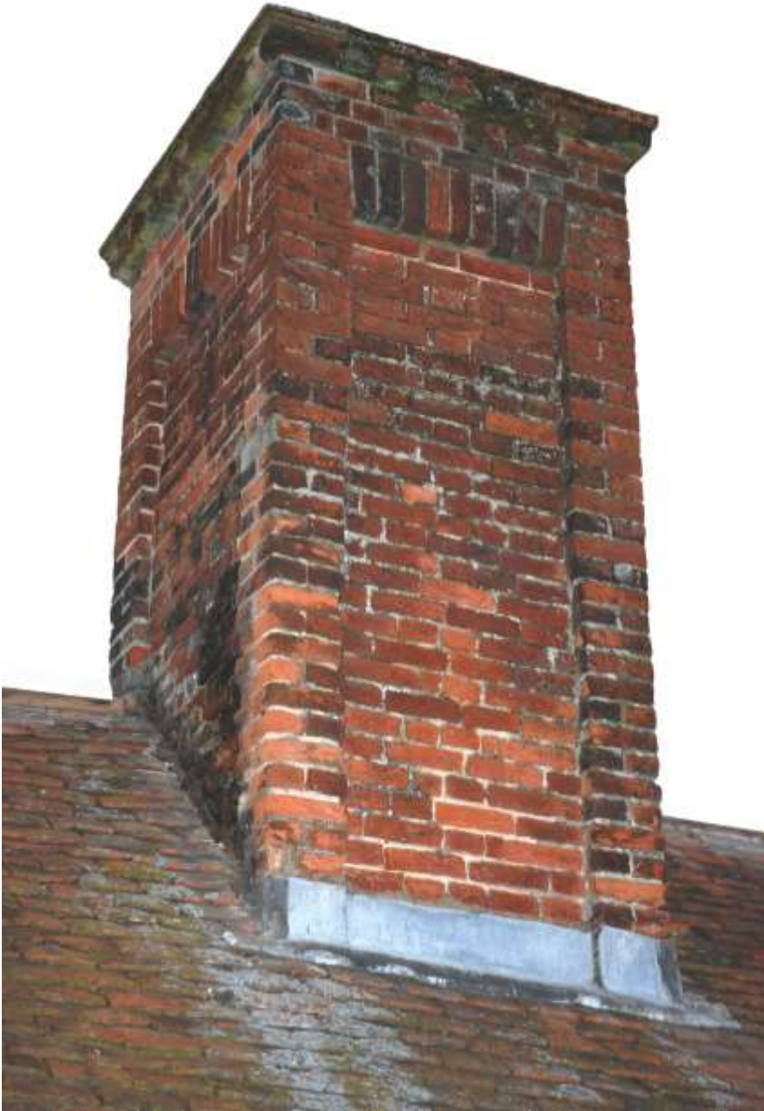
Fig. 259: Photograph of the chimney above the entrance hall and billiard room, with the upper courses clearly having been rebuilt during the 1924-25 repair works.
