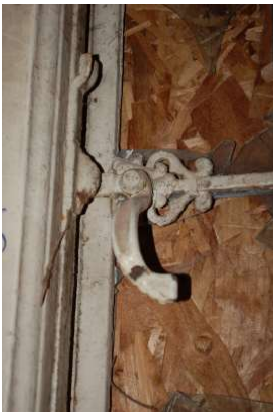
Fig. 36: Window catch in the kitchen (G19) – in the area of Partridge's rebuild.
