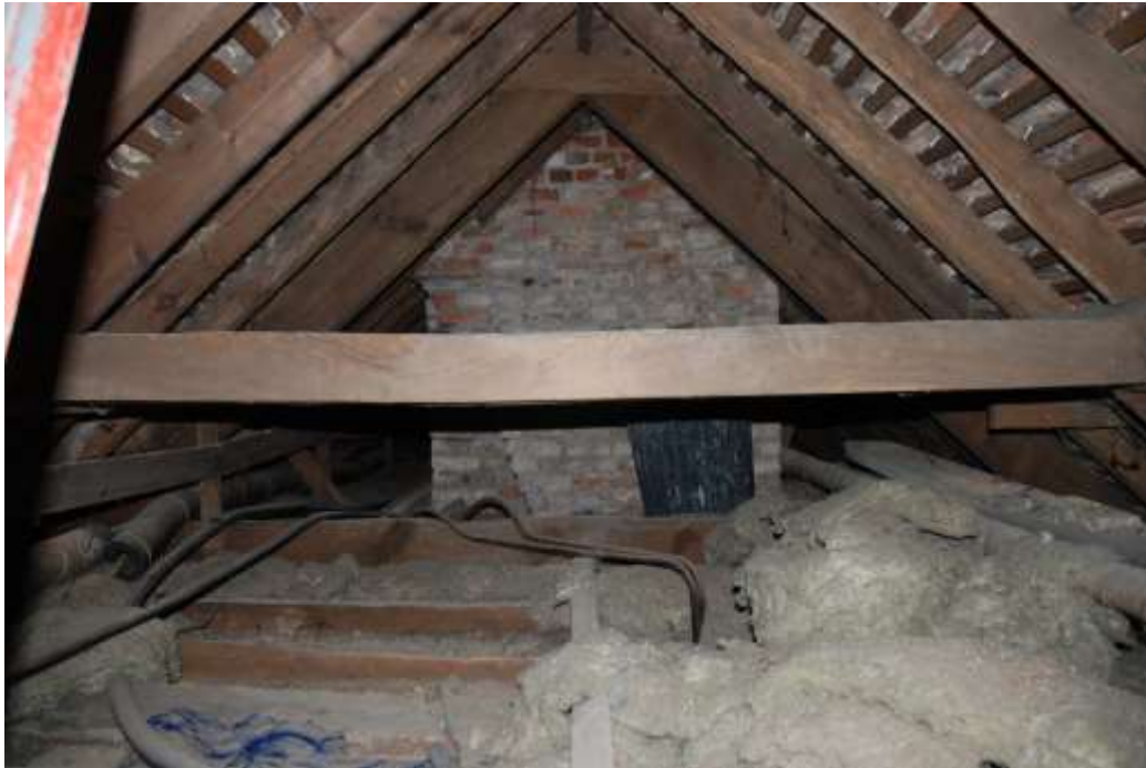
Fig. 43: Photograph of the roof-space, looking west from above room S18 (into the area of Partridge's extension).
