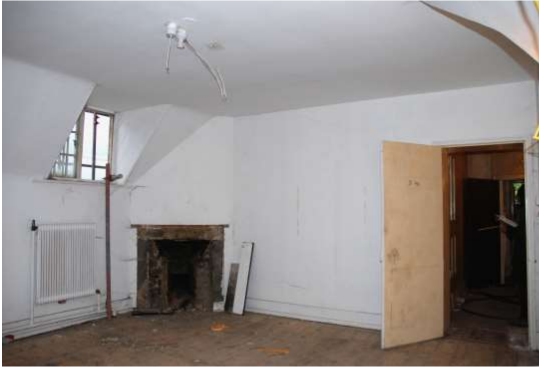
Fig. 244: Photograph of the upper engine room (S13), showing the inserted floors, fireplace, dormer window, and doorway.
