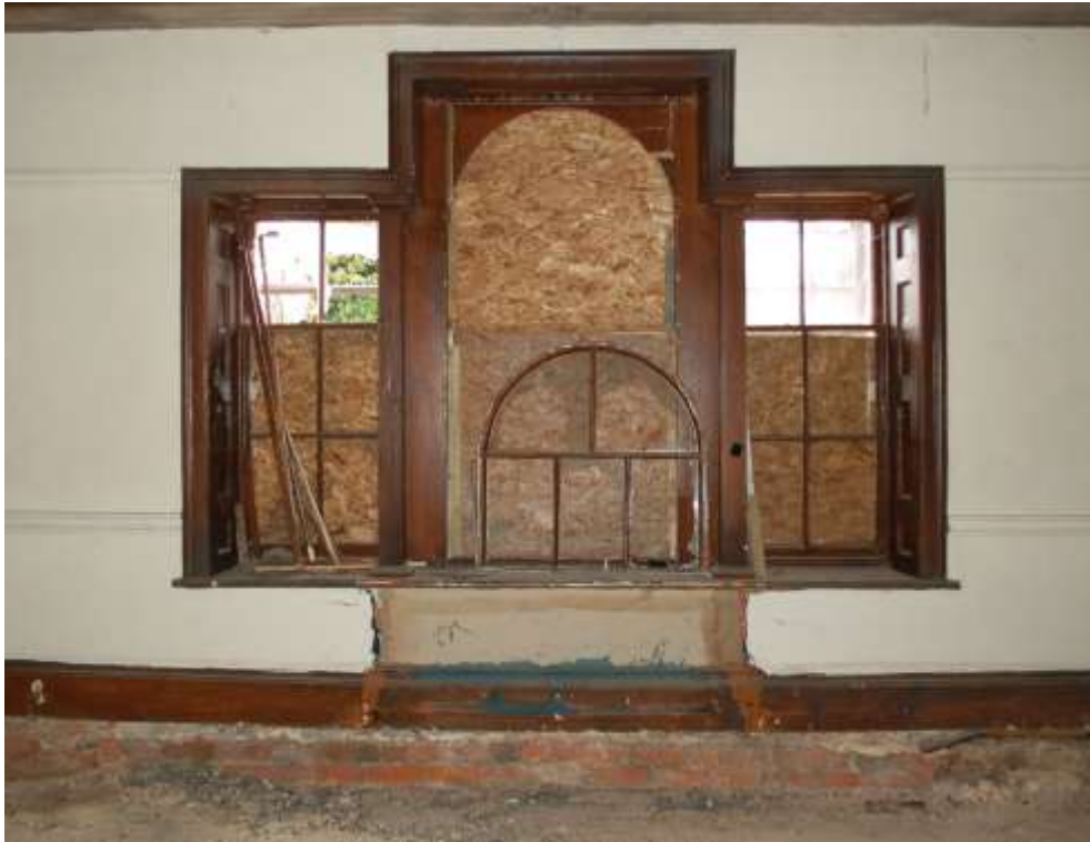
Fig. 253: Photograph of the brickwork underpinning the Venetian window – part of the 1924-25 repair works.
