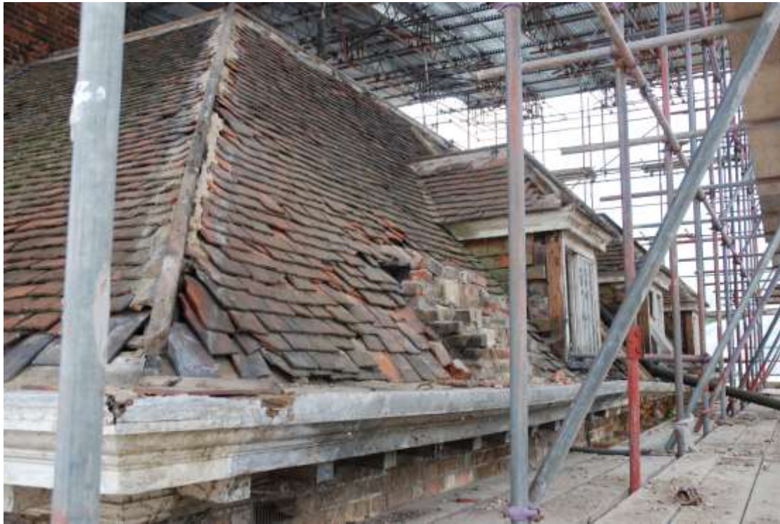
Fig. 54: Remains of the chimney located above the western wall of room S15.
