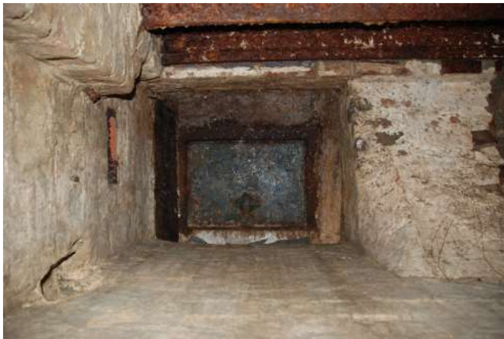
Fig. 118: Photograph looking directly up at the access hatch into the pump room.
