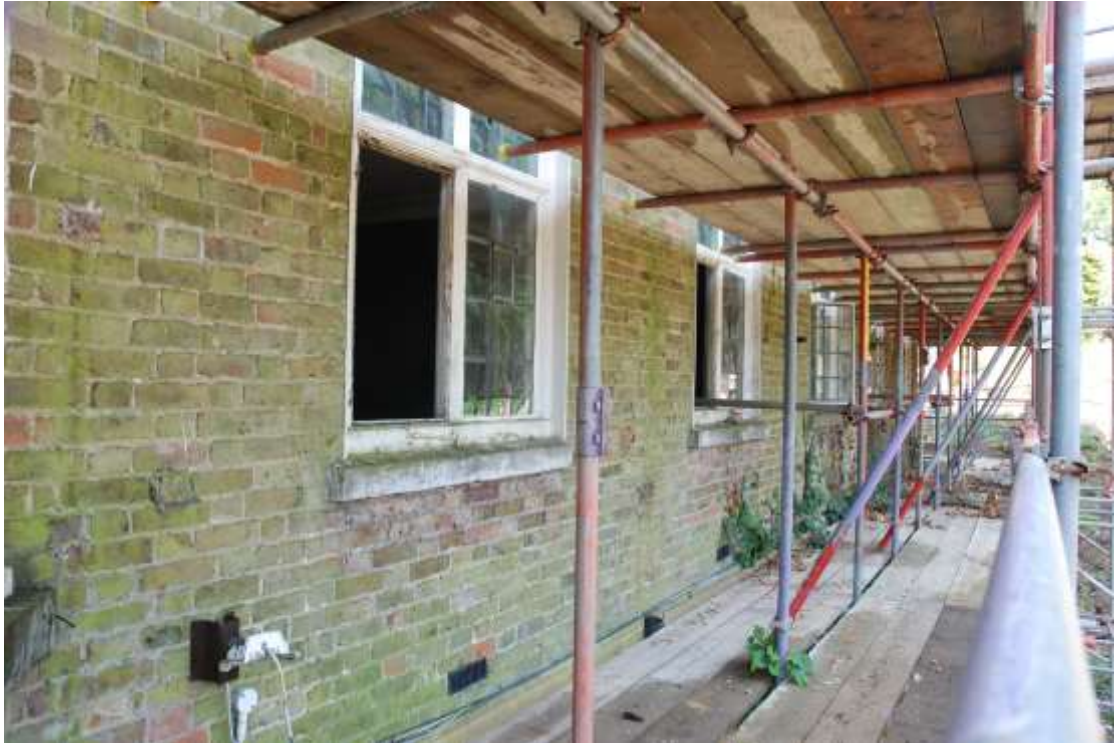
Fig. 29: Northern frontage, at first floor level, just to the west of room F22 (in the area of Partridge's western extension). The later brickwork, set in a regular Flemish bond, can clearly be seen.
