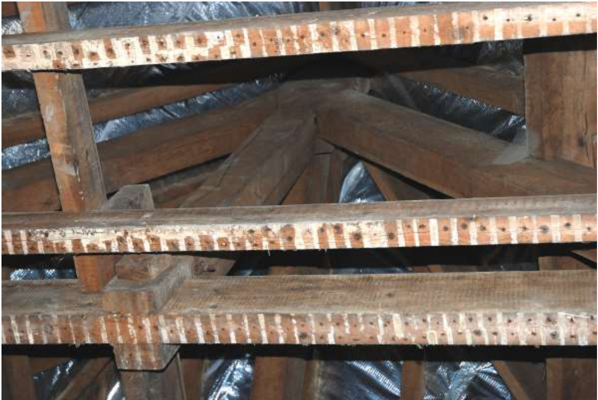
Fig. 102: Photograph looking up into the roof, with the southern king post running vertically up, blades running off it, and the collar beam running across.
