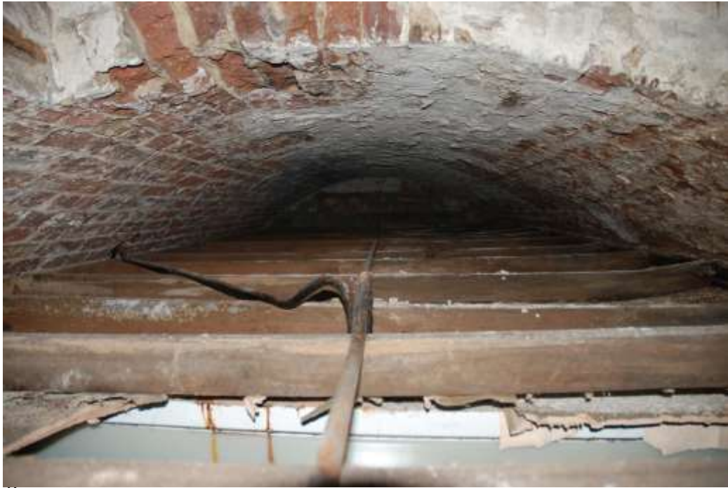
Figure 282: Photograph of the flat ceiling on the western side of the former Beer Cellar, inserted when Breakspears became a care home.
