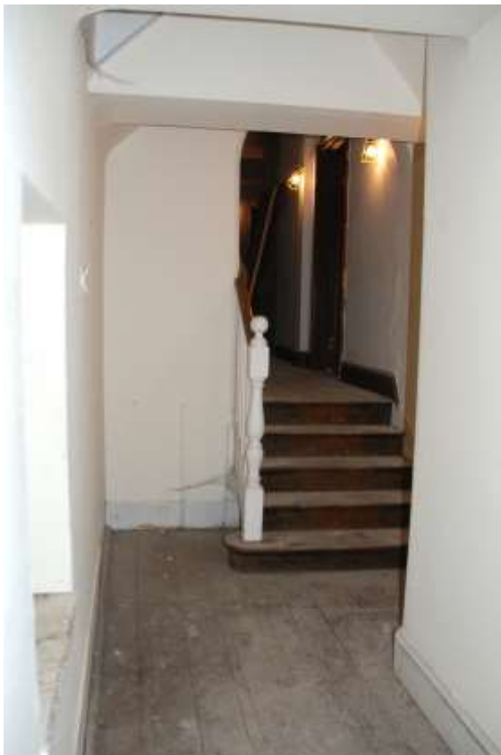
Fig. 228: Stairs on the second-floor, leading up into the area of the eastern extension, and reflecting the raised floor / ceiling level in this area.
