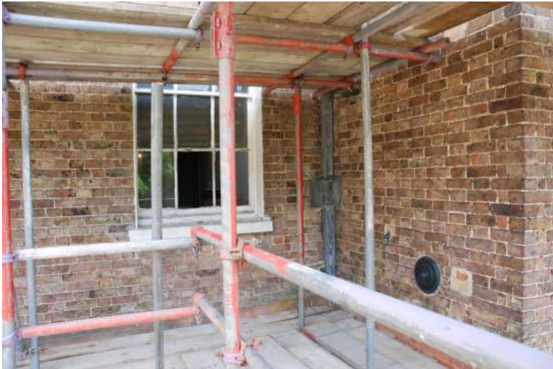
Fig. 32: Walls between rooms F5 and F7, at first floor-level, showing the area rebuilt by Partridge with the more modern brickwork.
