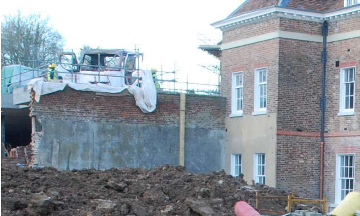
Fig. 60: Photograph showing the rendered areas of wall associated with the conservatory.
