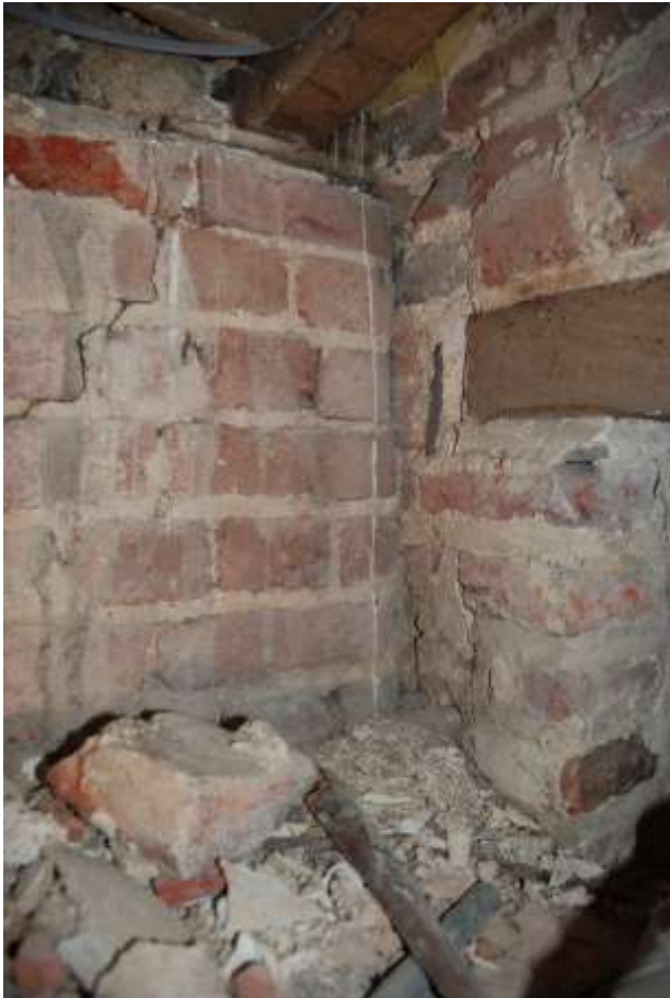
Fig. 173: Photograph of rubble infill and fairly modern secondary brickwork in area of earlier cellars (under the Drawing Room).
