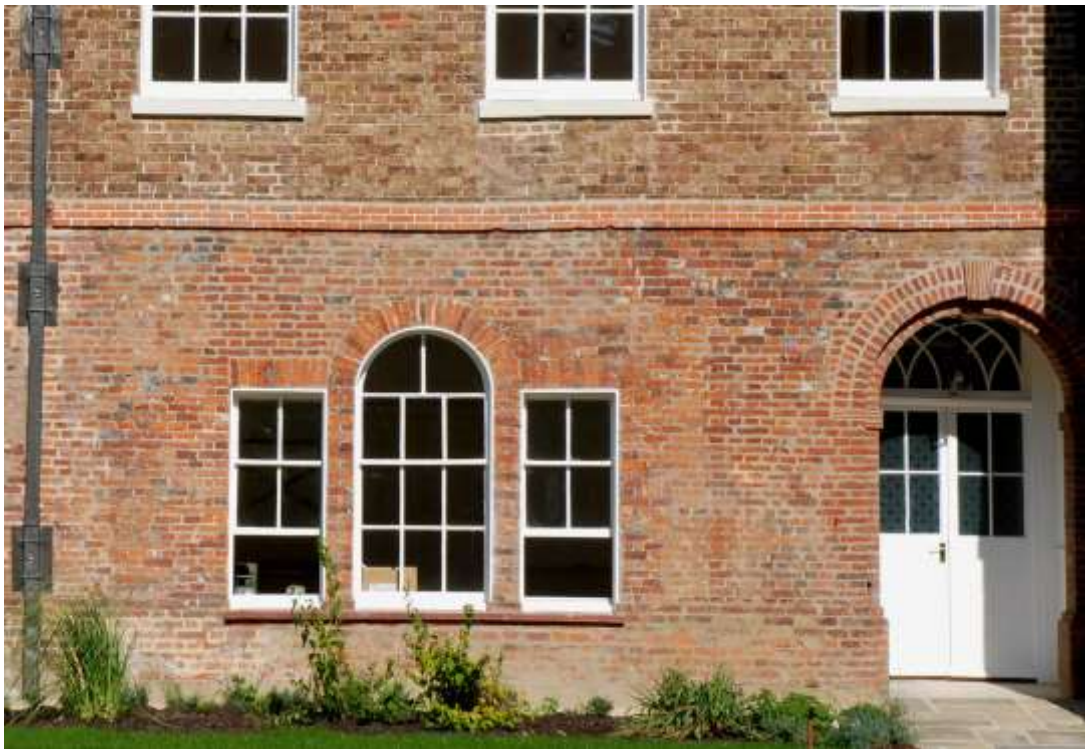
Fig. 145: Venetian window and southern door-arch – they both consist of poor-quality brickwork and the brickwork surrounding them is patchy.
