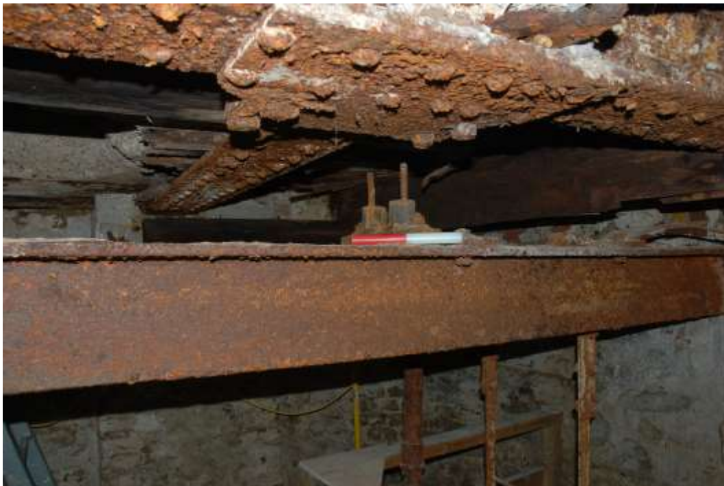
Fig. 120: Photograph of the two levels of girders – the uppermost riveted ones designed to support the overlying walls.
