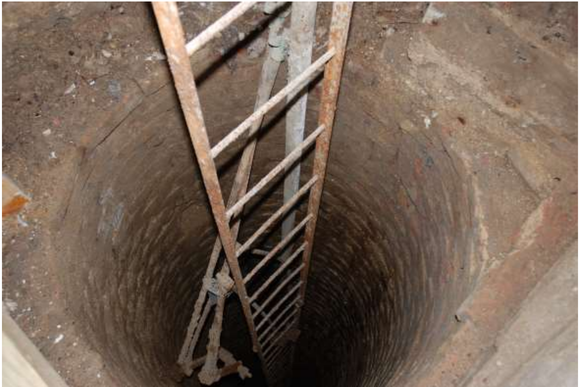
Fig. 113: Photograph looking down the well, with the ladder, actuating rods, and pipe visible.
