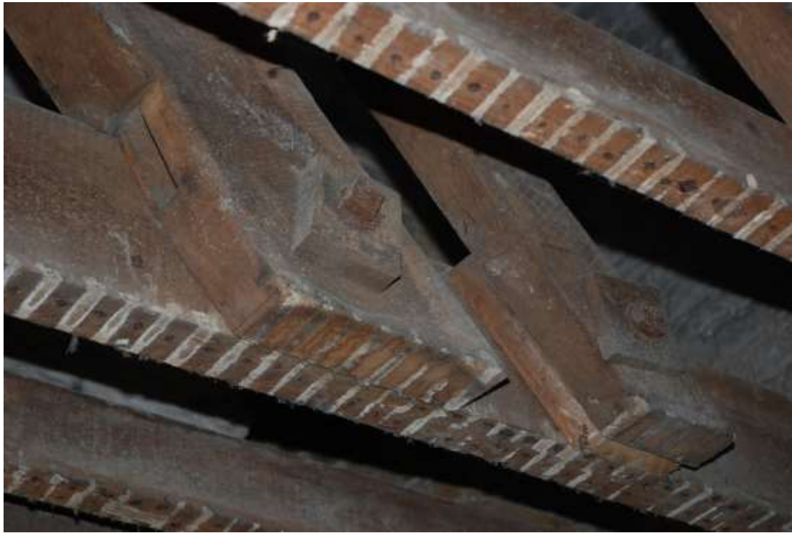
Fig. 103: Photograph of the eastern end of the northern truss, showing the collar and bolted-on blade, with a cut out and deeper mortice for the original raking strut, plus the common rafter bolted on to the right.
