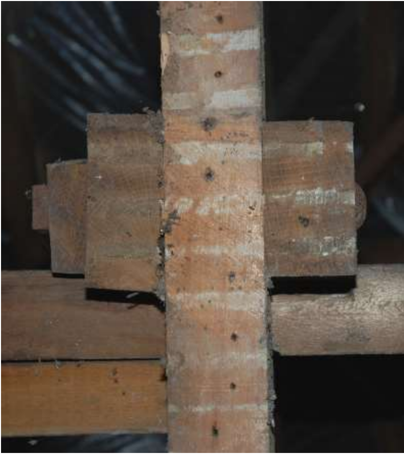
Fig. 101: Photograph of the truncated base of the king post (looking up), with the underside of the collar beam running across (top to bottom of frame) and clasped between the two parts of the king post. The saw marks of the subsequent truncation / removal of lower section are just visible.
