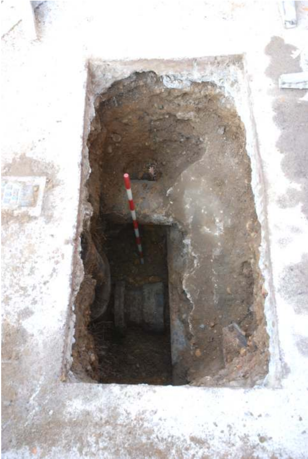
Fig.5: Finished pit, facing W and showing previous cast-iron pipes within trench; the uppermost buried within concrete
