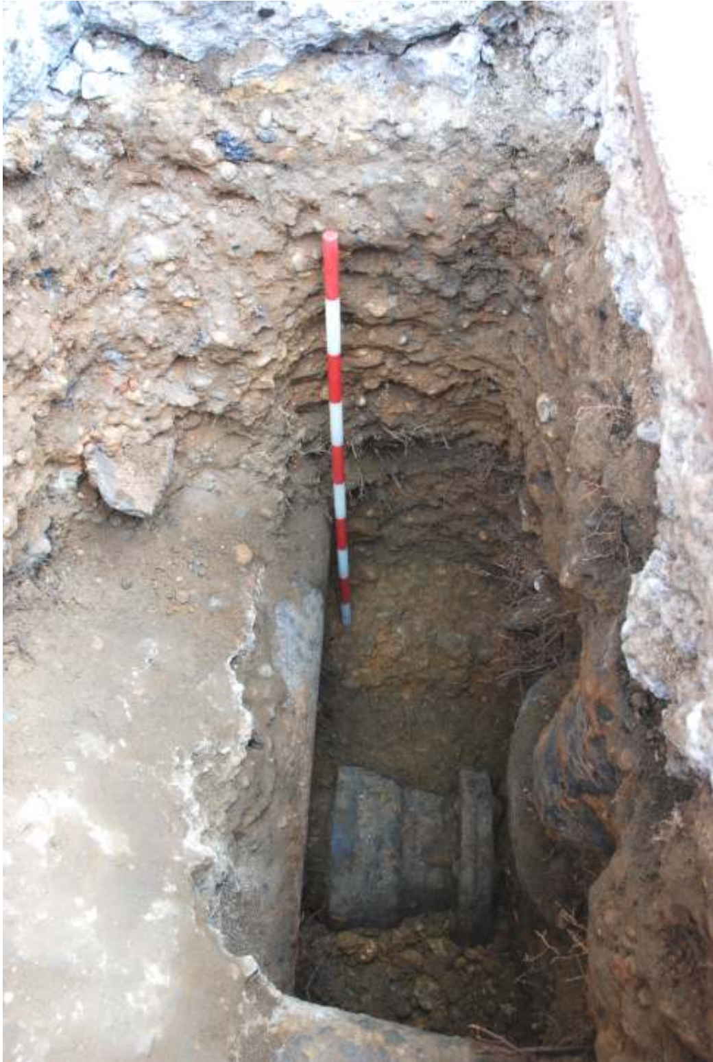
Fig.4: Section through finished pit, facing E. Exposed natural, (5), in base; pipe trench backfill, (3), above; and redeposited natural / backfill, (2), towards top of frame
