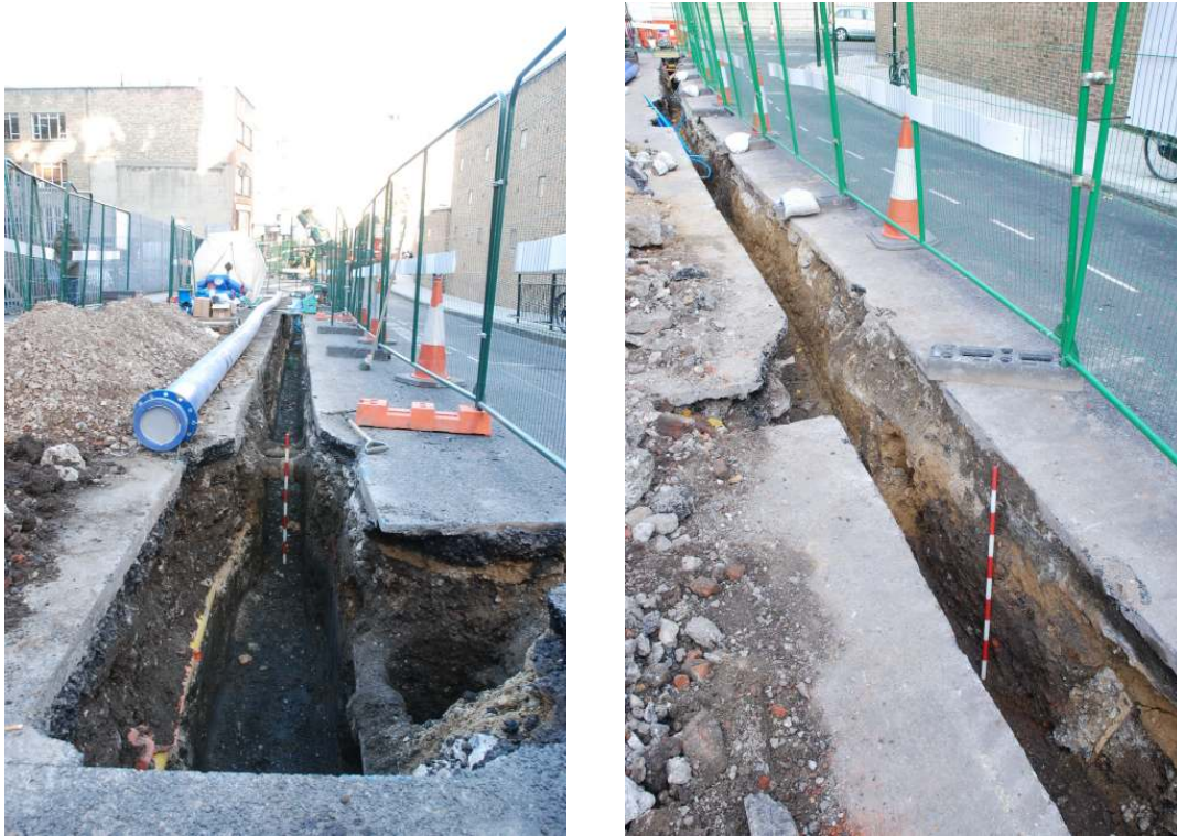
Fig.17: Trenching along Eyre Street Hill, November 2010, facing N, (left), and NE (right) (1m scale)
