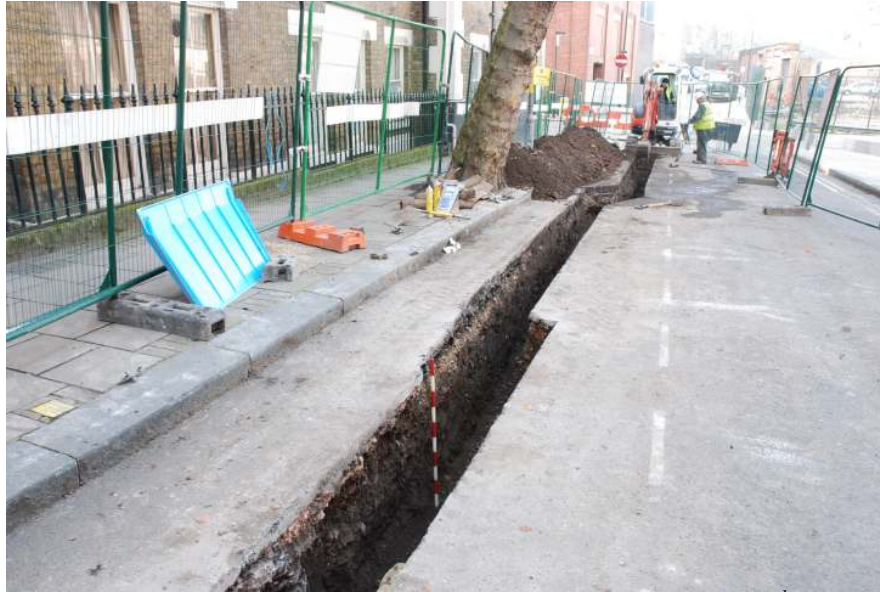
Fig.24: Trench opened on the SW side of Mount Pleasant, 2 nd March 2011, facing S, (1m scale)
