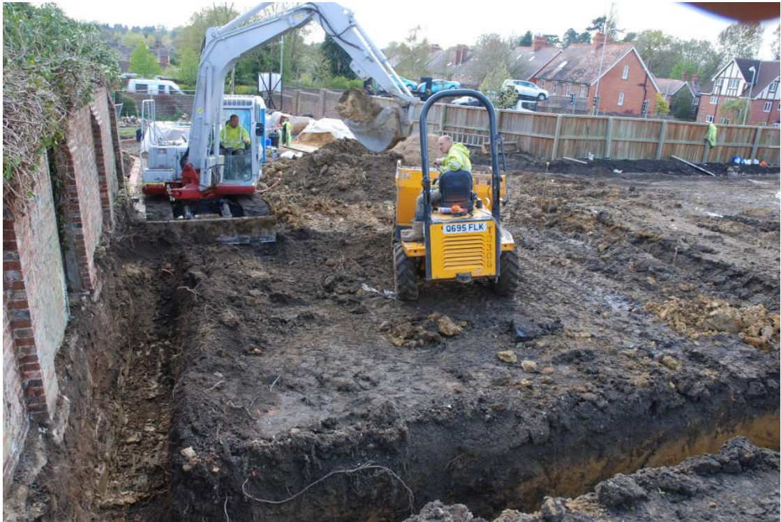
Fig. 36: Photograph of foundation trench 1, looking west. The stepped foundations of the boundary wall are visible.
