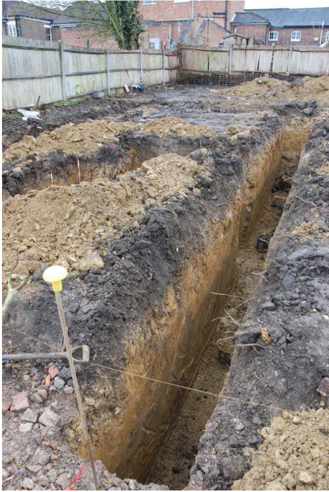
Fig. 21: Photograph of the foundation trenches monitored, looking east. The topsoil over subsoil over natural deposits can be seen.
