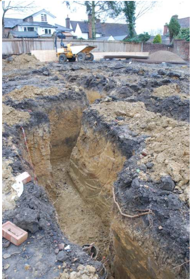
Fig. 22: Photograph of the foundation trenches monitored, looking south-east. The topsoil over subsoil over natural deposits can be seen.
