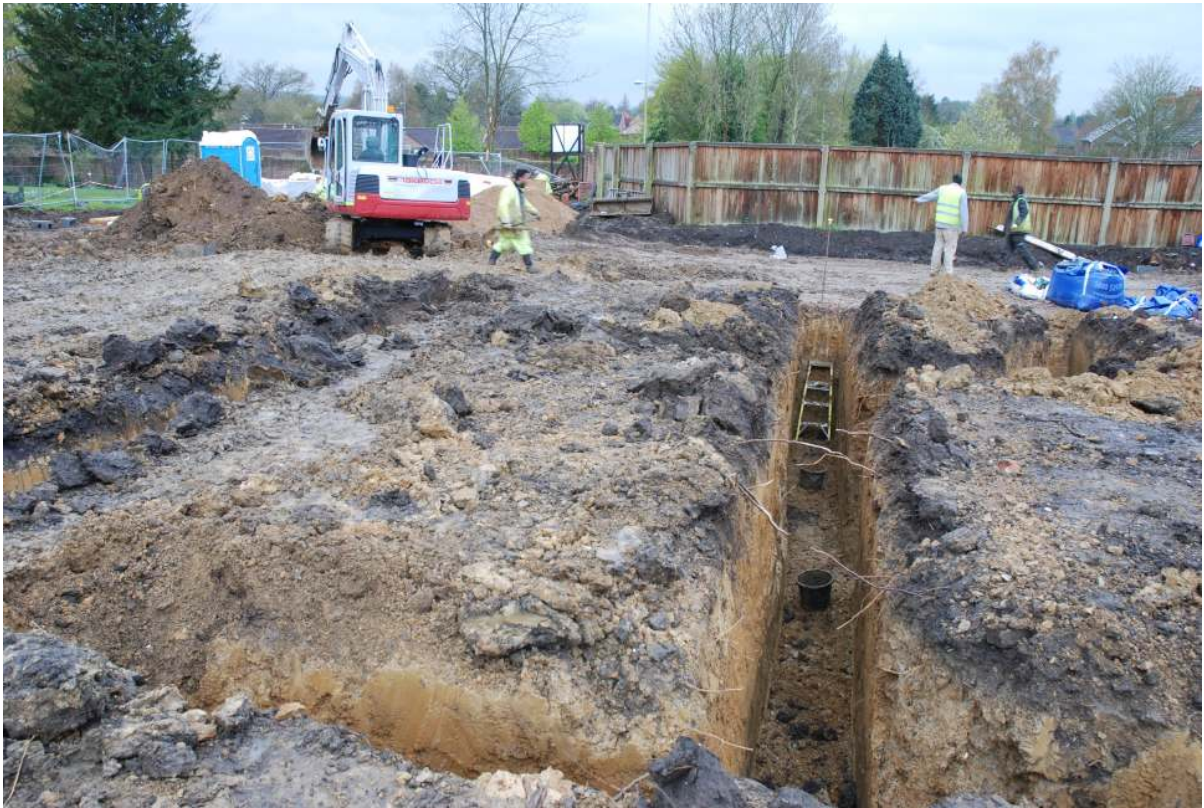
Fig. 23: Photograph of the foundation trenches monitored, looking west. The topsoil over subsoil over natural deposits can be seen.
