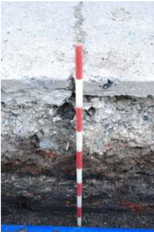
Fig. 24: Photograph of a section in the trenching along Cropley Street, showing the various different made-ground layers.
