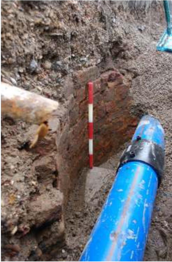
Fig. 96: Photograph of a brick lined soakaway observed in trenching on Wharf Road.
