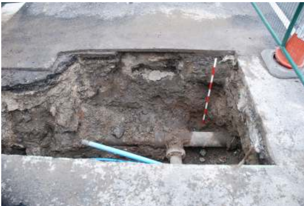
Fig. 34: Photograph of the northern-most pit on East Road, showing the modern road-surface overlying service backfill.
