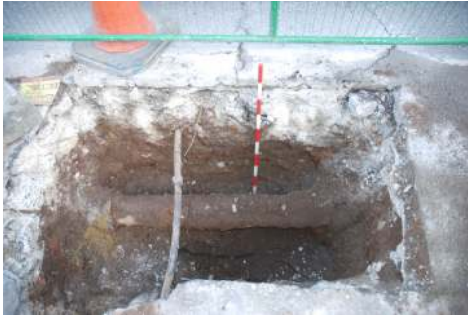
Fig. 21: Photograph of one of the pits on Croyley Street, showing the modern road-surface overlying service backfill and made-ground deposits.
