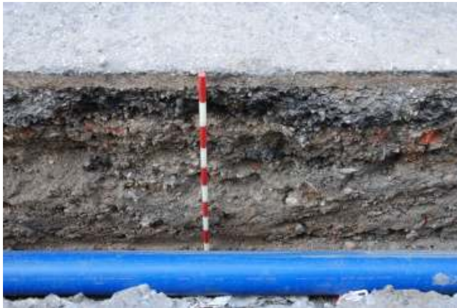
Fig. 46: Photograph of section in trenching along Murray Grove, showing the modern road-surface overlying mixed silty-sand subsoil.
