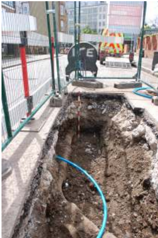
Fig. 83: Photograph of pit on Thoresby Street, showing the large watermain and disturbed deposits.
