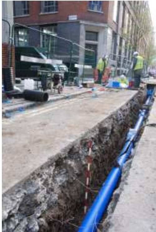
Fig. 73: Photograph of the open-cut trenching on Shepherdess Walk, looking south (towards Underwood Row).
