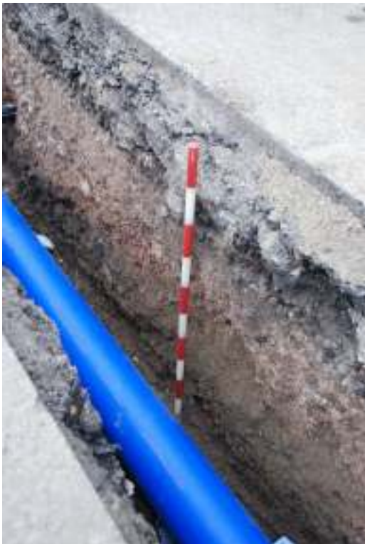
Fig. 78: Photograph of a section of the trenching along Shepherdess Walk, showing the modern road-surface and road make-up deposits, overlying the lighter subsoil.
