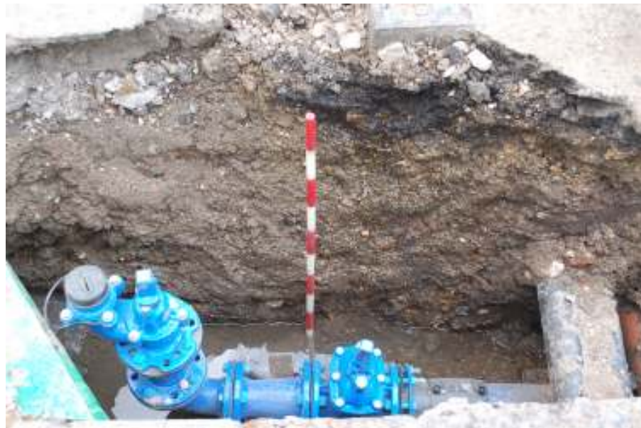
Fig. 11: Photograph of a section in the trenching on Bletchley Street, showing the modern road-surface over service backfill.
