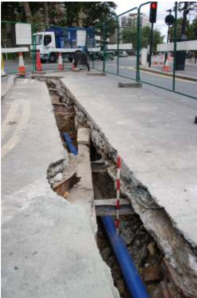
Fig. 51: Photograph of the trenching on New North Road, with the iron girders (supporting the underground toilet's roof) visible.
