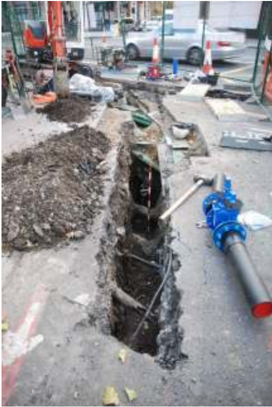
Fig. 71: Photograph of the trenching at the far southern end of Shepherdess Walk, showing modern road-surface over made-ground deposits.
