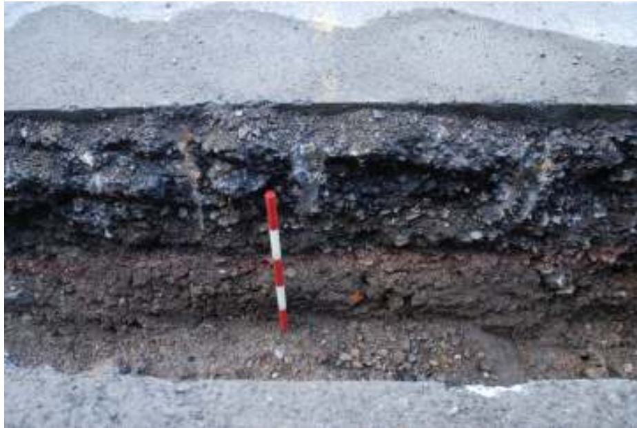
Fig. 76: Photograph of a section of the trenching on Shepherdess Walk, showing the modern road-surface overlying various road make-up layers and made-ground deposits.
