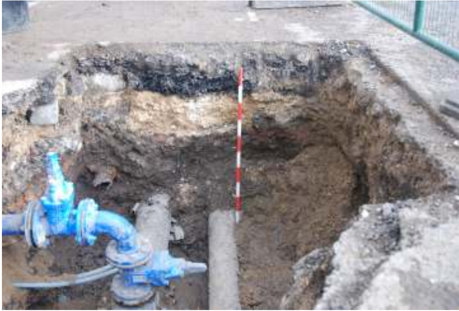
Fig. 27: Photograph of one of the pits on Eagle Wharf Road, showing the modern road-surface overlying disturbed service backfill.
