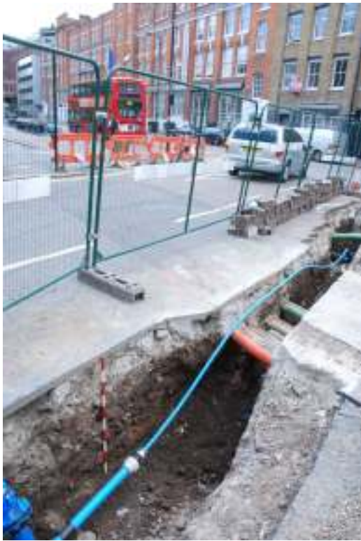
Fig. 41: Photograph of the trenching at the far western end of Haberdasher Street, looking onto East Road.
