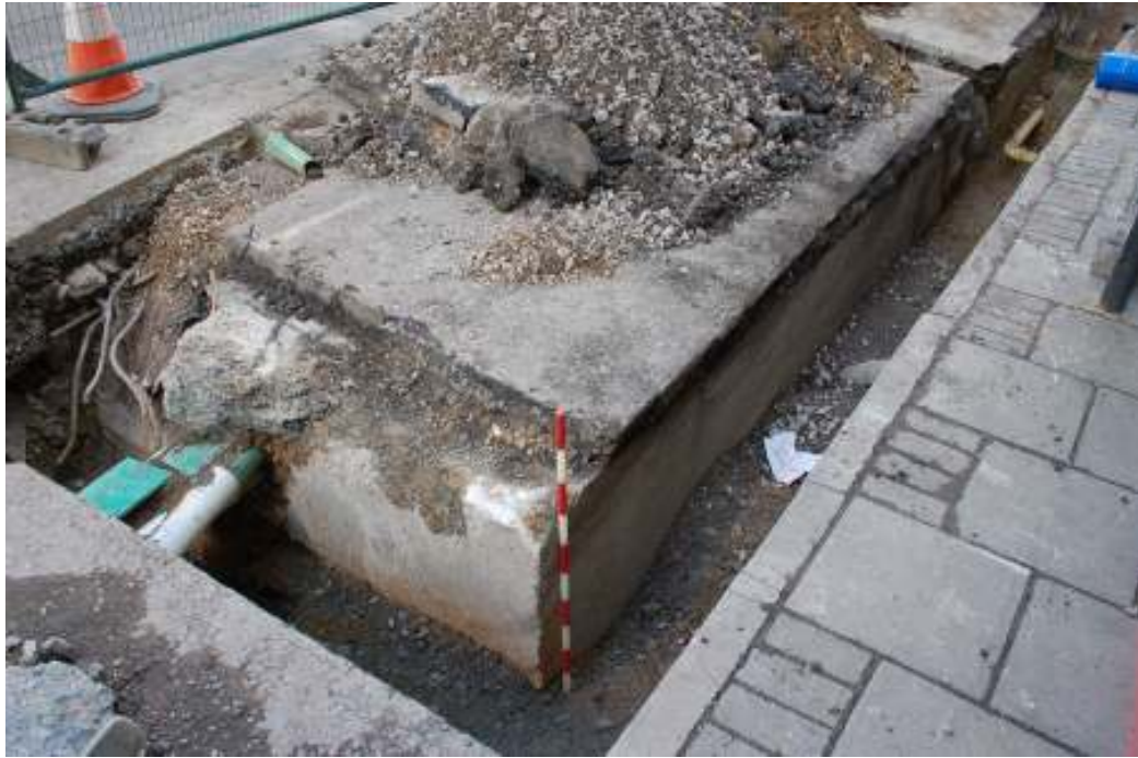
Fig. 97: Photograph of the modern basement slabs observed in the northern end of the trenching on Wharf Road.
