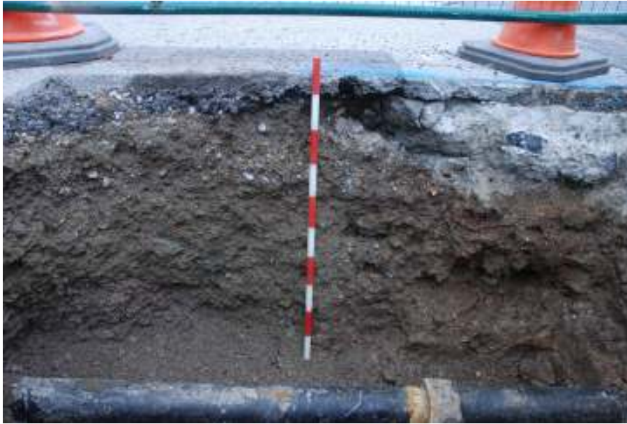
Fig. 14: Photograph of the pit in Cavendish Street, showing the modern road-surface overlying service backfills.
