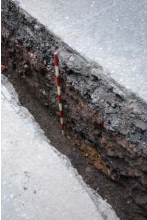
Fig. 8: Photograph of a section of the open-cut trenching on Bevenden Street, showing the modern road-surface overlying various made-ground deposits.
