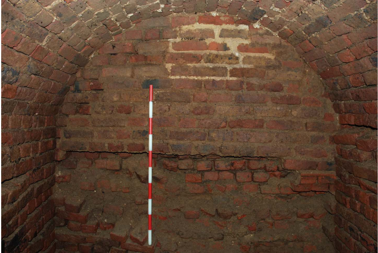
Fig.22: Collapsed face work on the rear wall of the structure. The scale, (1m), rests on surviving face work at the base and the top 40cm, the space in between has collapsed revealing less finely finished brickwork behind. Facing SW
