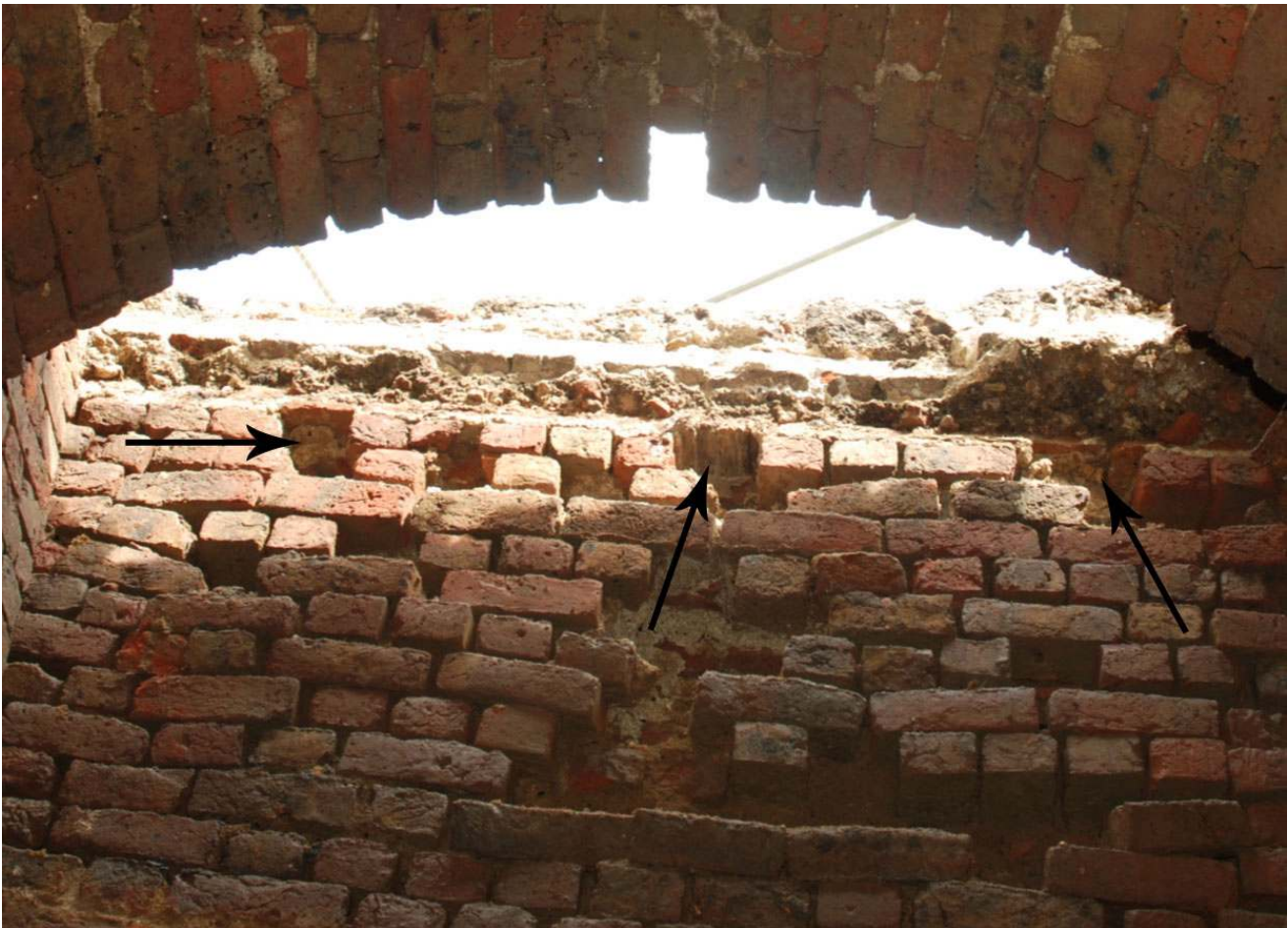
Fig.29: Photograph showing the timber slots on the NE wall face. Note that the central and right hand slot still contains elements of timber. Facing NE
