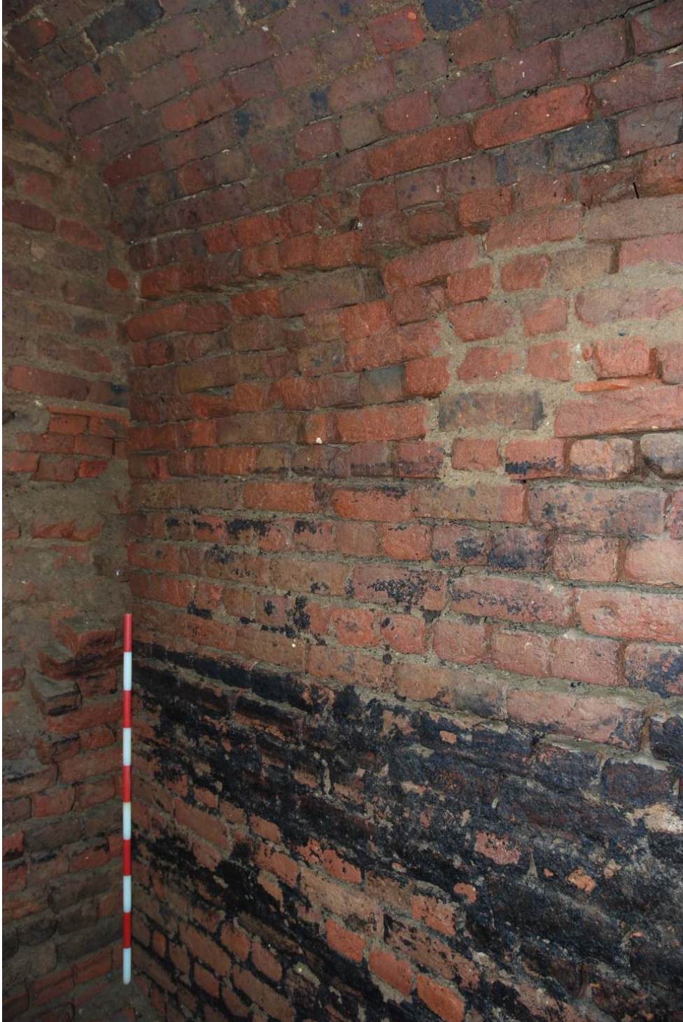
Fig.20: Detail of the W corner of the structure, (left side of frame), illustrating the fact that neither the SW or NW walls are keyed into one another. Facing W, (1m scale)
