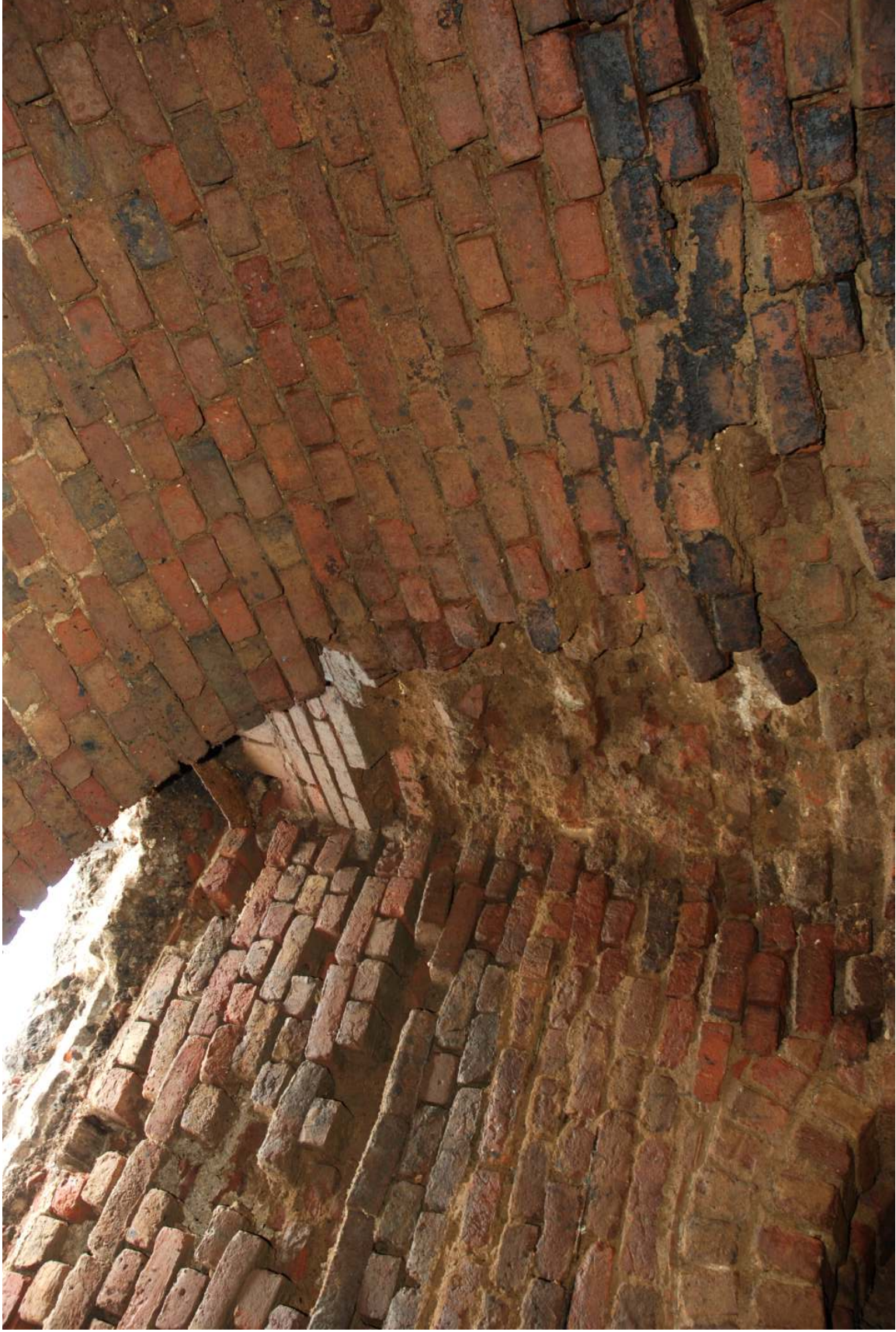
Fig.21: Oblique view of E corner of structure looking up towards the battered face of the SE wall. The arch of the vaulted roof is visible to the right and top of doorway visible to the bottom left of frame
