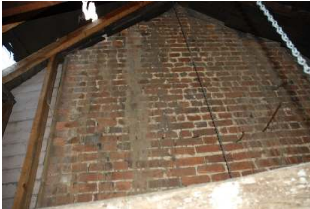
Fig. 64: Photograph of the eastern wall of room 2, which is the western wall of the adjacent house.
