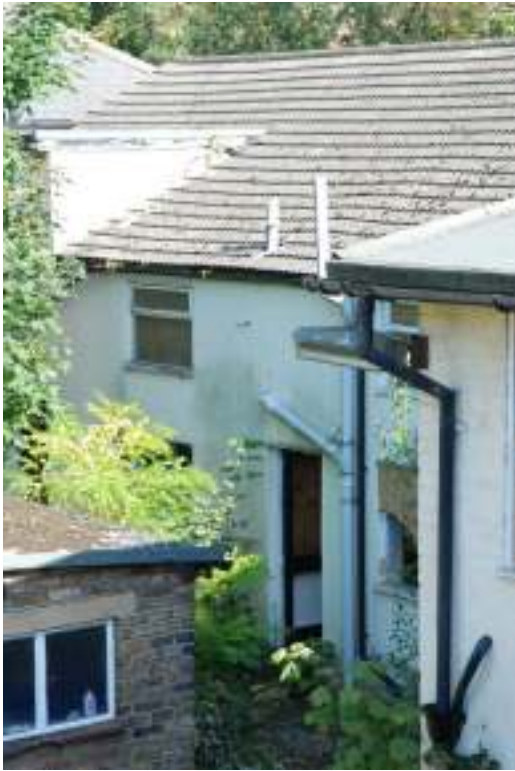
Fig. 31: Photograph of back (northern) of cottages, looking south-east, and showing the raising of the roof in the far eastern part.
