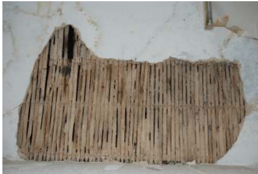
Fig. 42: Photograph of original lathe-and-plaster ceiling, under more modern plasterboard ceiling, in room 25.
