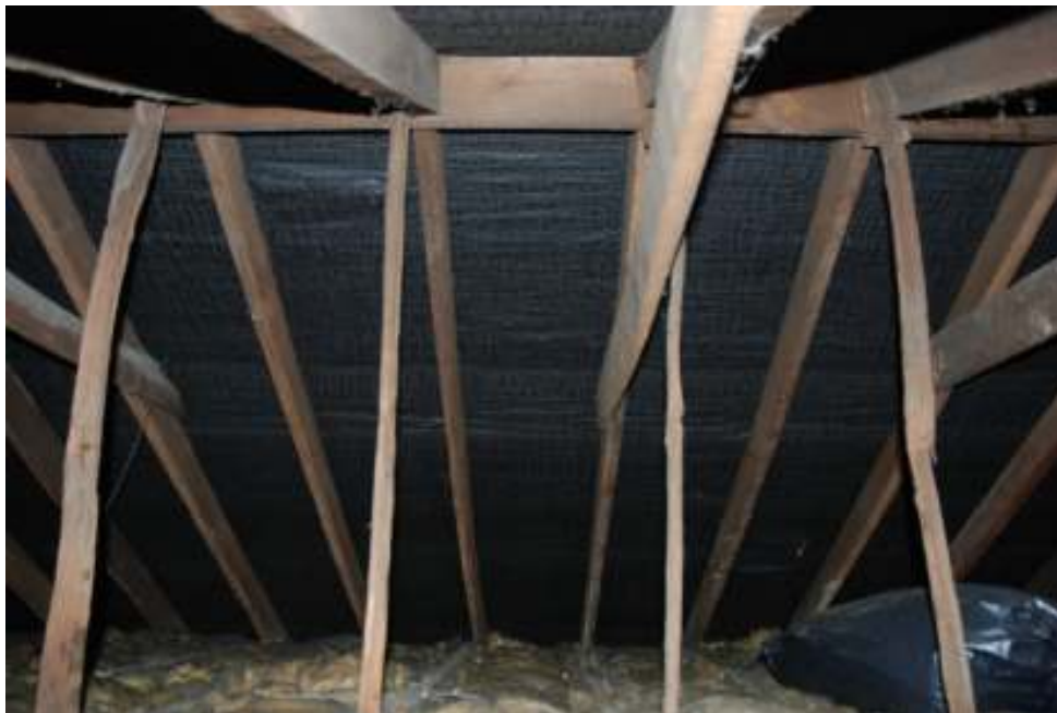
Fig. 20: Photograph of the roof-space above the cottages, showing the original timber structure.
