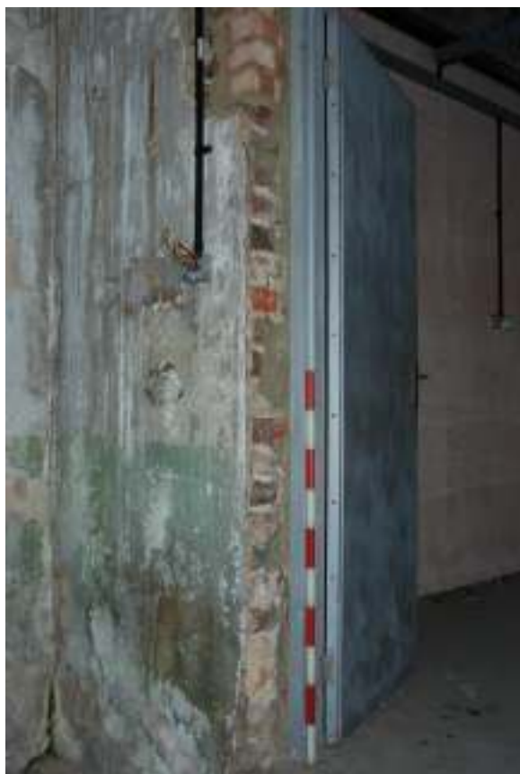
Fig. 107: Photograph of door from room 2 to room 3, showing how it has been cut through the wall at a later date.
