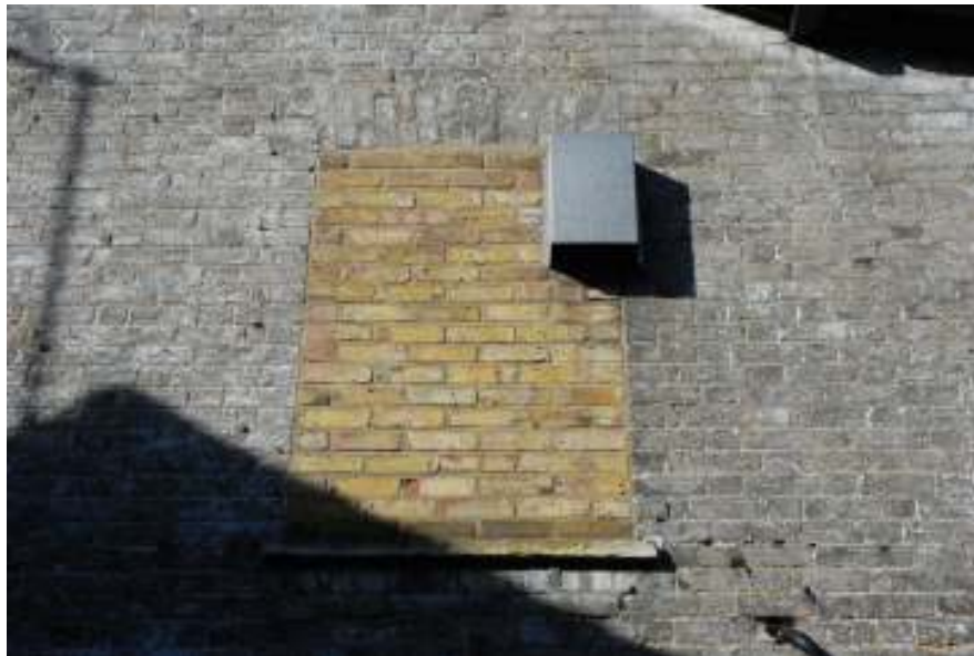
Fig. 59: Photograph of blocked window on eastern wall of main building.
