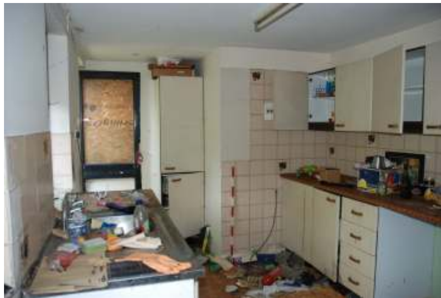
Fig. 15: Photograph of room 10, looking east. The stub-wall, reflecting the line of the original passageway, can be seen behind the scale, with the door, in the position of the original northern exit of the passageway, to the left.
