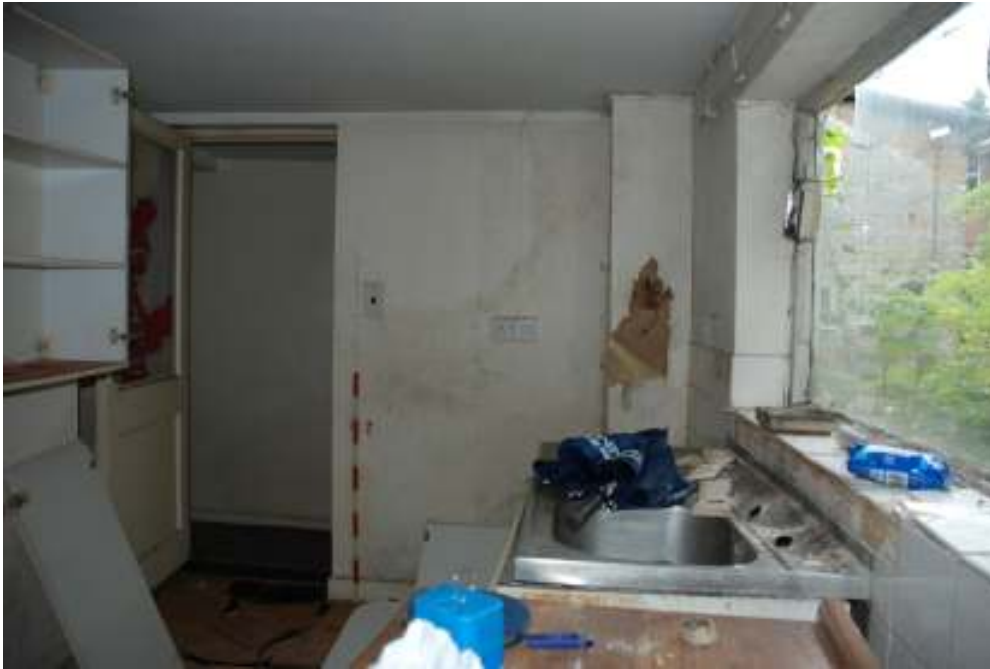
Fig. 25: Photograph of entrance into room 15 from corridor 14 (to the left of the scale).
