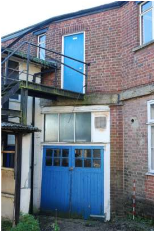
Fig. 108: Photograph showing the keyed-in brickwork at the upper level in the change of angle, and the line in the brickwork at the lower level.
