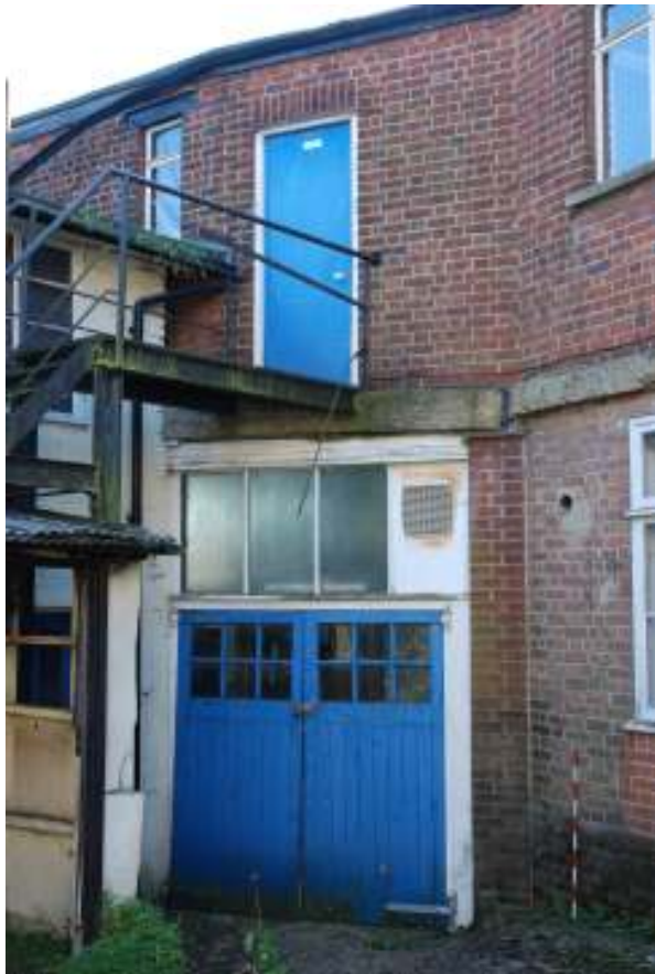
Fig. 96: Photograph of the join between the northern part of room 7 and the north-south building on the western side of the site. Room 6 can be seen overlying this part of room 7, and being constructed of similar brickwork, with room 5 (ground-floor, right of image) abutting room 7 (ground-floor, left of image).
