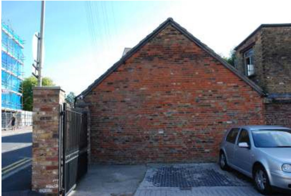
Fig. 69: Photograph of the western wall of the room 2 building, from the outside, showing the red brick and poor construction of this wall.
