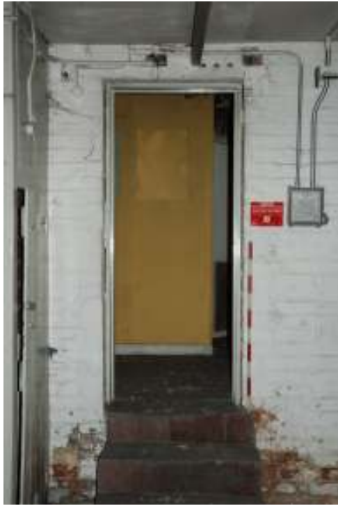
Fig. 38: Photograph of door from room 32 into room 31 - punched through at a later date.
