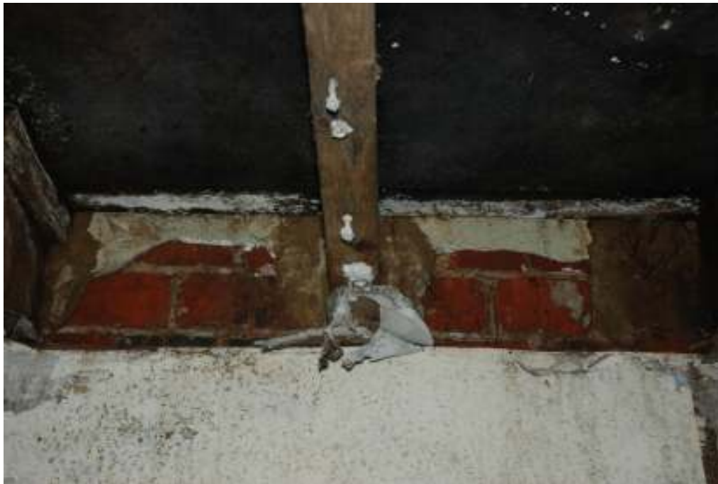
Fig. 30: Photograph of raised ceiling above room 19. The joists here have clearly been punched through the brickwork, and cemented in by modern concrete.
