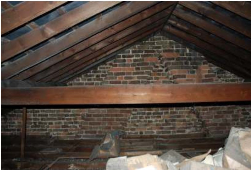
Fig. 46: Photograph of the roof-space above the main building, and the brick wall at the eastern end.
