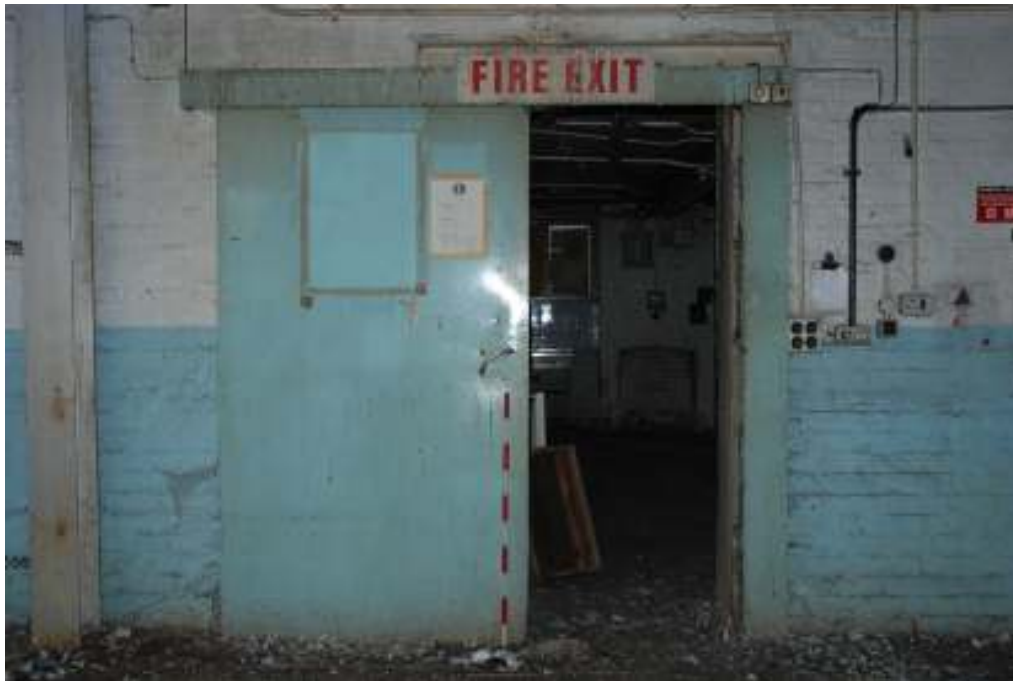
Fig. 90: Photograph of sliding door in eastern wall of room 7, leading into room 32.
