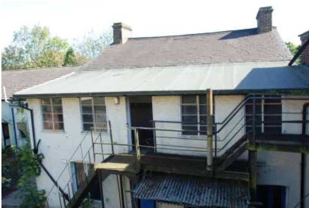
Fig. 52: Photograph of the main building, looking south, and showing the different roof constructions and flattening of the roof.
