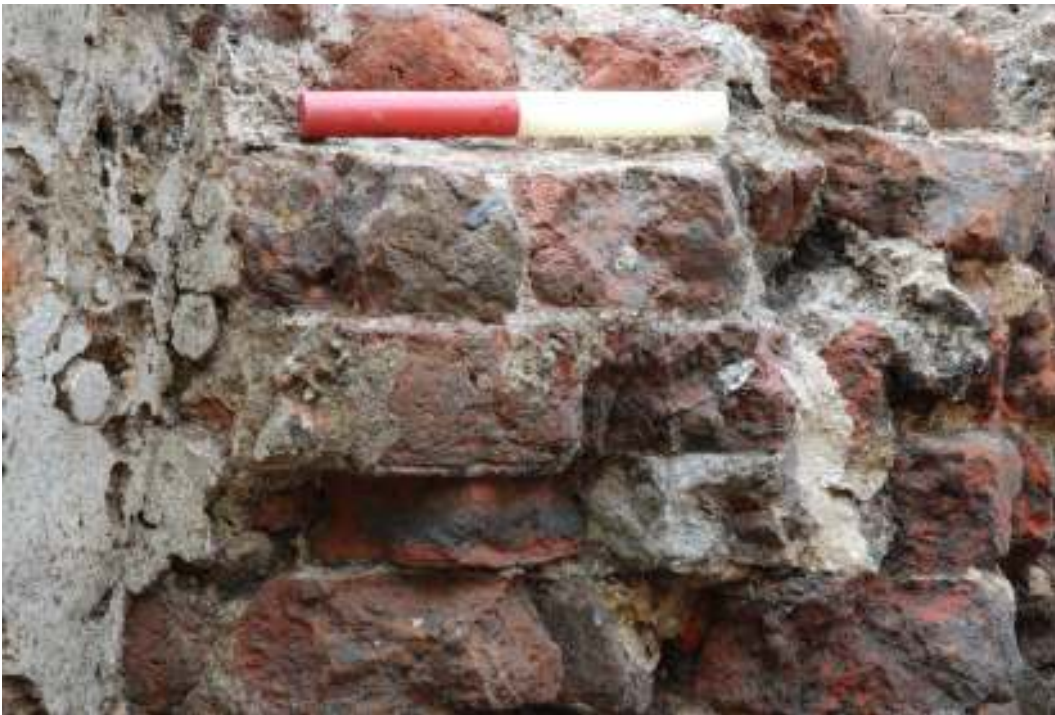
Fig.86: Close-up photo of chamfered brick and tile (presumed reveal and sill) at the western end of the recessed window / lightwell area. (20cm scale)
