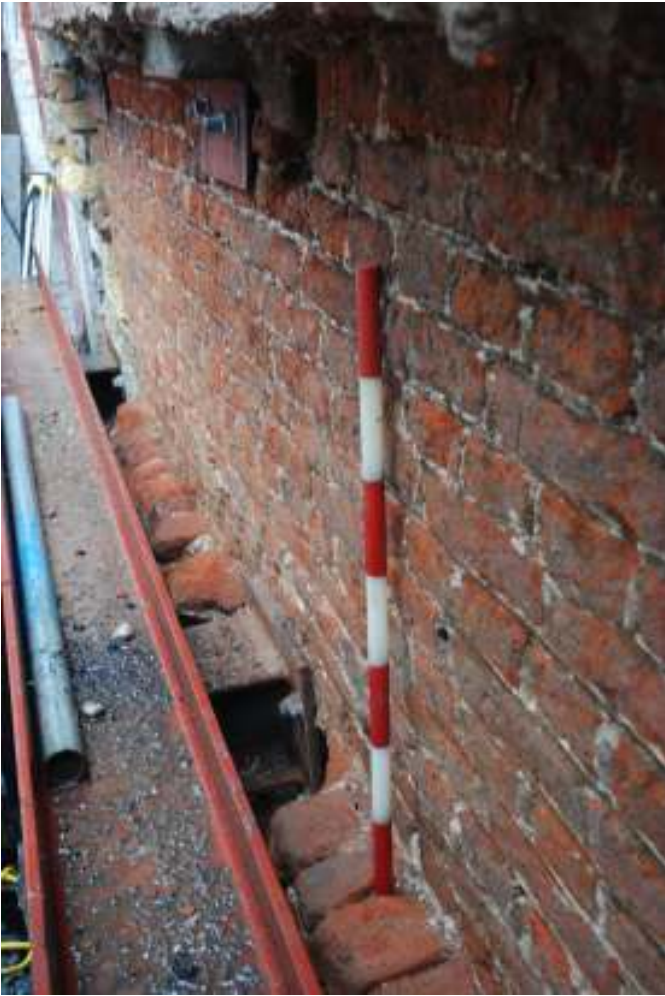
Fig.25: Photo of the 16 th century wall within the standing wall in the southern part of the site, looking south, and showing the rubble foundations. (70cm scale)
