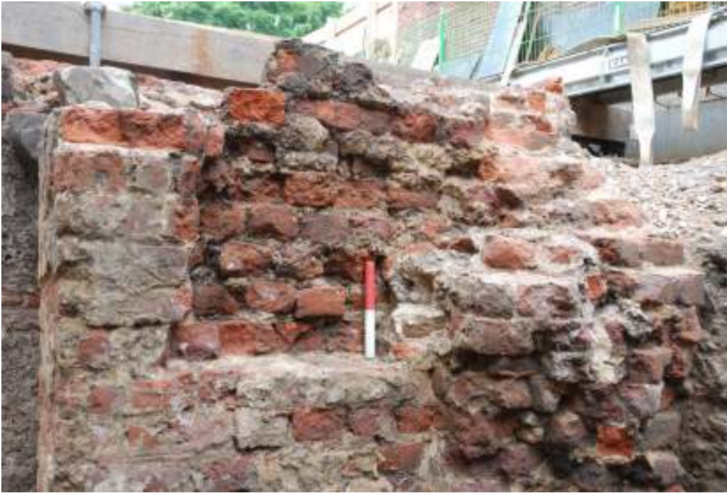
Fig.85: Photo of skim of wall in western wall of recessed window / lightwell area. (20cm scale)
