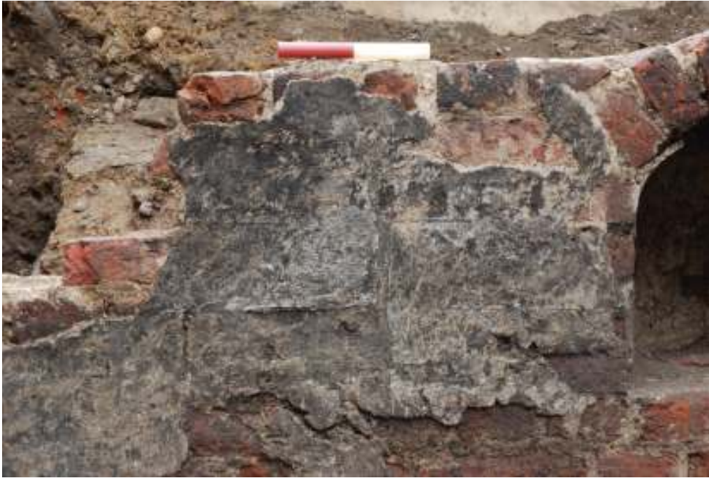
Fig.41: Photo of plaster on the western basement wall, showing indentations which may reflect the position of shelving. (20cm scale)
