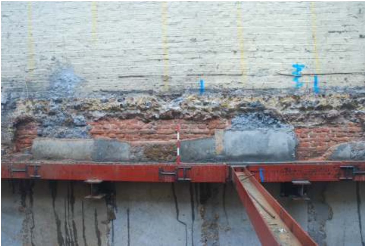
Fig.22: Photo of the 16 th century wall within the standing wall in the northern part of the site. (50cm scale)
