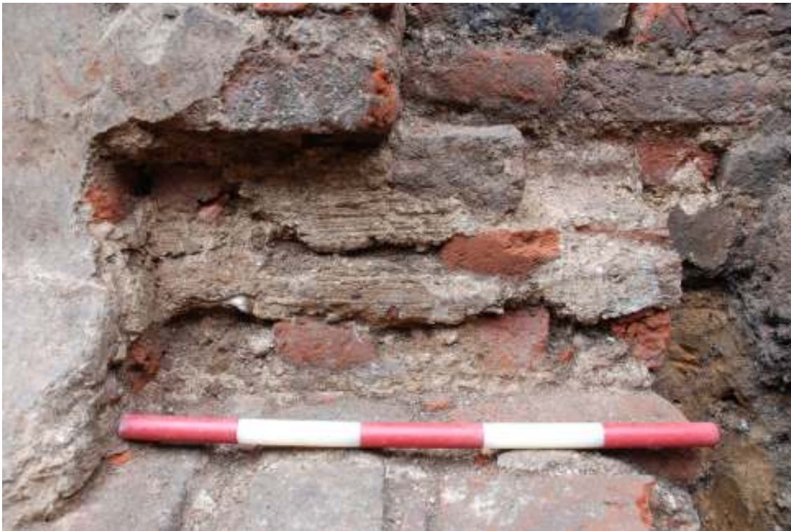
Fig.74: Close-up photo of ledge on [68], showing the imprint of timber on the rear face. (50cm scale)
