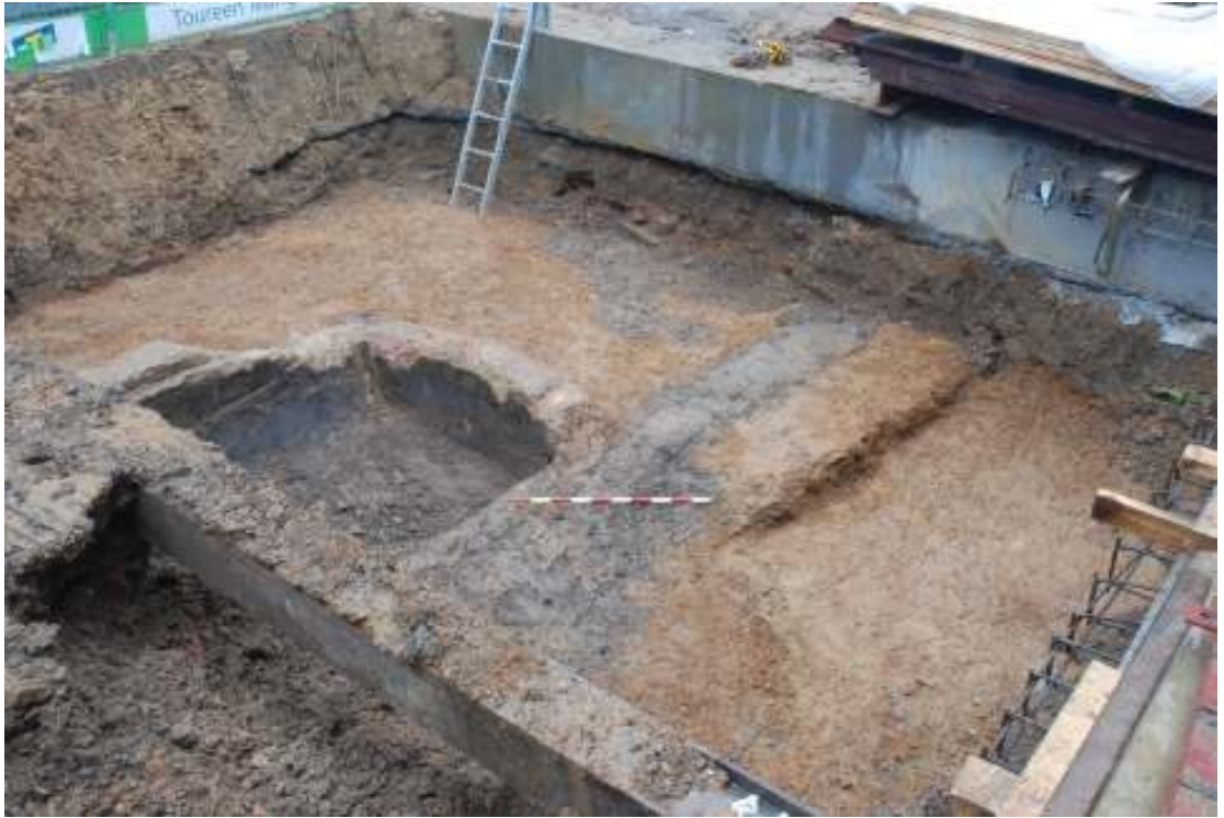
Fig.144: Photo of concrete surroundings of iron tank [13] to the left of the 1m scale
