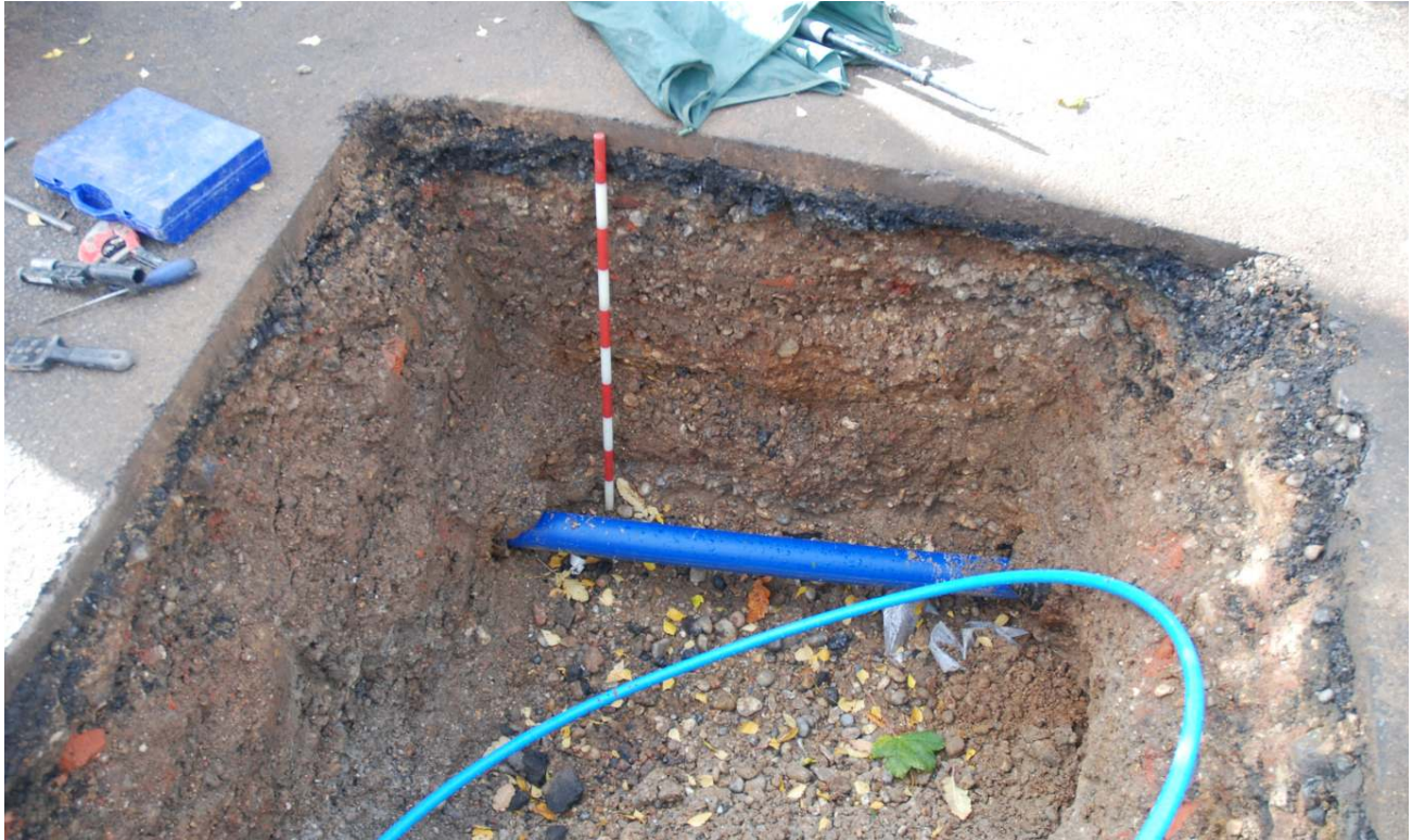
Fig.9: Pit towards the western end of Fairfield Road. Facing S, (5 th October 2012)
