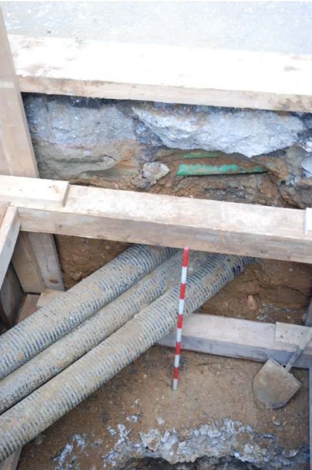
Fig.9: Photograph of shaft 2, looking north. The concrete base of the basement, plus the orange-brown basement infill and later services, are all visible.
