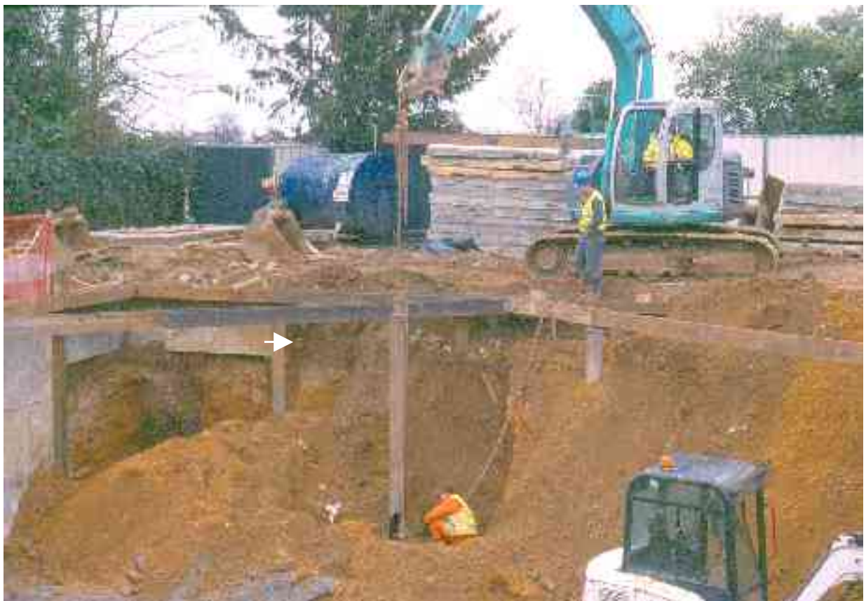
Fig 5 View looking east during the final stage of the excavation, with the small area of in situ brickwork in Figures 6 & 7 arrowed
