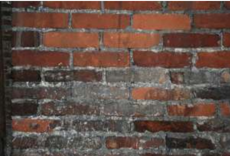
Fig.18: Photo showing the small section of limewashed brickwork in the northern chimney, possibly on the line of the original exterior wall (taken within the roofspace of the later western extension)
