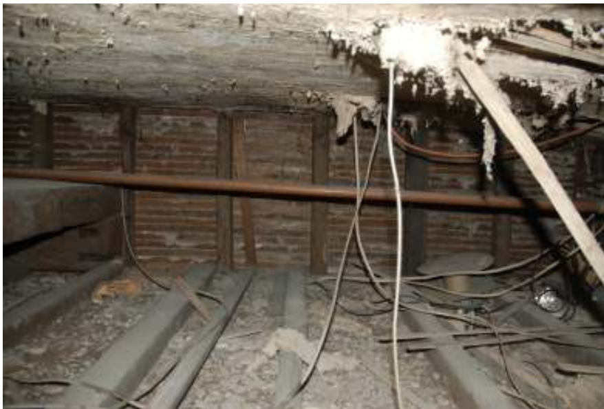
Fig.55: Photo of wall between rooms 11 and 12, looking west, and showing its substantial nature. The gap between the floor of rooms 17 and 18, and the ceiling of room 11, is also visible here
