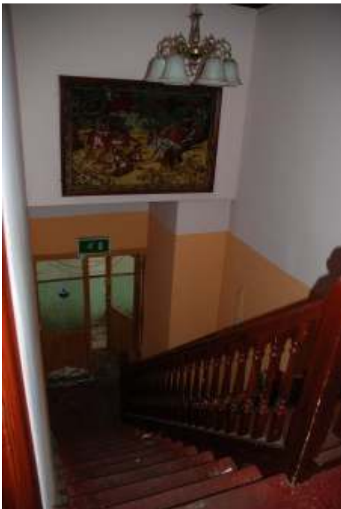
Fig.58: Photo of the stairs positioned within the first south-western extension, looking south
