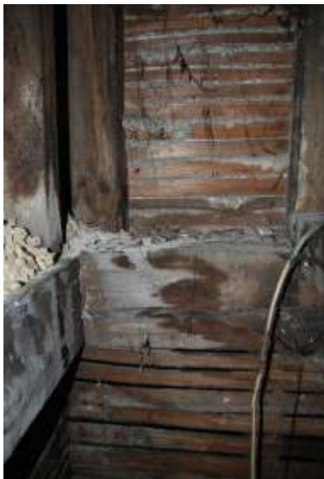
Fig.56: Photo showing the large timber in the wall between rooms 11 and 12 (probably the wall of the first south-western extension)
