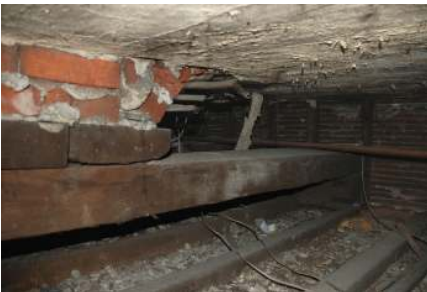
Fig.54: Photo showing the southern chimney 'kinking back', looking south-west, and showing the northernmost of the two basal supporting beams
