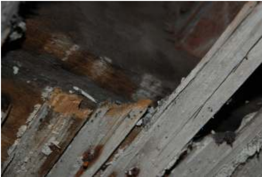
Fig.26: Photo of lath-and-plaster ceiling in room 1, with imprint of possible earlier lath-and-plaster on timber underneath
