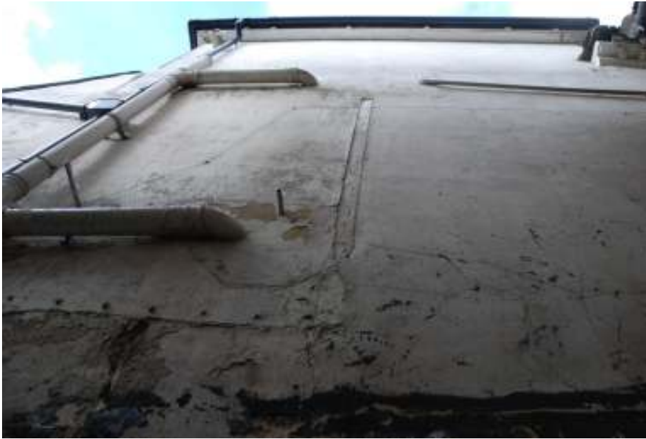
Fig.57: Photo of the piece of timber in the exterior southern wall, on the line of the first south-western extension
