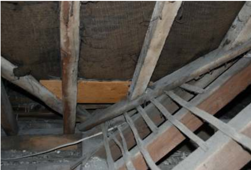
Fig.43: Photo of the roof of the junction between the rooms over the passageway and the original part of the building. The roof of the rooms over the passageway (left of frame) overlies the laths of the roof over the original building (right of frame)
