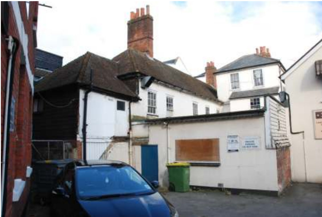
Fig.65: Photo showing the different roof construction in the south-western extension (right of frame)
