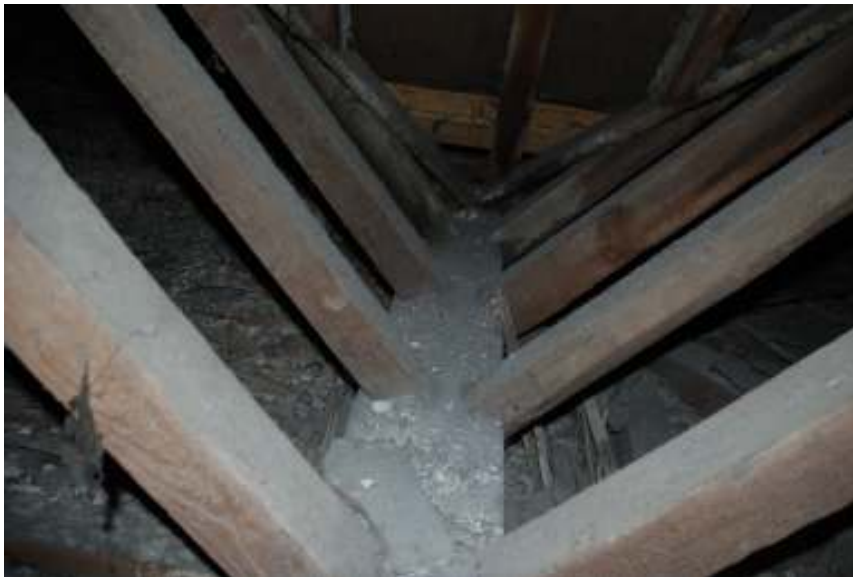
Fig.31: Photo of the roof timbers over the original part of the building, showing how the rafters in the rear (western) part are attached to the central beam differently from those in the front (eastern) part
