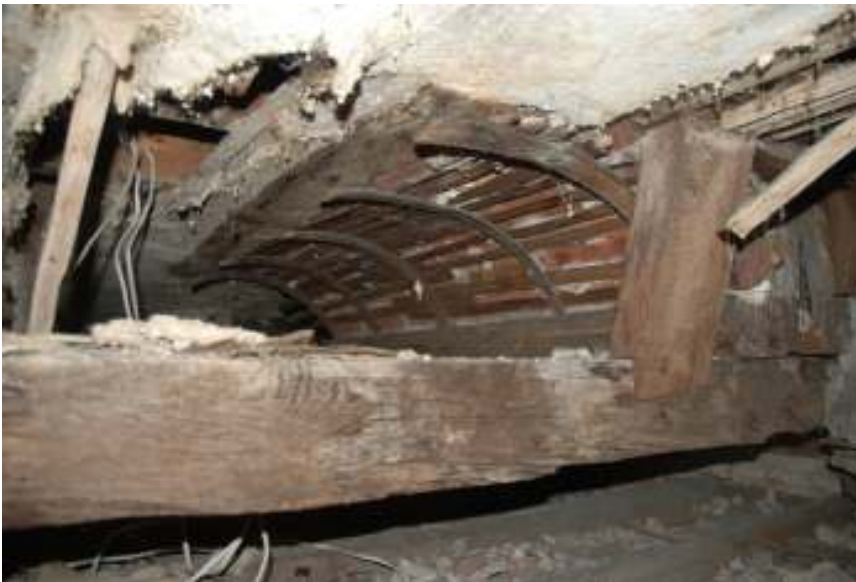
Fig.53: Photo showing the southern chimney 'kinking back', looking north-east. This shows one of the large supporting timbers in the foreground with brickwork supported on laths and rising up to a second north-south timber at the top of the frame
