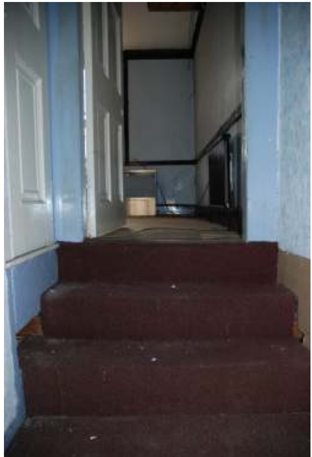
Fig.64: Photo of stairs leading up to the second south-western extension, on the second-floor
