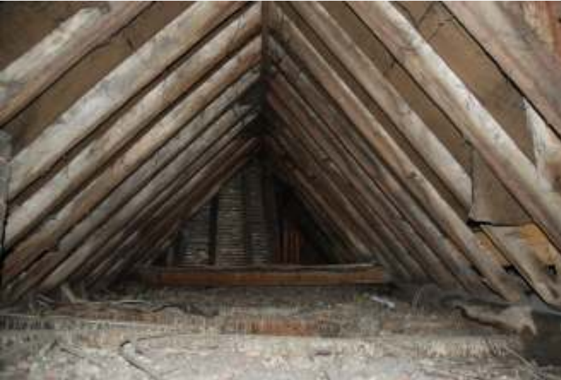
Fig.19: Photo of the double-hipped roof over the original part of the building
