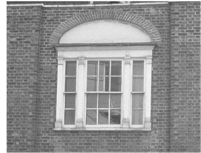
The first-floor tripartite window with decorated pilasters, frieze and dentil cornice, plus gauged cambered arch above the spandrel
