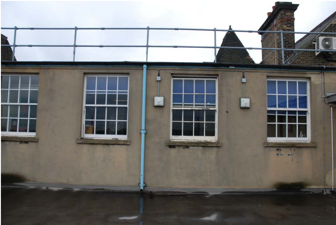
Fig.38: Close-up of the new northern wall of room 4, exterior face, showing rendering and wider 4-pane windows
