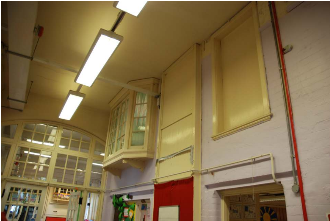
Fig.50: The panelling showing the area of the dumb waiter on the first-floor, viewed from the central lobby, looking south-east
