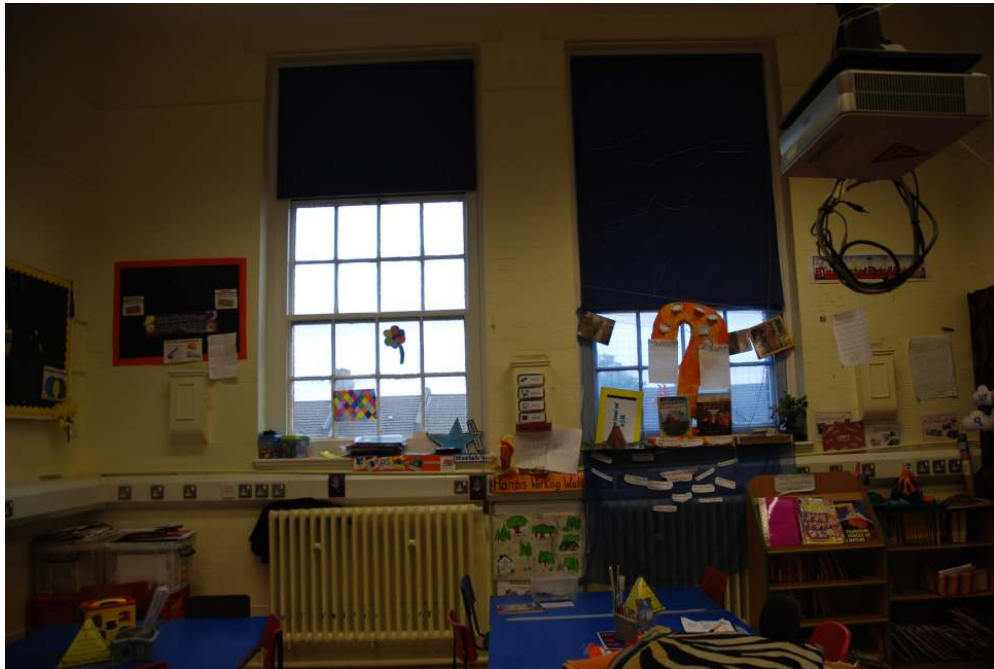
Fig.75: The northern wall of room 9, showing the original windows and three ventilation boxes
