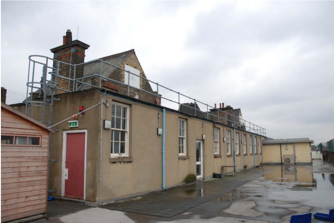
Fig.37: The northern exterior face of room 3 (in foreground) and room 4 (in background), rendered over
