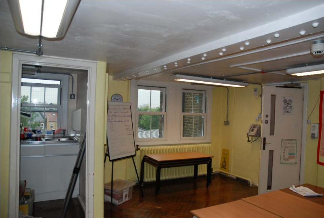
Fig.64: Mezzanine level 2B, looking south-west, showing the area of the proposed new lobby
