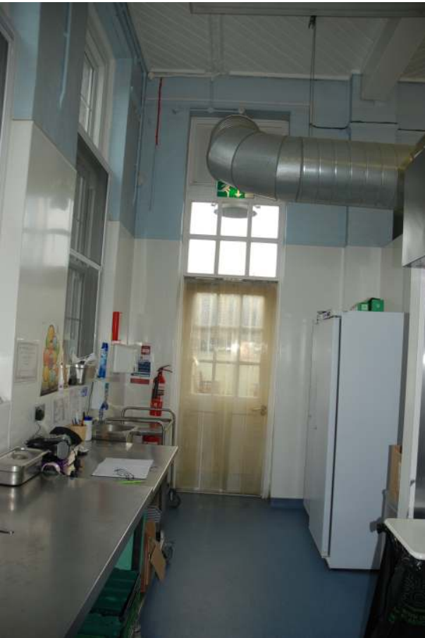
Fig.56: The door to the exterior in room 15, with the original lower part of the overlight
