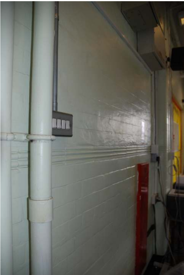
Fig.21: The string course running along one of the original walls in room 4, but seen throughout the school
