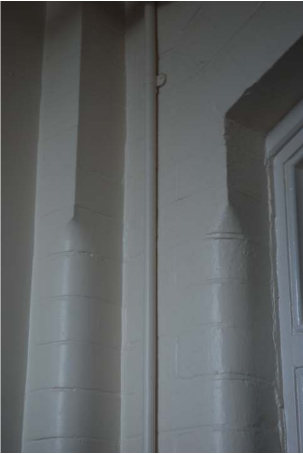
Fig.20: The rounded (bullnosed) corners of brickwork in one of the corners in room 3
