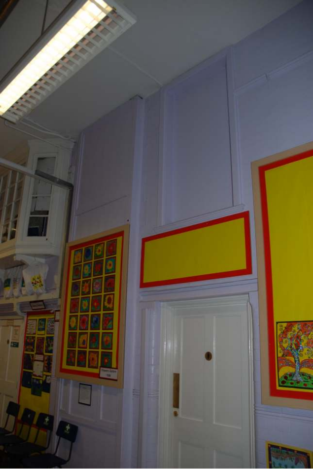
Fig.51: The panelling showing the area of the dumb-waiter on the ground-floor, between the door on the right of frame and high-level internal window to left
