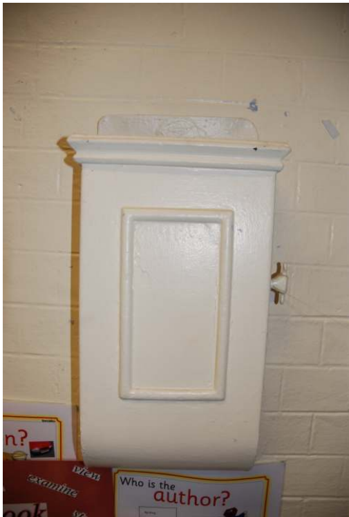
Fig.76: One of the ventilation boxes on the northern wall of room 9
