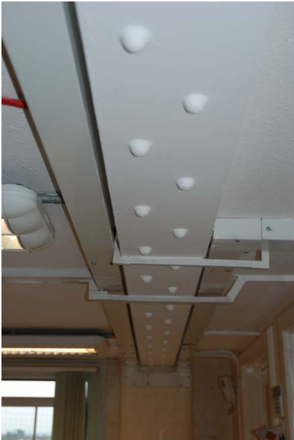
Fig.63: The original riveted cross-beam, in mezzanine level 2A, but seen elsewhere across the building
