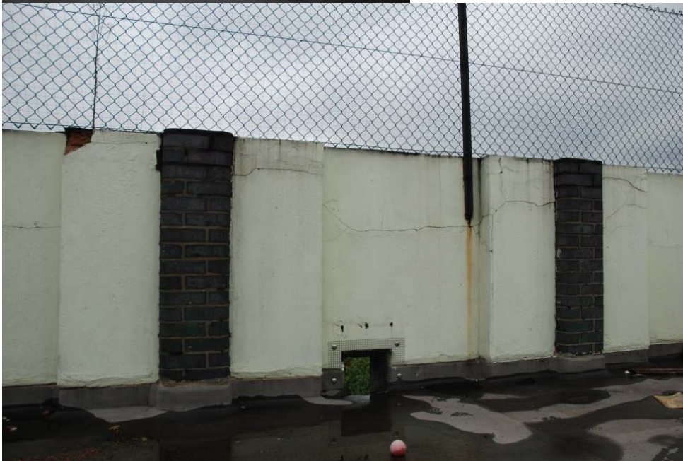
Fig.34: Some of the engineering brick abutments on the perimeter of the building
