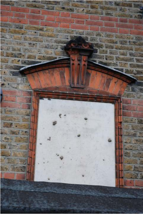
Fig.38: Plaque recording the opening of the school, on the original western frontage of the building
