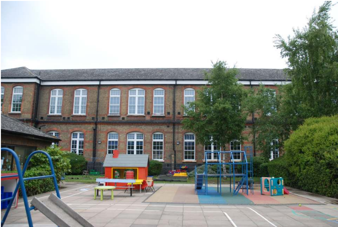
Fig.19: The southern side of Central Park School today, showing the new roof
