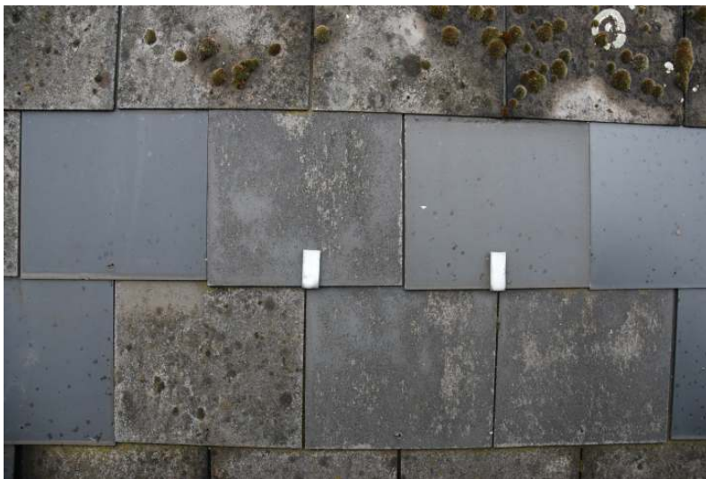
Fig.22: The artificial slate tiles on the roof today (some clearly replaced quite recently)
