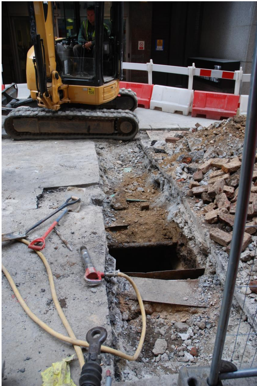
Fig.8: Pit 2 facing ENE with services present at both ends and the sondage sunk into the passageway in the centre
