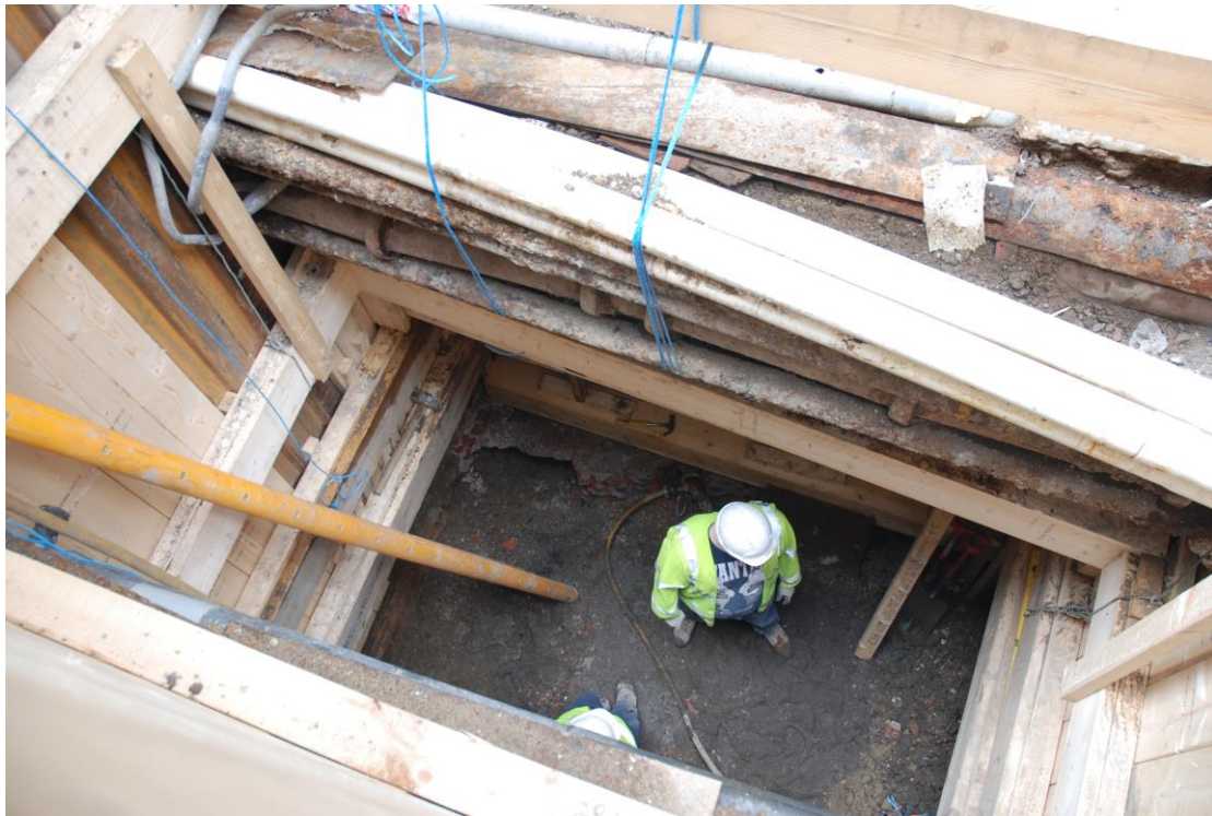
Fig.12: Pit 3 facing SW showing shoring down to 3.5m below ground surface. Base of pit at 4.2m
