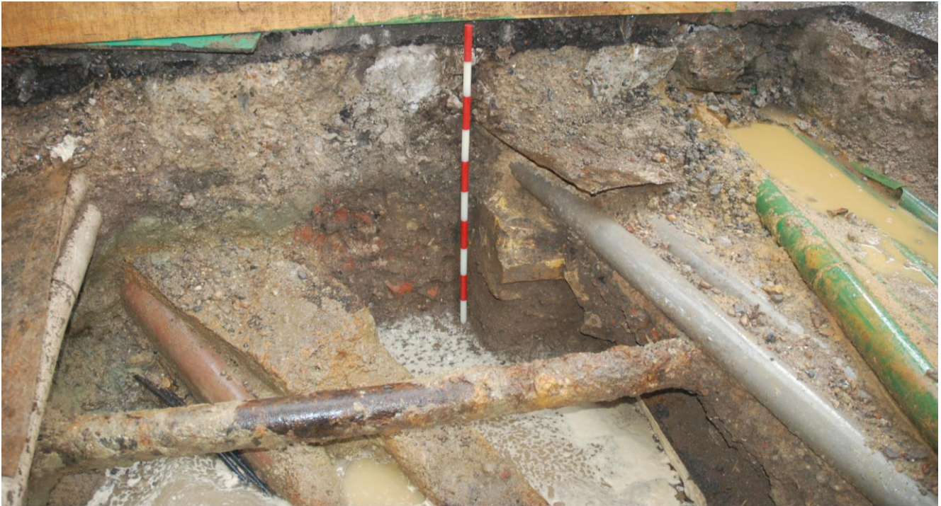
Fig.7: Pit 1 facing NNE showing the column of surviving 18 th century made ground, modern wall footings and the abundance of existing services crossing the roadway (1m scale)
