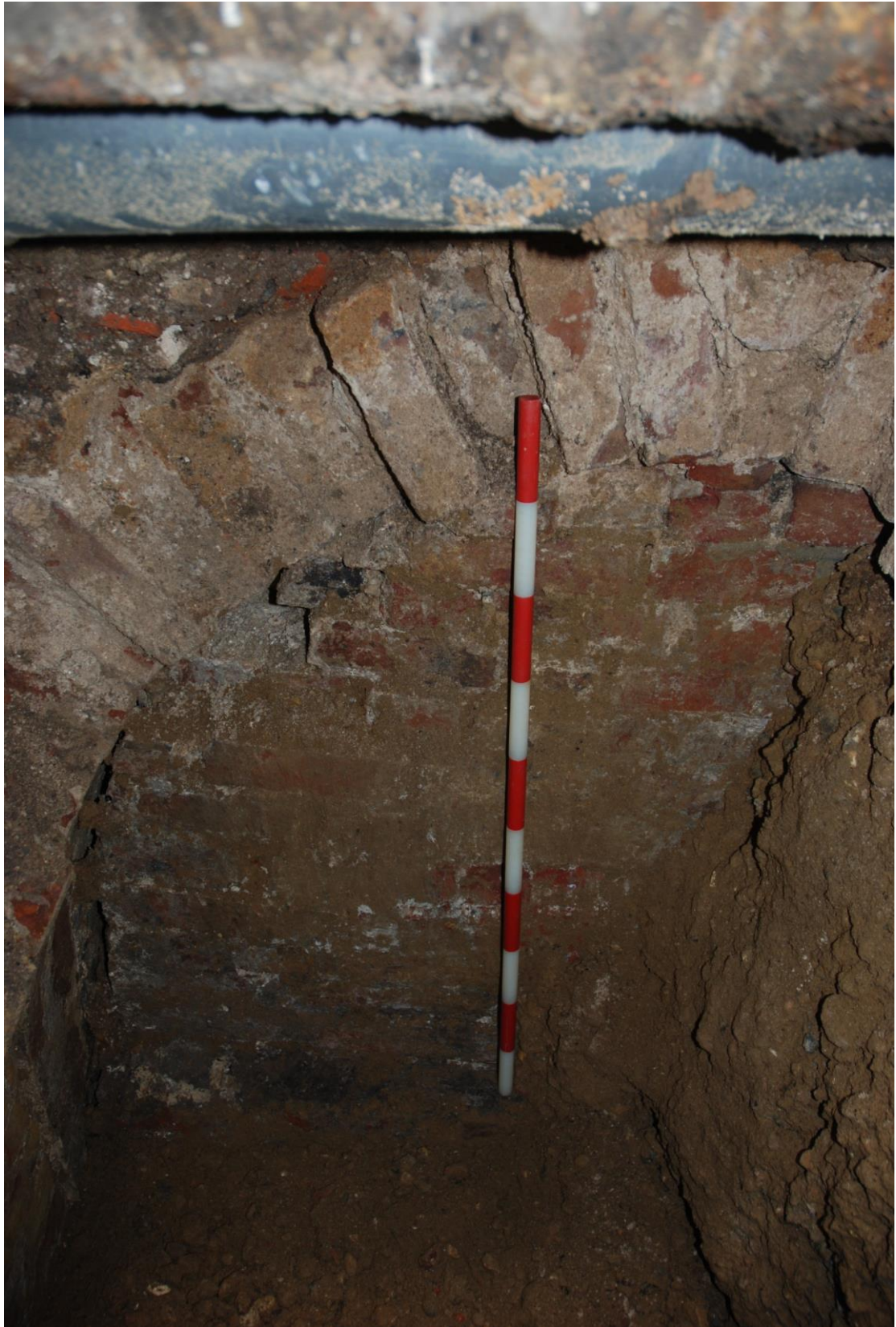
Fig.9: Blocked passageway facing ENE. A noticeable gap between the passageway wall and the brickwork blocking any access is clearly visible (1m scale)
