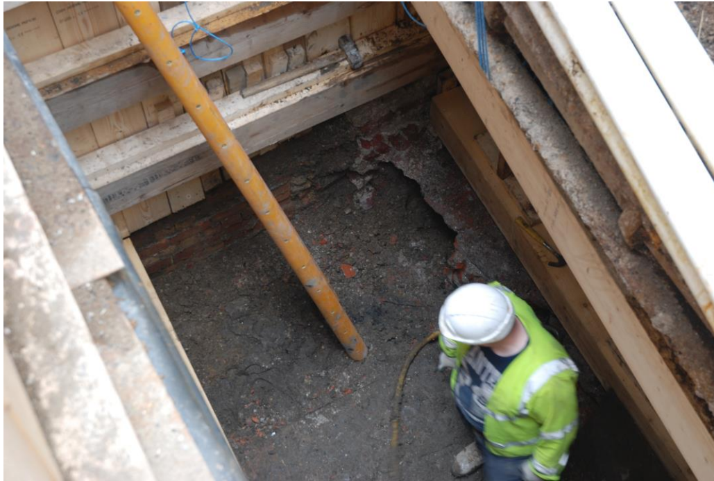
Fig.13: Pit 3 facing S showing the brick passageway and possible culvert in SW section. Approximate depth is 4.2m at base
