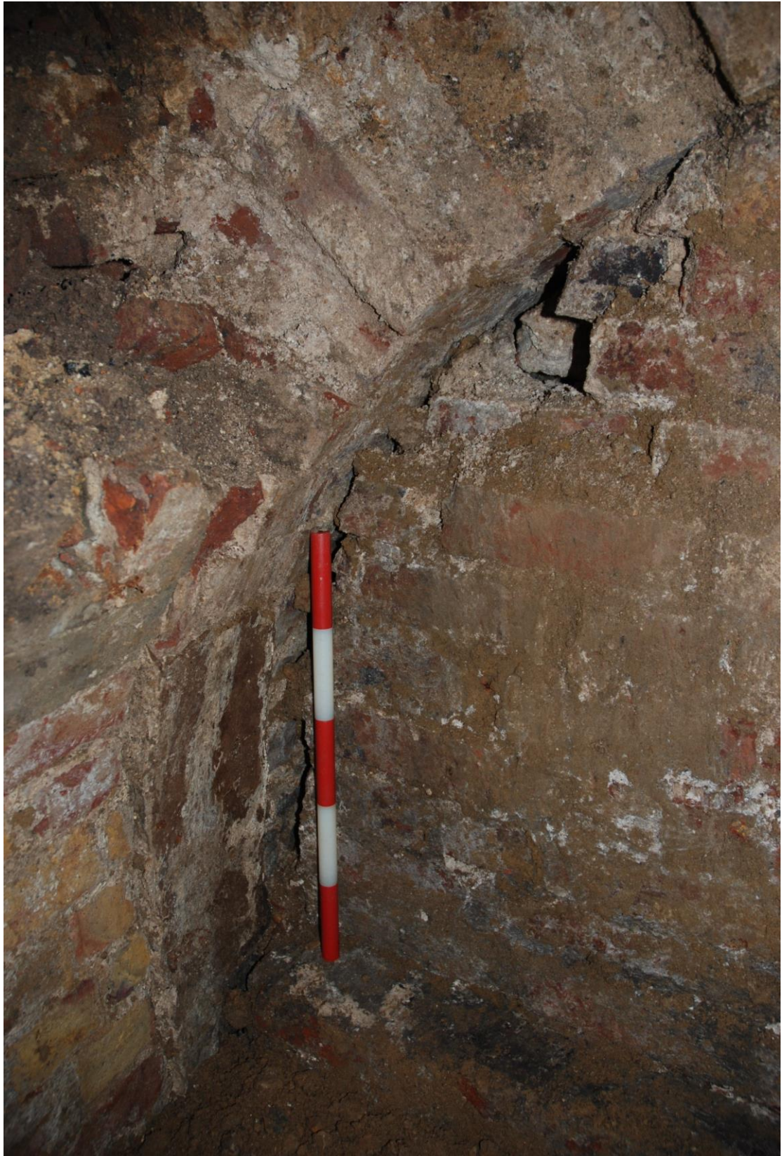
Fig.10: Blocked passageway facing NE. The crudely built wall blocking access is visible, as is the fact that the archway is constructed independently from the east and west section of wall, 'wedged' between the two (50cm scale)
