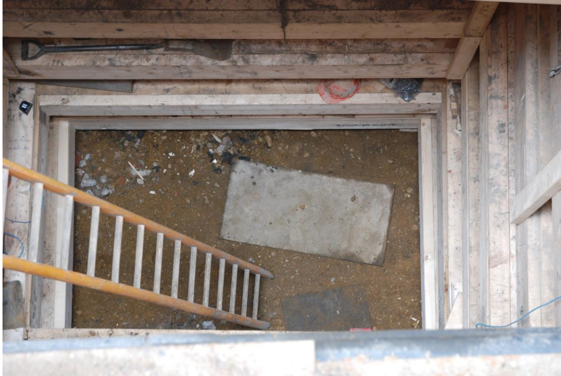
Fig.15: Base of pit 3 at c6.5m below ground level showing natural gravels and sands.
