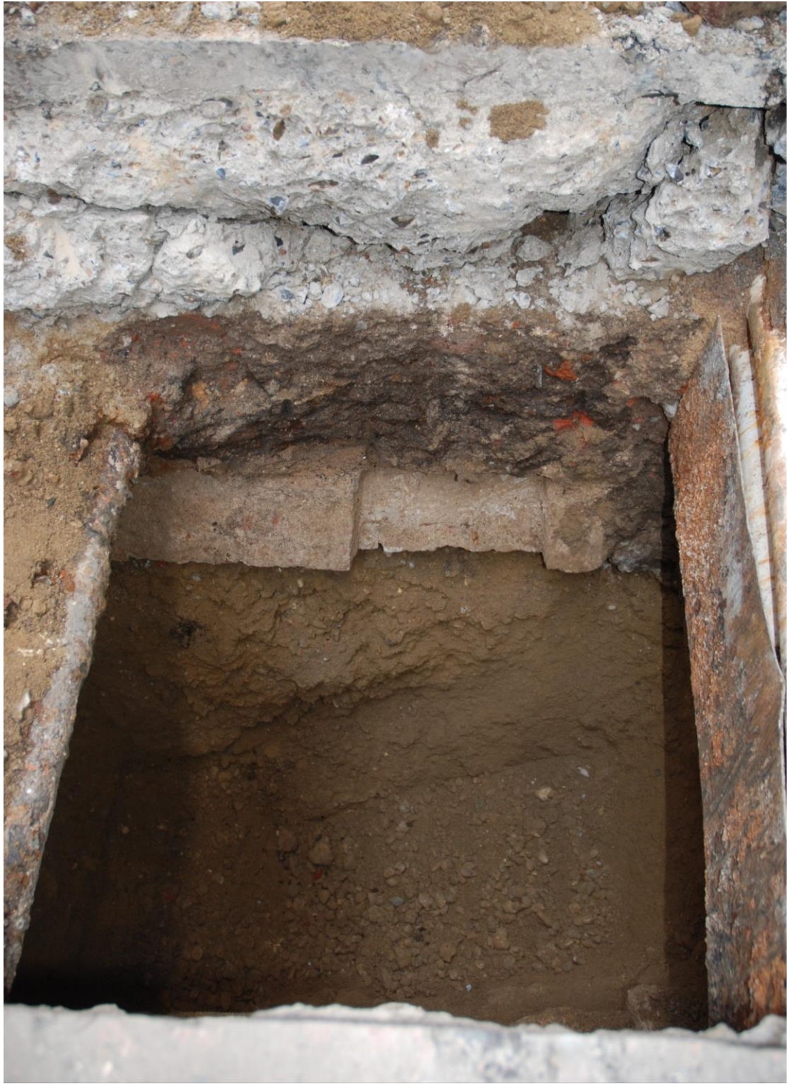
Fig.11: Sondage facing SSW showing the broken spring-work of the passageway arch below made ground and the existing road base
