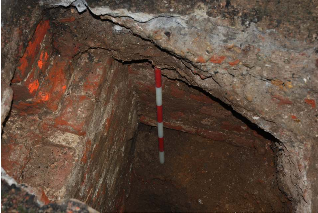
Fig.7: Walls within Trial pit 8. The wall to the left of frame is an earlier incarnation of the eastern garden wall, with the beginning of a doorjam just visible by the remnants of spray paint. The brick wall to the right abuts this at right angles and runs E-W across the present courtyard. (1m scale)
