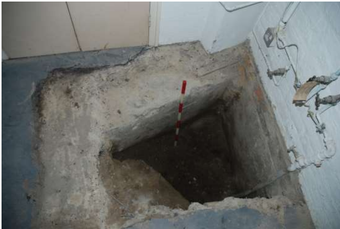
Fig.11: Photo of the trial pit from above, showing the concrete foundations of the walls and the brick and concrete dump in the north-western corner (front left of photo)
