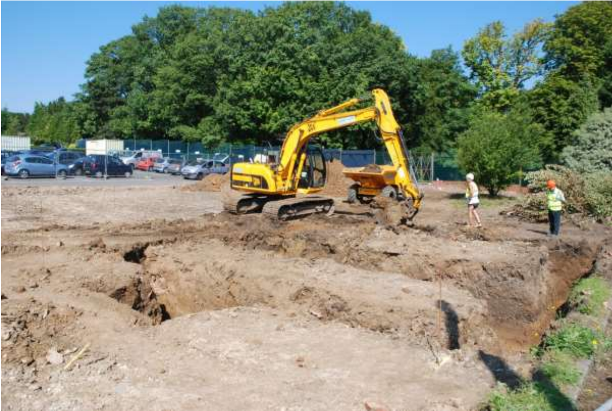
Fig.8: Photo of the excavation of the foundations of the main building, looking north-west
