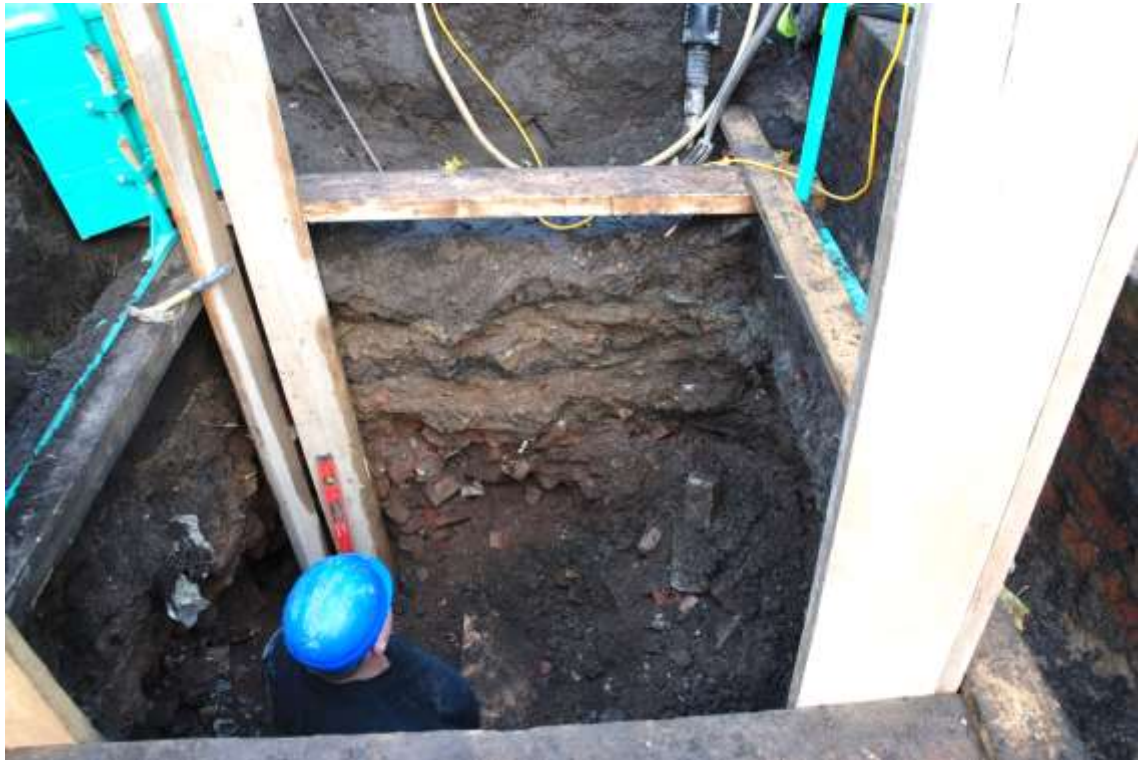
Fig.21: Pit 3 at a depth of approximately 1.8m showing the layers of made ground. Facing NE
