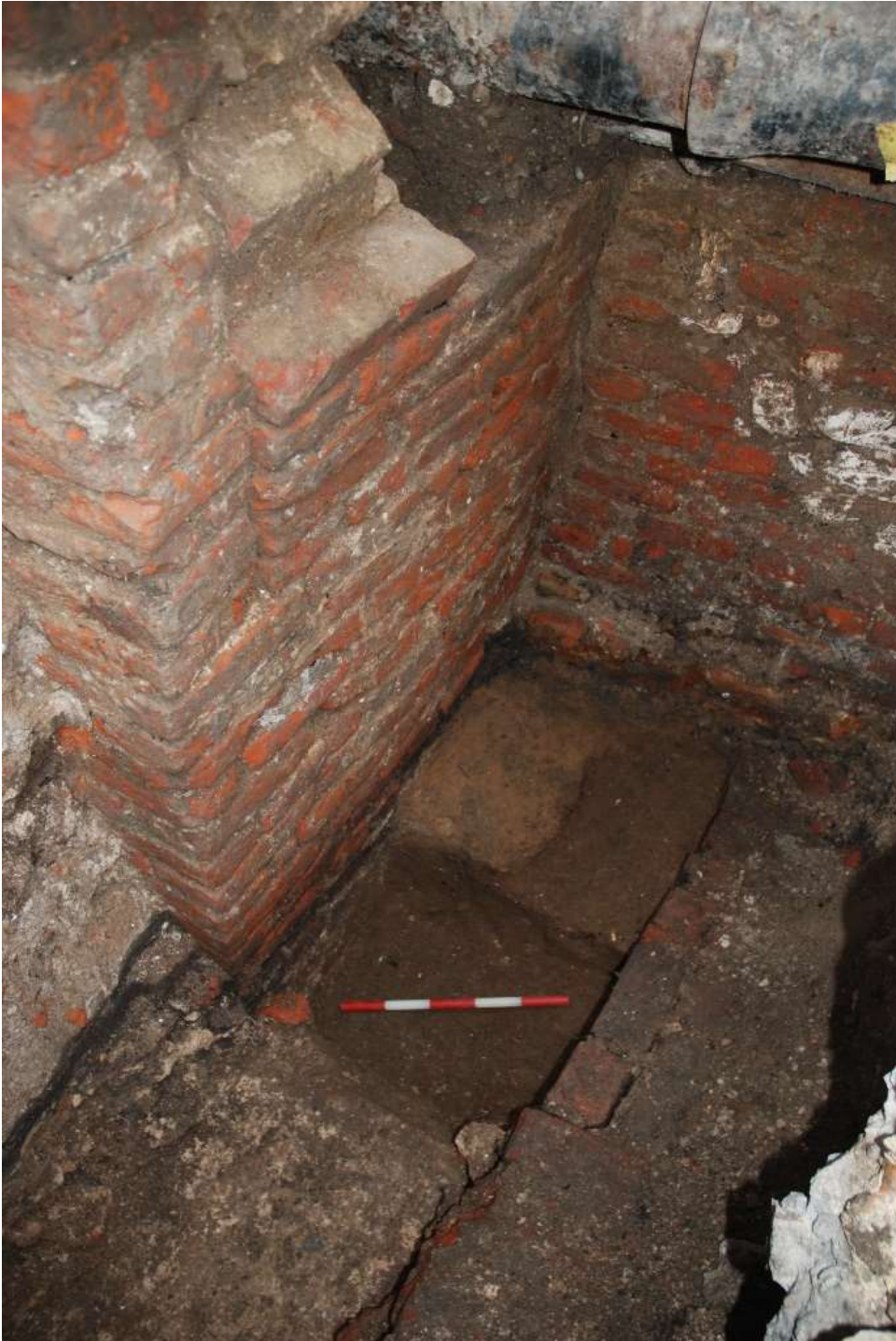
Fig.12: Coal Cellar facing SW, post removal of brick floor. The 50cm scale rests within the robber cut [14]. Also on top of, and, adjacent to Roman deposit, (16). The remnants of the City wall, [15], are visible as a block of buff-coloured mortared masonry in the bottom left of frame.
