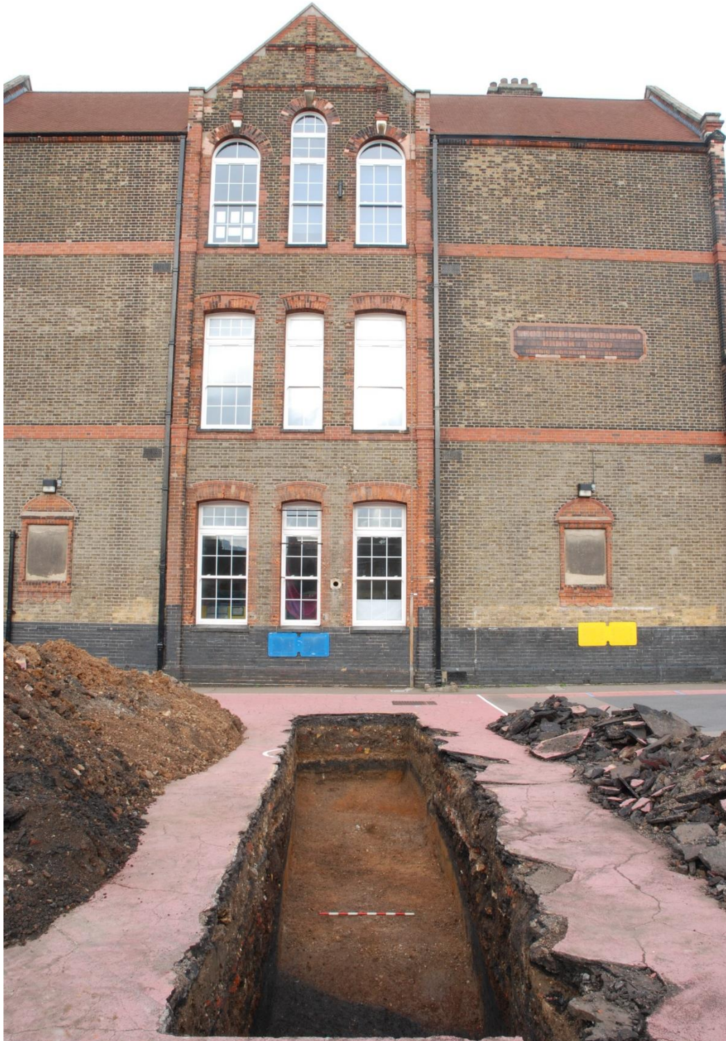
Fig 7: General view of the evaluation trench looking northeast, with the main School building in the background
