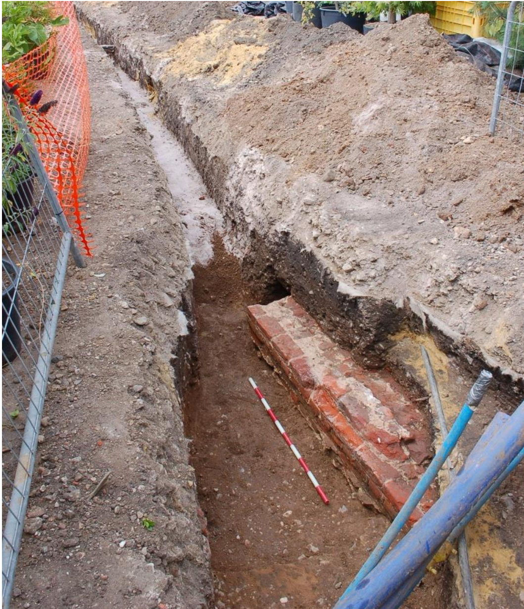
Fig.5: Truncated wall in Trench 2 of the 2010 watching brief, facing W (towards the NW end of the proposed glasshouse). It is possible the wall may survive at a greater depth elsewhere within the glasshouse footprint, but is not visible here.
