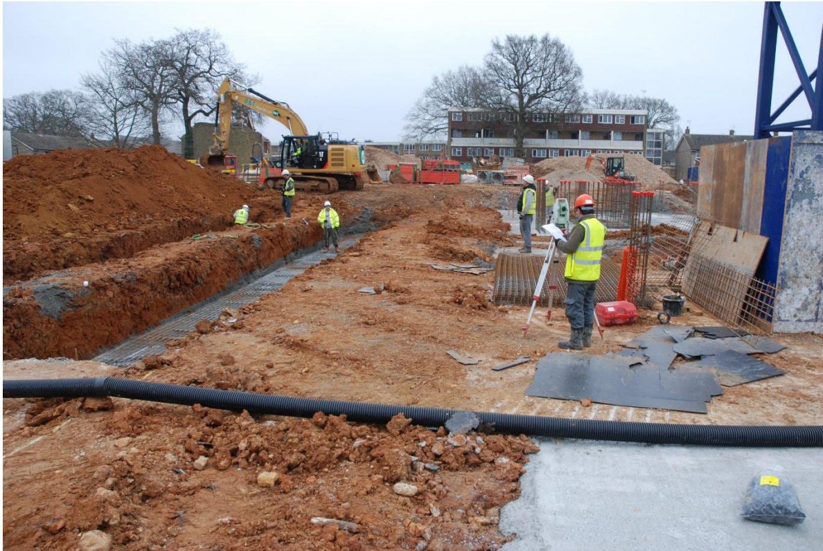
Fig. 20: General view looking east across the site towards Area 3 (located just to the right of the tracked machine)
