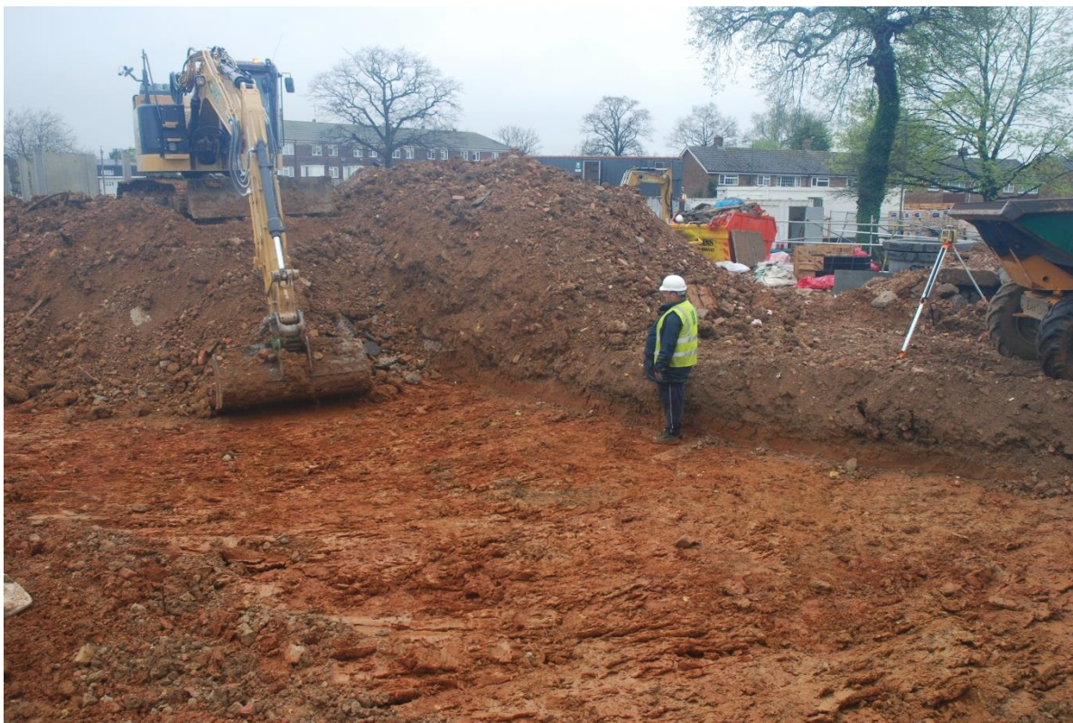
Fig. 23: A further view of the northern part of Area 4 during machine reduction, looking northwest towards Wallis Avenue
