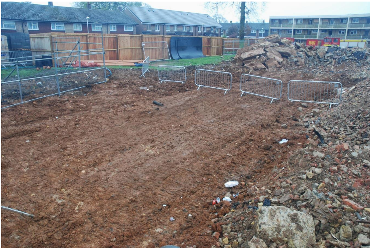
Fig. 28: The eastern part of Area 6, looking northeast towards the boundary with Wallis Oak Avenue. Recently removed demolition concrete footings, etc., can be seen in the background
