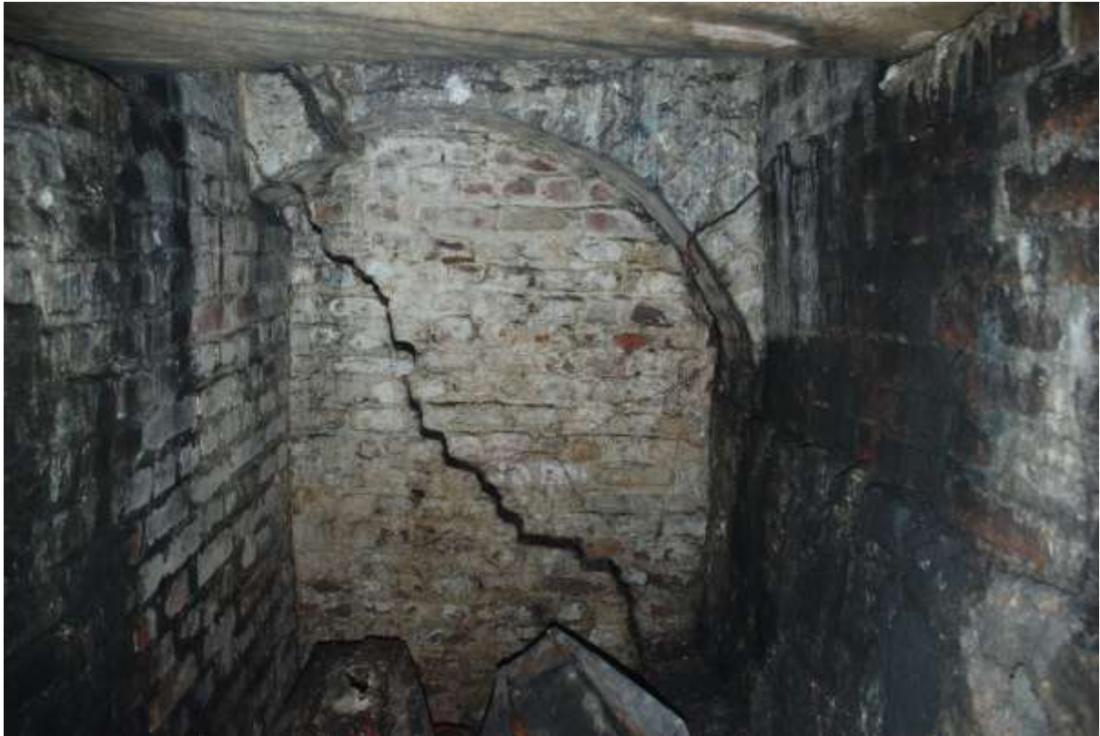
Fig.15: The east end of v/004, showing the blocked up entrance to v/003, including the truncated arch. This entrance would once have had steps leading up to ground level
