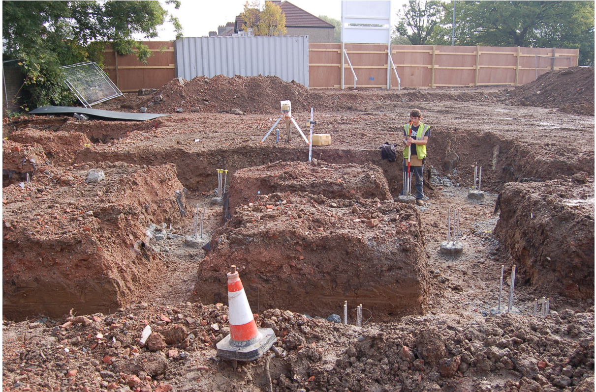
Fig 13. View of the first phase of strip footing works, looking towards Church Street at the east of the site
