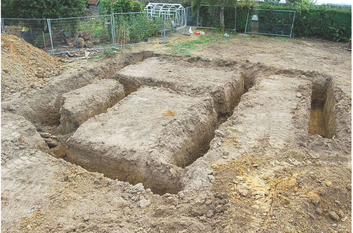
Fig 11. View of the c 2m deep excavated footings for Plot 1, looking south
