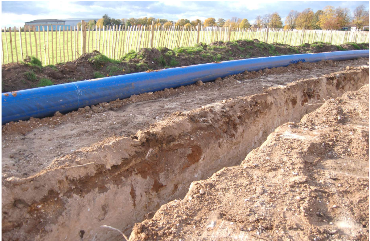
Fig 8. The pipe trench and buried trackway, in the same area as above but facing west towards Purley Way
