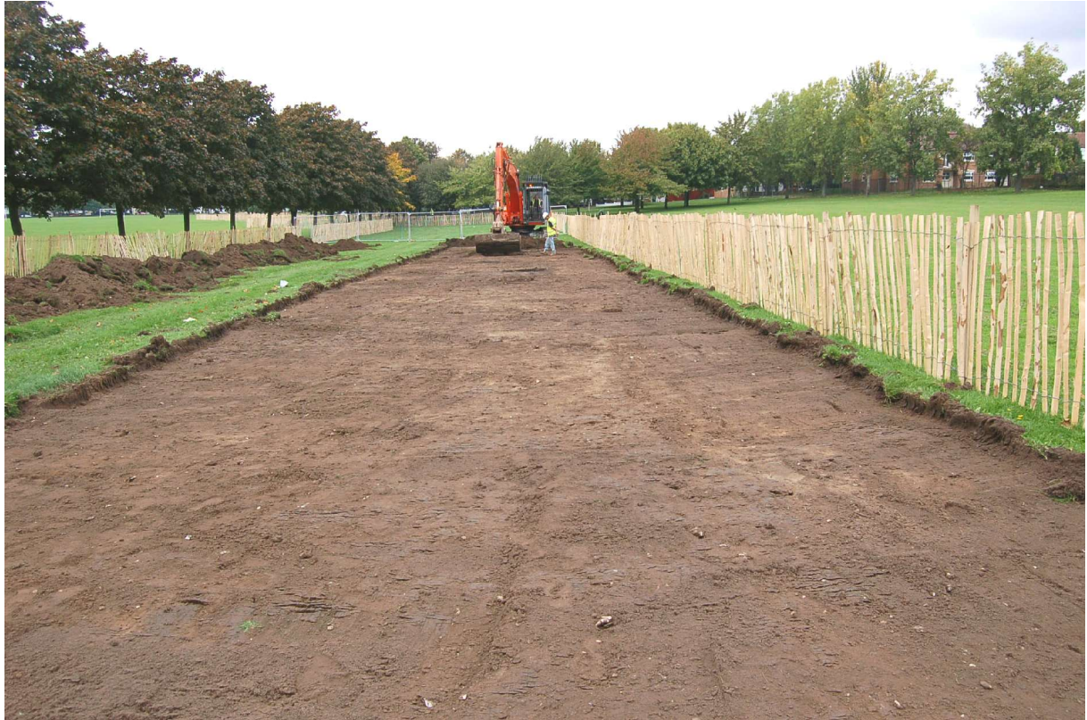
Fig 5. Photograph showing the machine topsoil stripping that took place during the first phase of works on the site, facing north towards Waddon Way
