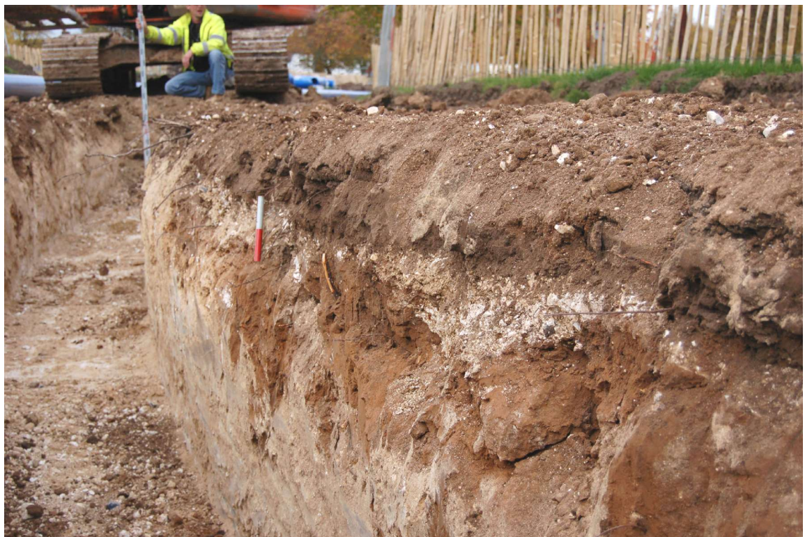
Fig 11. Further photograph of the above area looking north along the line of the pipe trench, with the trackway visible as a thin layer in section at the level of the 0.2m scale
