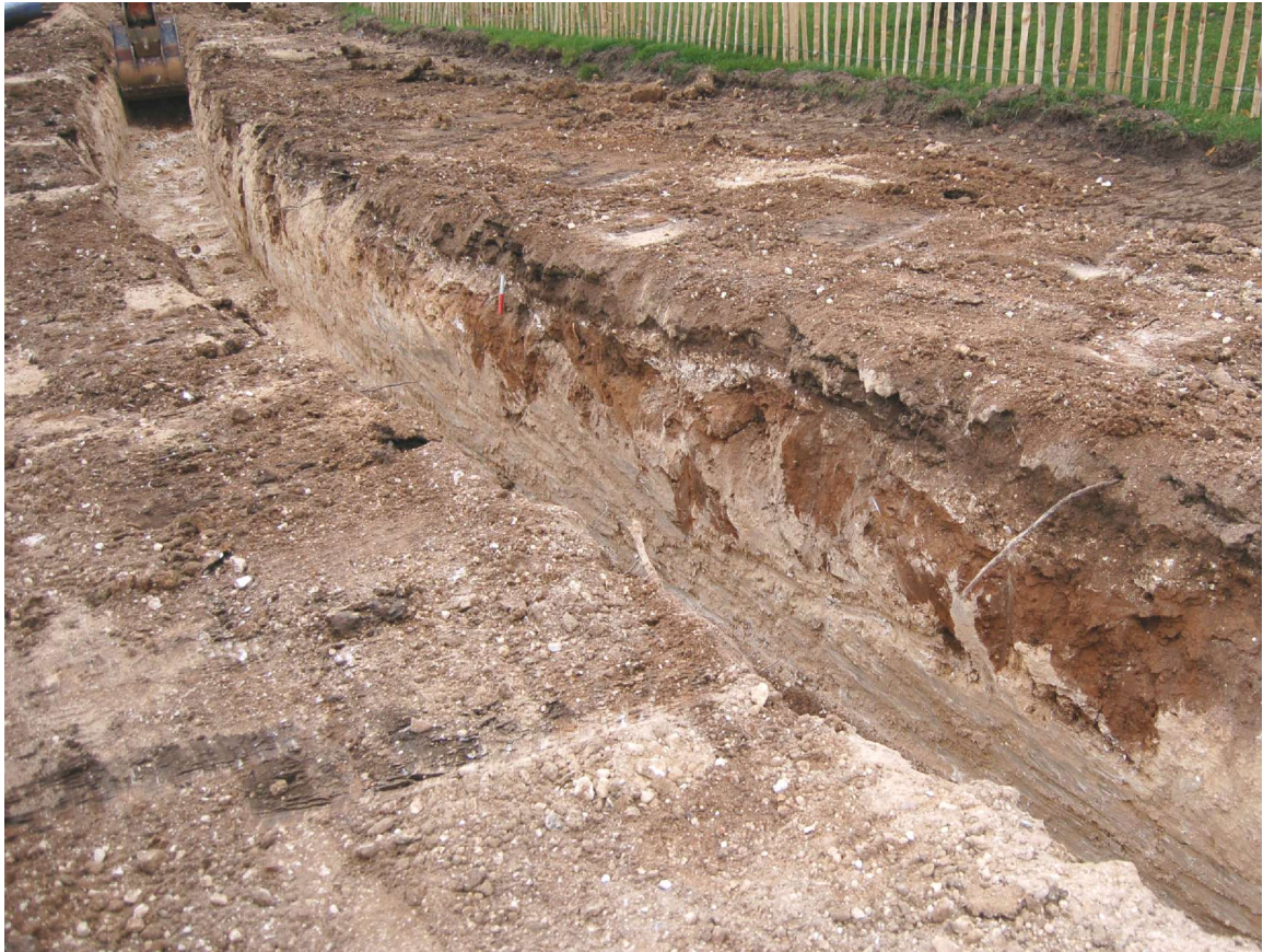
Fig 10. Detailed photograph of the area of pipe trench shown in Figure 7, with the trackway visible as a thin chalk and gravel layer
