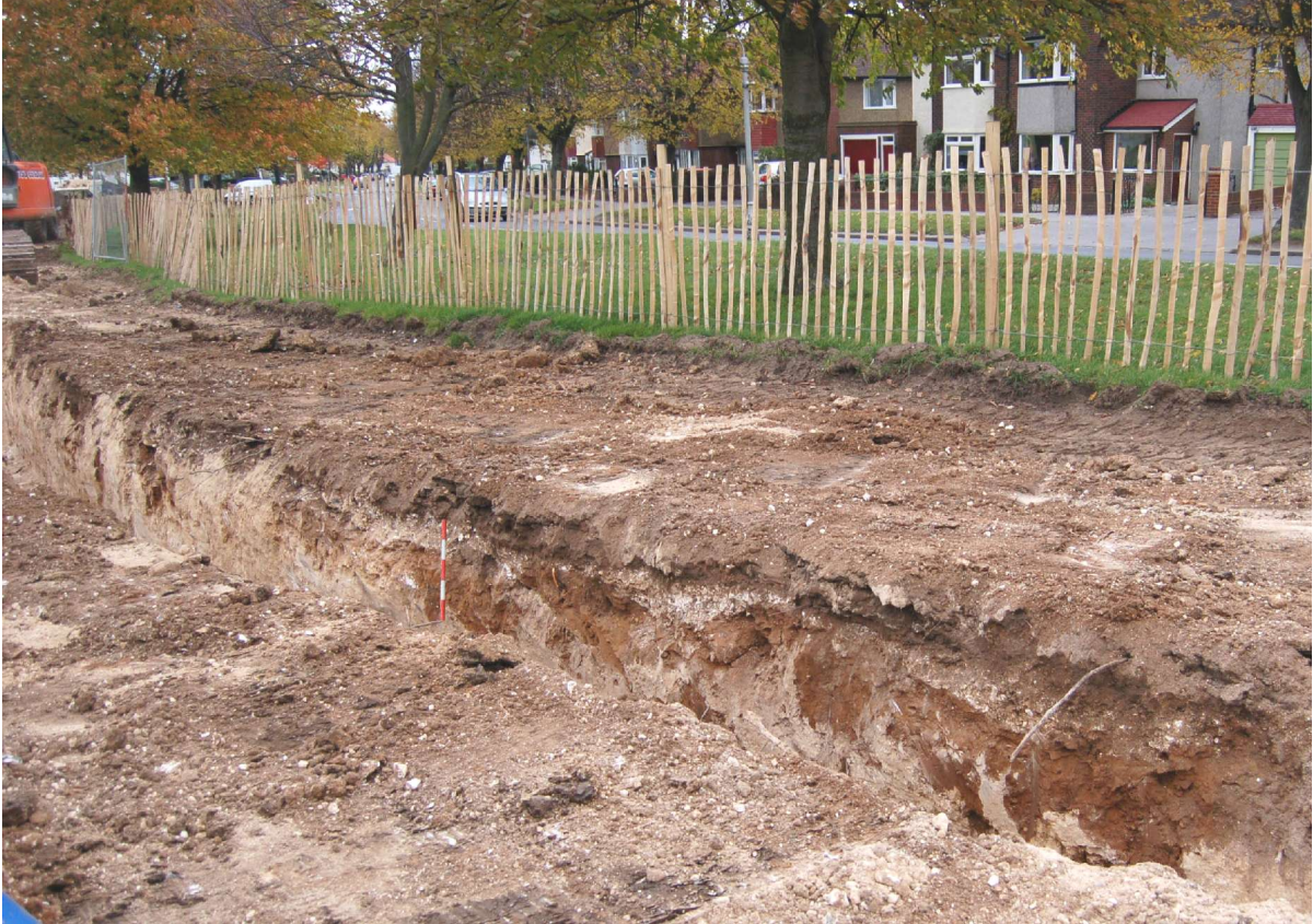
Fig 7. Photograph facing north towards Waddon Way, showing the pipe trench with the buried trackway visible as a relatively thin chalk layer near the top of the 0.5m scale. See also Fig. 9
