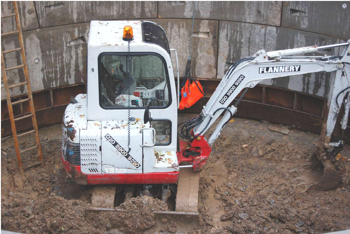
Figs 6 & 7. Facing south-west. Further work on the chamber has been carried out and the base of the excavated area is now free of water. The clay and alluvial deposits have been clearly revealed.
