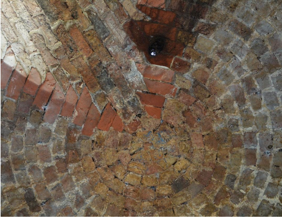
Fig.14: The centre of the dome visible from below (a hole in the structure at the top of the frame representing later damage)
