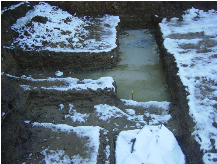
Fig 31 Periods of very poor weather and flooding of the site in early April 2006 (see front cover), looking south along the partially reduced cut for Groundbeam 2.
