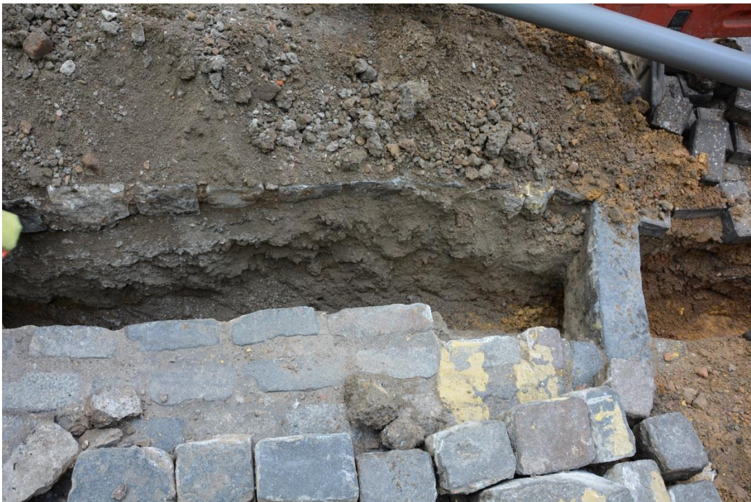
Figure 6: Rubble and road make up beneath cobbled surface. Facing N. No scale.
