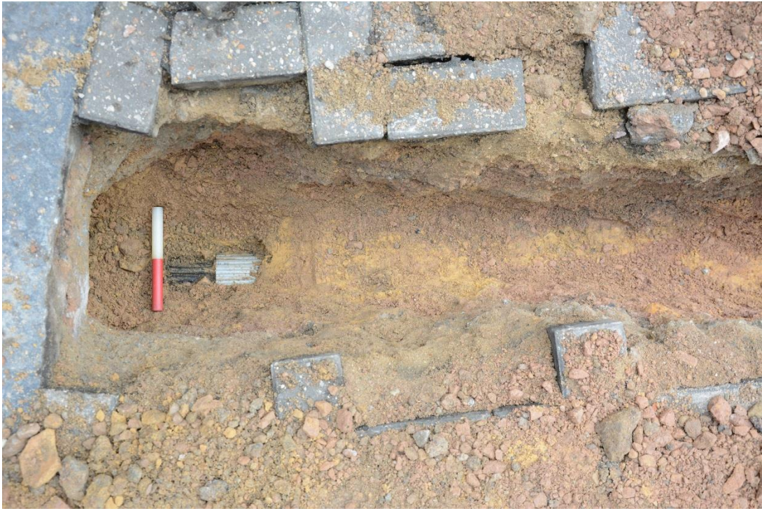
Figure 5: Exposed services below the level of excavation, east of Spital Yard. Scale 0.2m.
